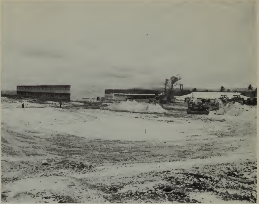
The foundation is laid for a new $245,865 classroom building at the College of Guam. Another classroom building, library, and cafeteria-recreation hall are in the background.
