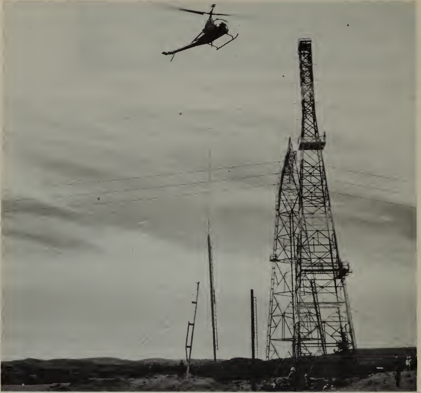
A helicopter is used to carry a steel tower leg across the Columbia River to an island for the Big Eddy-Chenoweth transmission line near The Dalles, Oreg.
