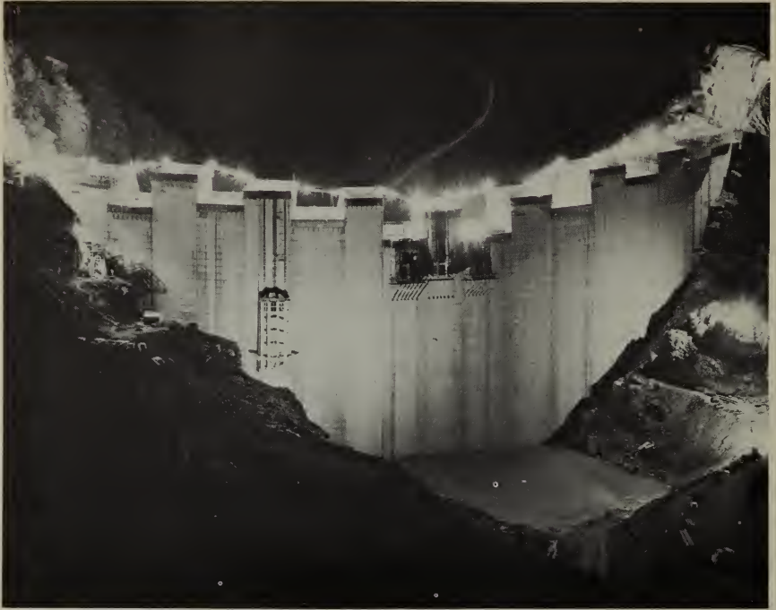
Night view of Flaming Gorge Dam on Green River in Utah as construction passes the three-quarter mark.
