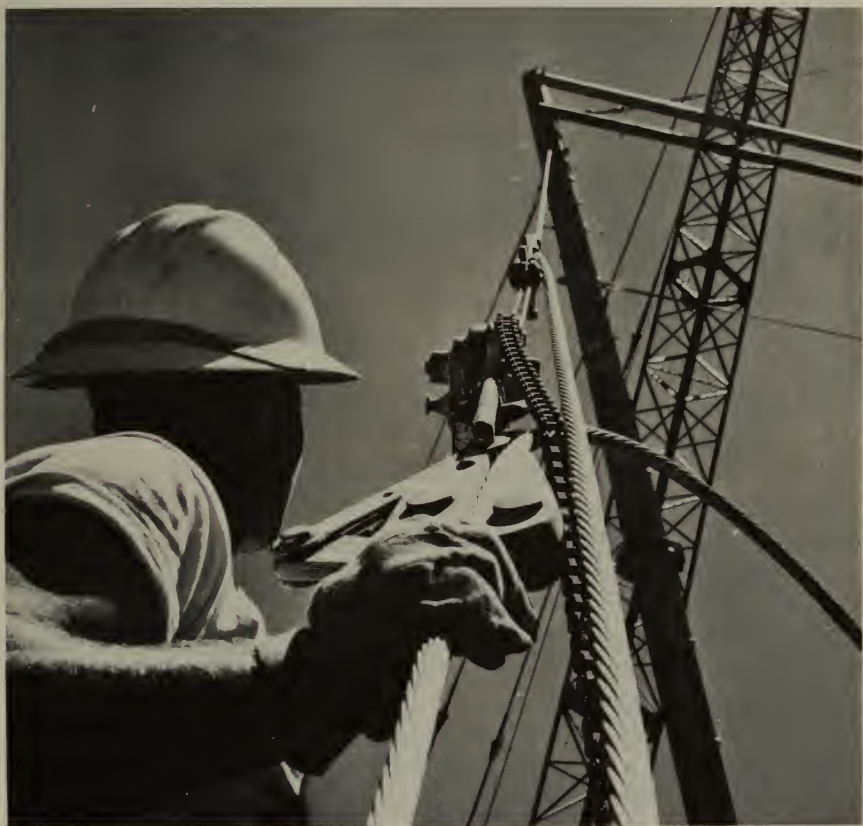
A lineman tightens the guys on a new type of steel H-frame transmission structure carrying power from the Cougar Dam in the Willamette Basin to lower Willamette Valley load centers.
