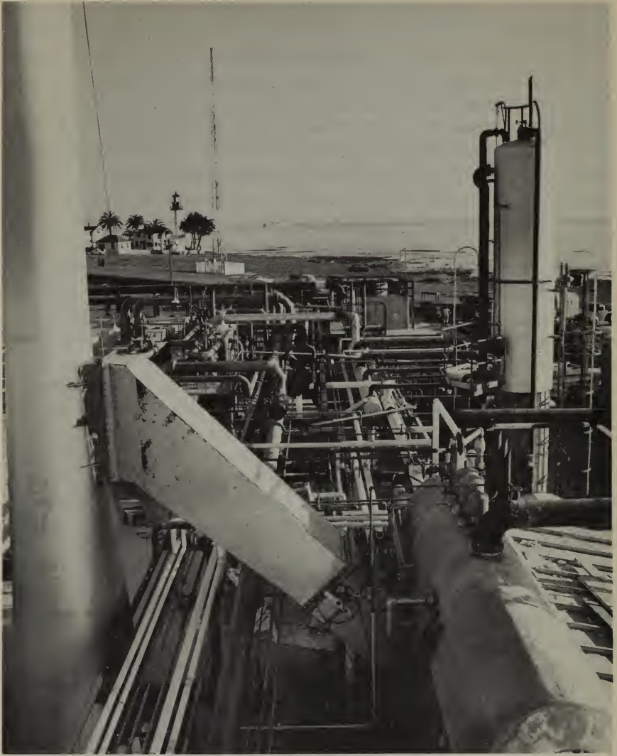
New Point Loma sea-water desalting plant near San Diego, Calif., points out multiple piping systems through which the flash evaporator process functions.
