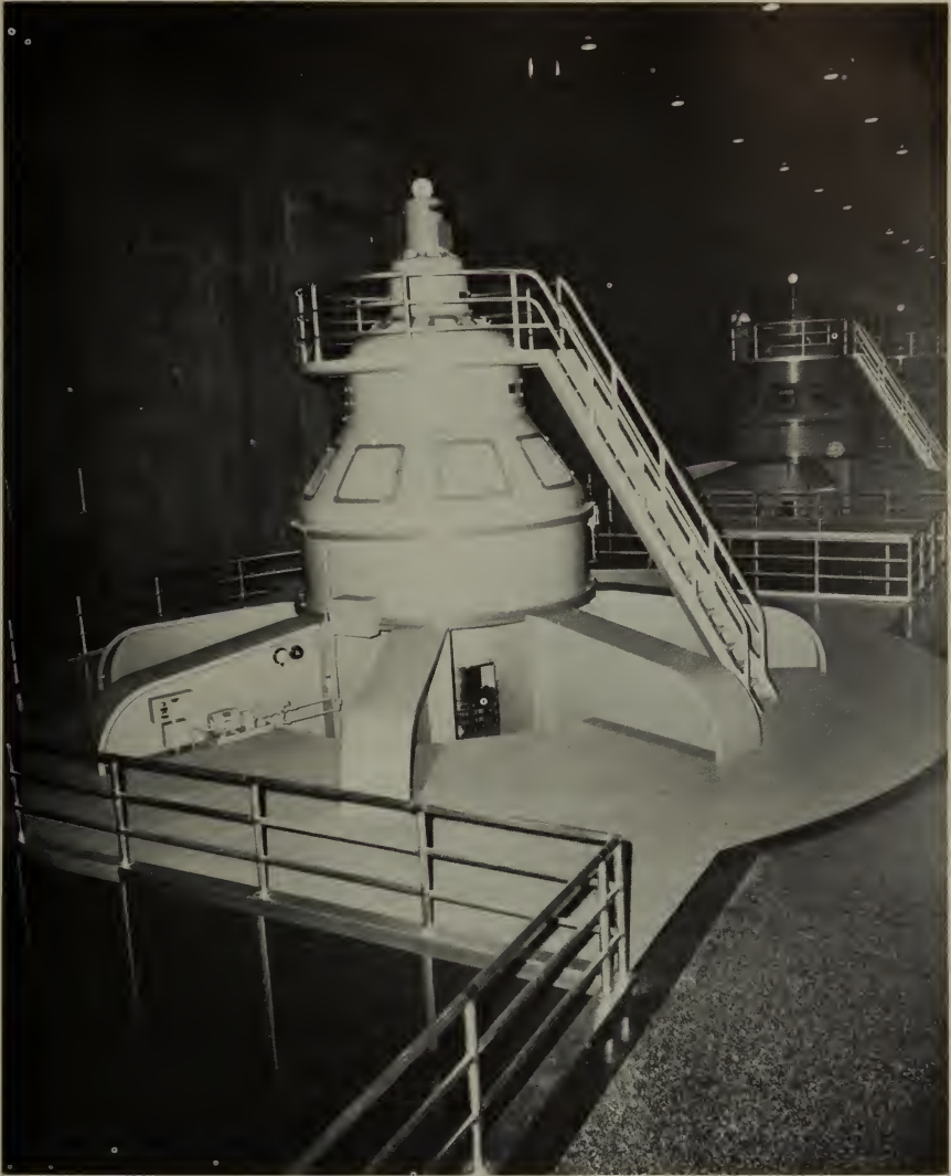
Installation of Hoover powerplant's final generating unit brings the Boulder Canyon project to its full capacity of 1,344,800 kilowatts.
