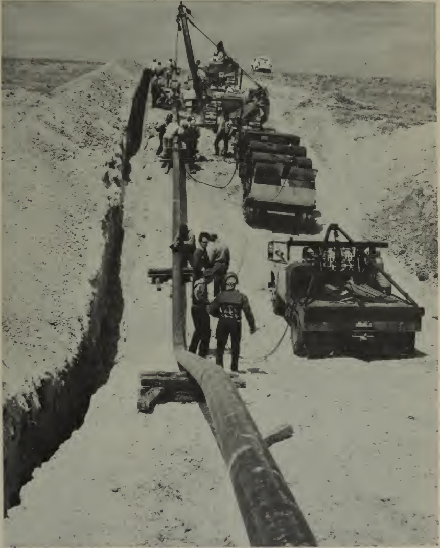
Bureau of Mines has completed 430-mile pipeline system to carry newly saved helium to underground storage in Texas.
