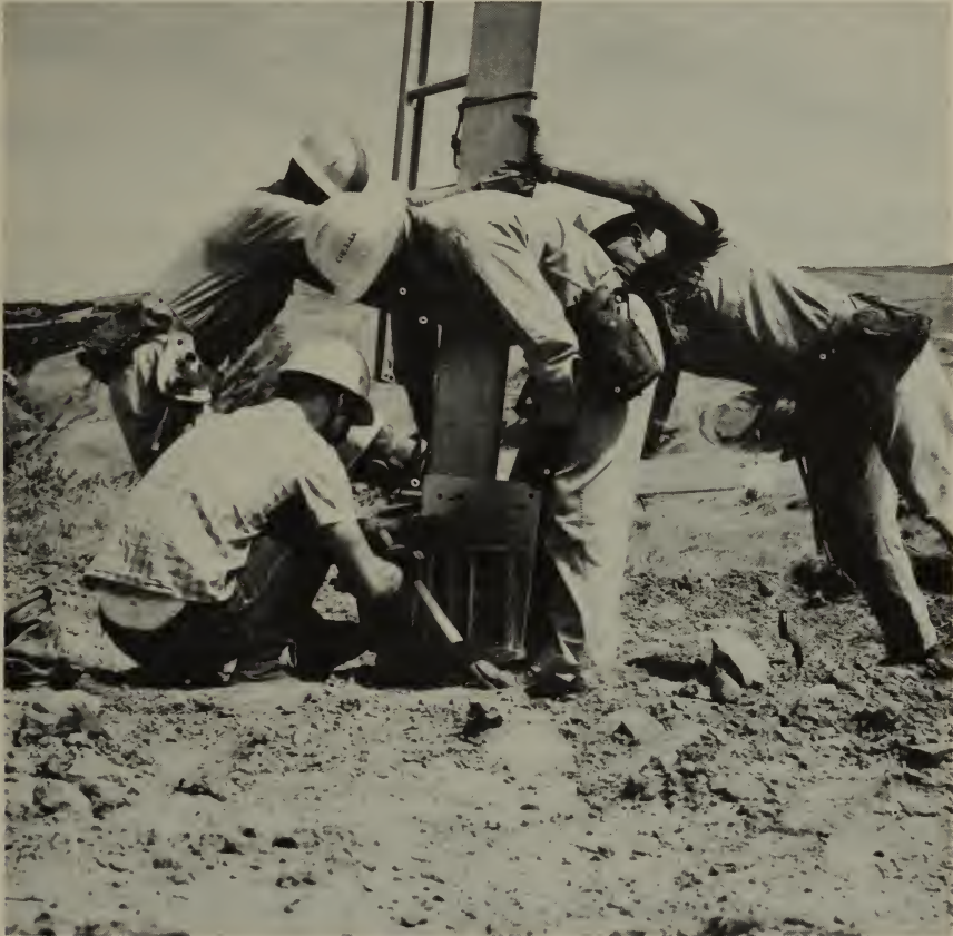
As the helicopter holds the tower leg vertically, workers bolt it in place on the anchor strut.
