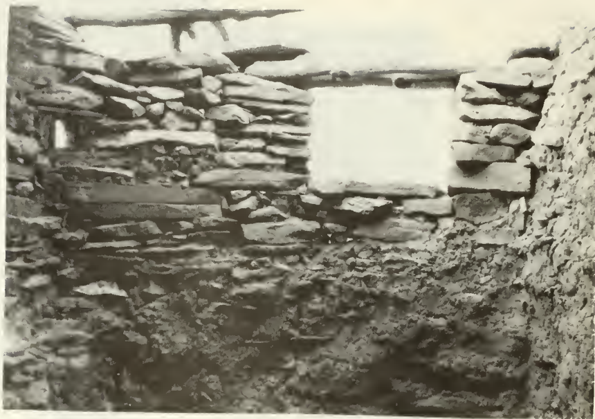
"Before" shot of the interior south wall of room 1. Note the missing section of roof and lack of mortar on the stones around the window. (looking south)
