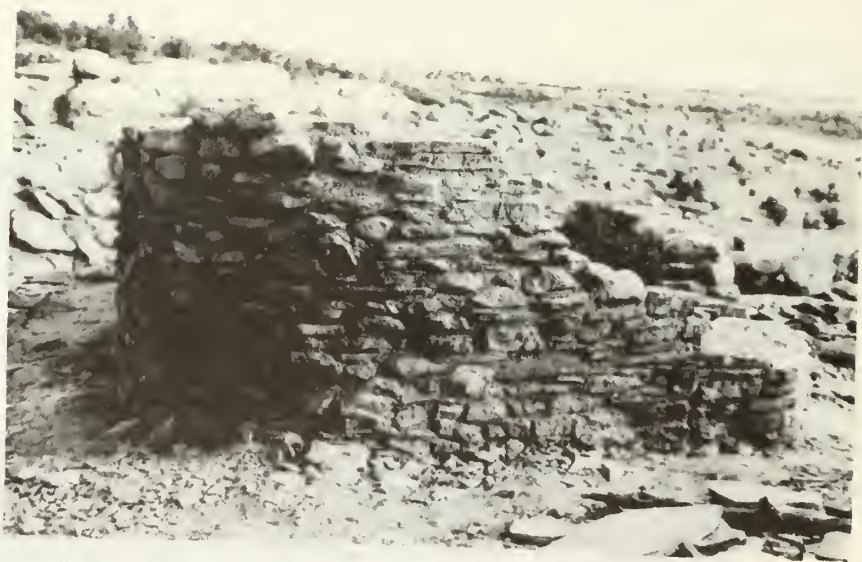
"After" stabilization; the walls have been reconstructed to their former height. (looking north)
