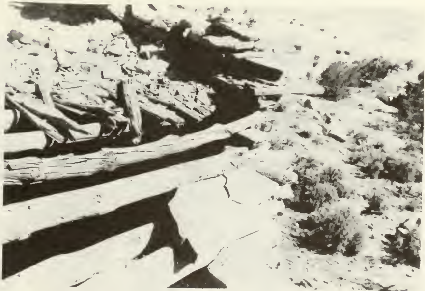
The 2 vigas used to fill the section of missing roof during the stabilization. (looking east)
