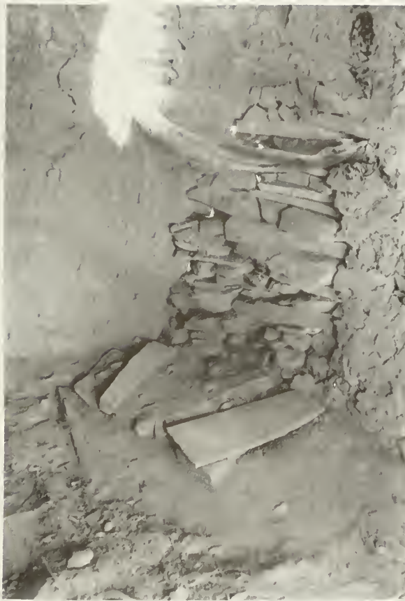
"Before" shot of "hooded" fireplace in northeast corner of room 1. The juniper bough was the base of the "hood". Water coming through chimney has caused wall deterioration. (looking north)
