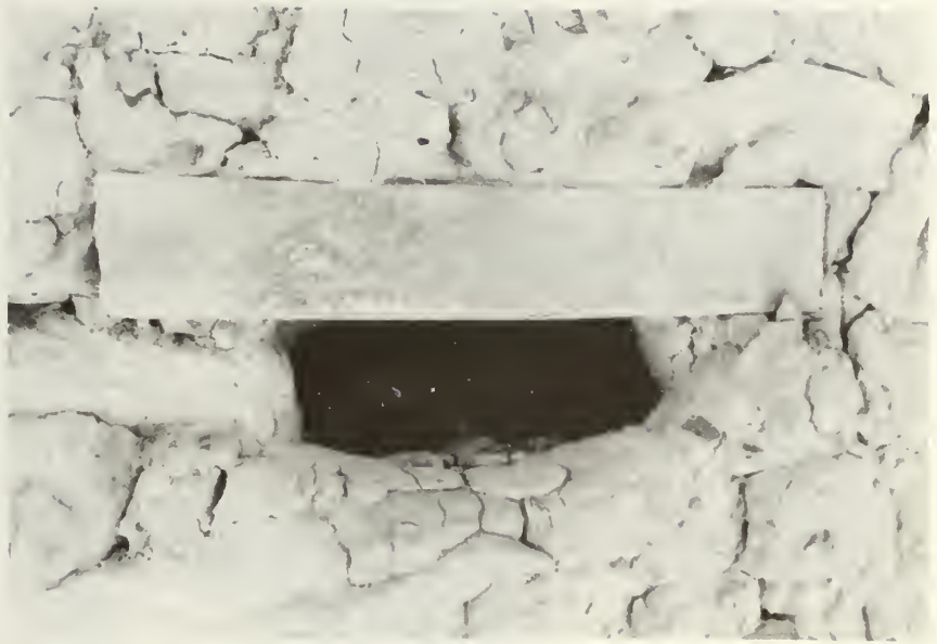
Small niche in east wall of room 2, located above and south of the doorway. (looking east)
