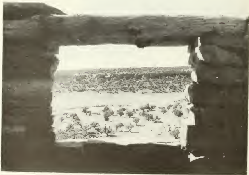
"Before" shot of the large window in the south wall of room 1. The window is the product of a recent repair job as indicated by size (too large), kind of lintels (juniper vigas) and color of clay (gray). (looking south)
