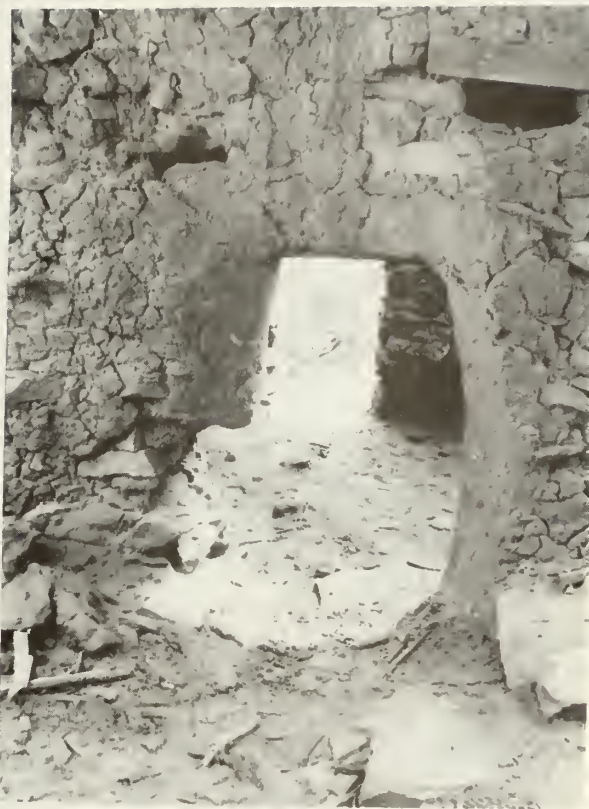
"Before" shot of the doorway connecting rooms 1 and 2. Note how the side of the door is eroding out. (looking east from room 2)
