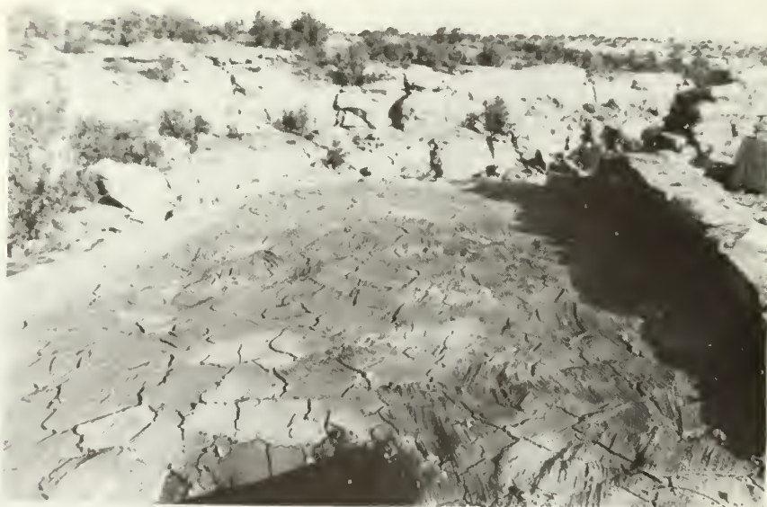
"After" stabilization; the reconstructed roof of room 2, and the rebuilt section of parapet wall. (looking north)
