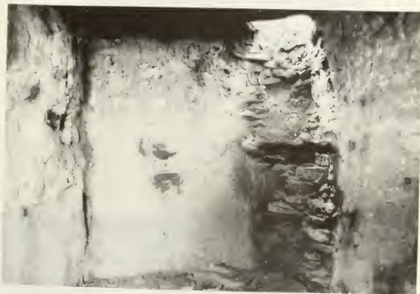
"After" stabilization; the hooded fireplace. Note the dark areas of grout on the interior walls. (looking north)
