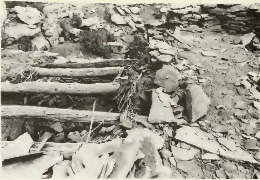
"Before" photo showing the collapsed parapet wall on room 1 and the deteriorated roof of room 2. (looking north)
