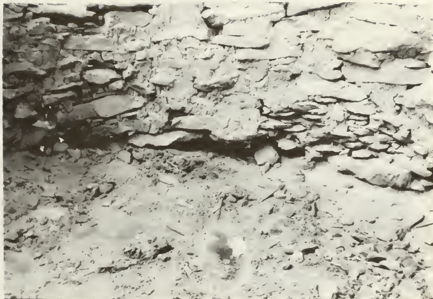
"Before" shot of west wall of room 3 showing base of wall undermined by erosion. (looking west)
