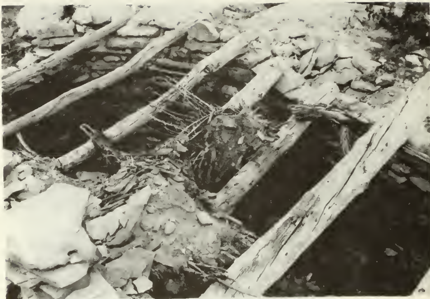
"Before" photo showing the original appearance of the roof on room 2. (looking south-west)
