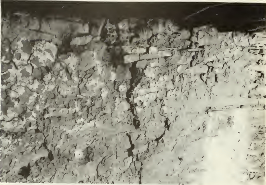
"Before" shot of a large crack which formed in the east wall of room 1 upon the removal of the stone in the hearth area during the stabilization. (locking cast)
