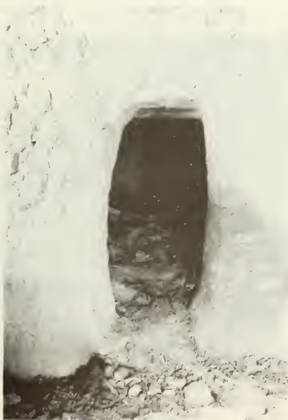
"After" stabilization; the eroded area has been patched. (looking west from room 1)
