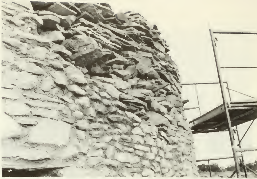
Grouting the exterior east wall of room 1, showing the contrast between the grouted and original wall surface. Note the ends of the roof beams protruding from the wall. (looking northwest)
