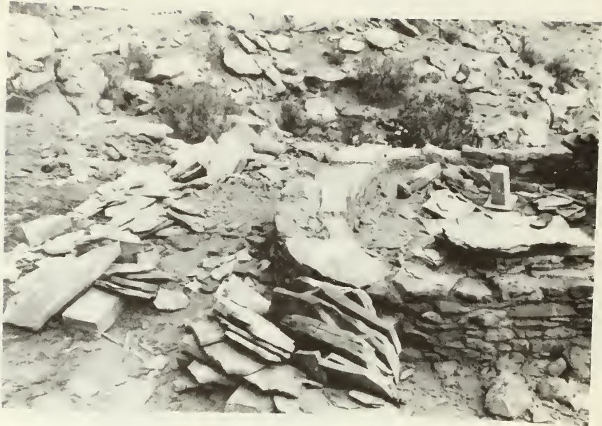
Stabilizing the walls of room 4. The south and west walls were taken down in order to correct their outward leaning. Note the cement core used in the base of these walls. (looking north)
