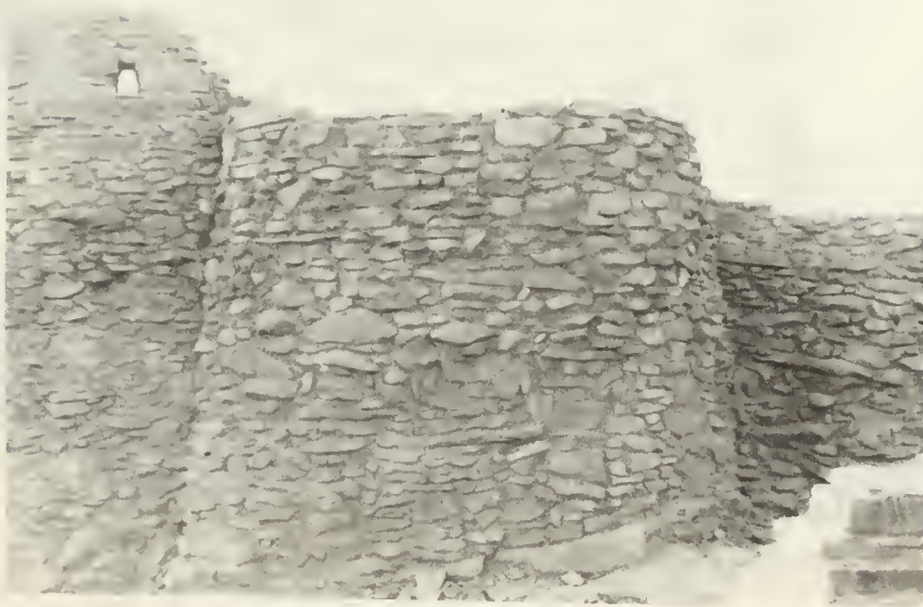
"After" stabilization; the north wall of room 2. The wall has been built up to accommodate the reconstructed roof. (looking south)
