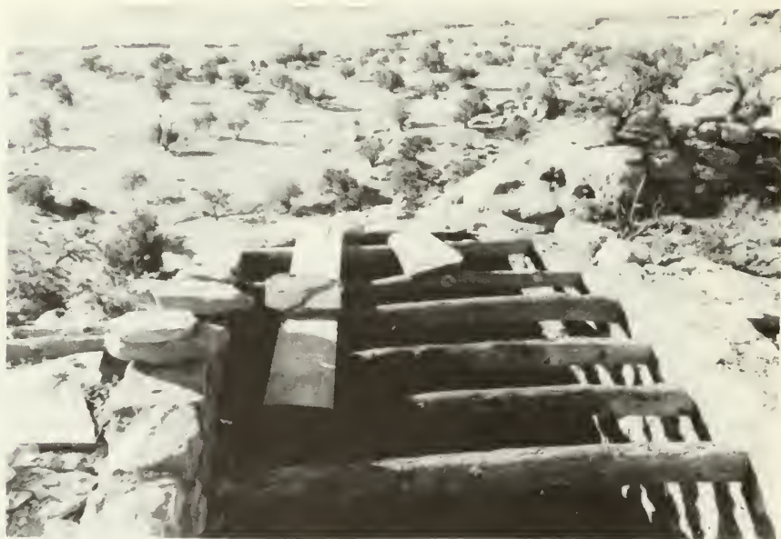
Clearing away the original roofing and building up the walls. (looking south)
