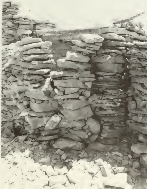
"Before" shot of the poor construction in corner joint of room 2. (looking southeast)
