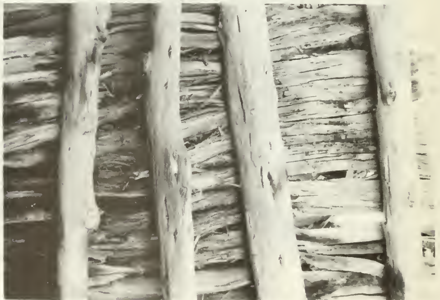
A section of roof on room 1 which shows a former repair job. The repaired section lacks smoke stain and contains branches mixed with the split wood latillas. Vigas are of juniper, Douglas fir, and pinyon.
