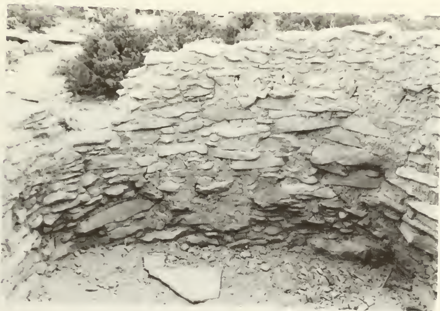
"After" stabilization. Note the eroded window in the left of the photograph. This window may have been the original entrance. (looking west)
