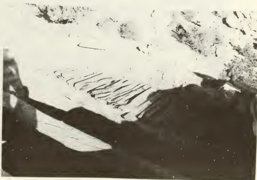
Adding the split wood latillas transverse to the vigas during the reconstruction of the roof on room 2. (looking north)
