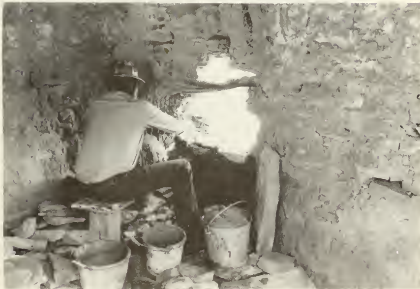
Raymond Torrivio rebuilding wall in area of the hooded fireplace. Removal of the stone caused the wall to settle causing a large crack to form in the east wall of the room. (looking north)
