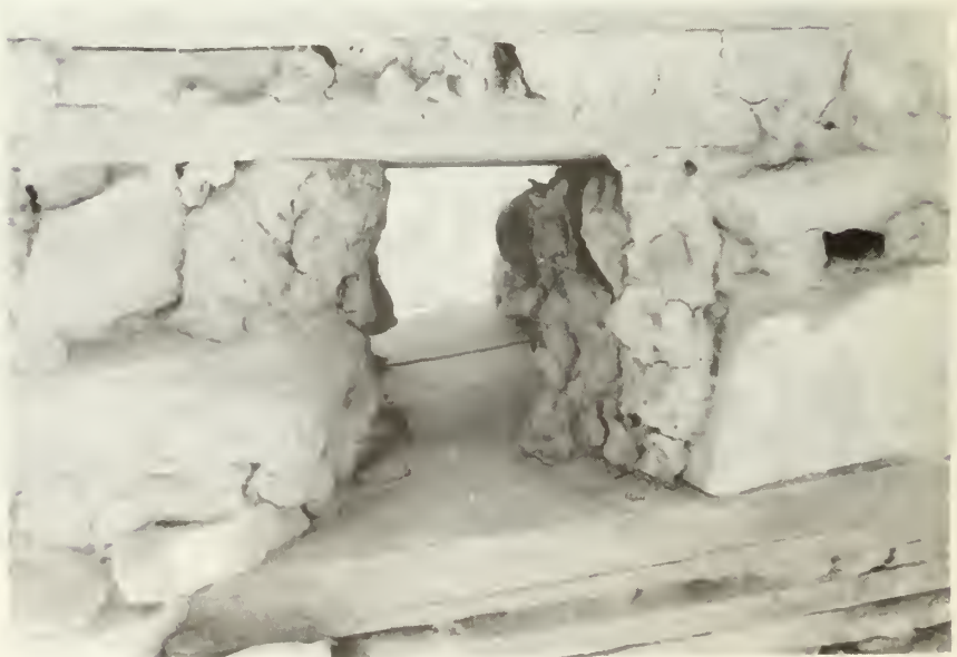
Loop-hole style window in west wall of room 2. Window lines up with winter solstice sunset. (looking west)
