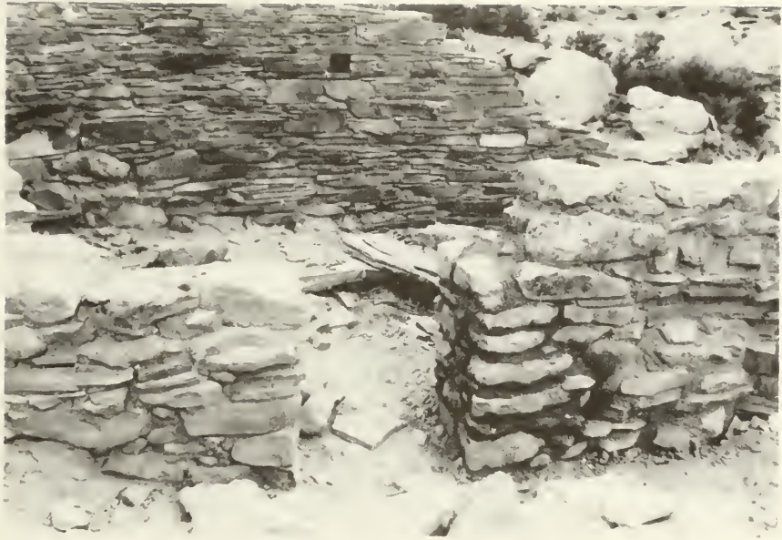
"After" stabilization; the reconstructed side entrance to room 4. The doorway was originally 18 inches wide. The first reconstruction put the stabilized width at 24 inches, necessitating the door be taken down and reconstructed again to the original 18 inch width. (looking west)
