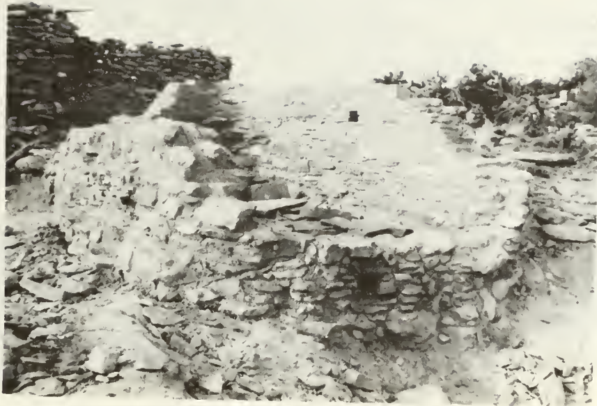
"After" stabilization. Note the drain in the foreground wall and the loophole in the west wall. (looking south)
