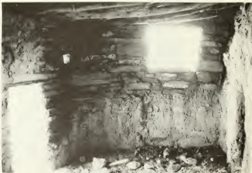
"After" stabilization; the stones have been grouted and the roof reconstructed. (looking south)
