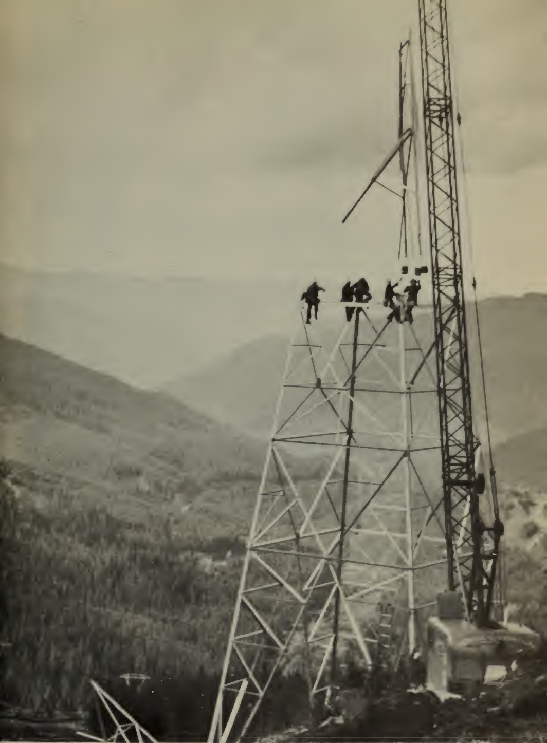
A construction crew, with the aid of a giant crane, erects a single circuit steel tower for Bonneville Power Administration's Tacoma-Grand Coulee 287,000-volt transmission line in the rugged Stampede Pass section of the Cascade range.
