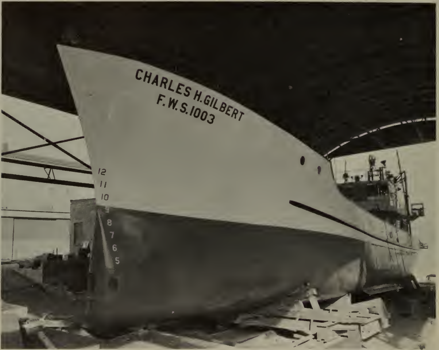
Construction of the underwater observation chamber on the bow of the "Charles H. Gilbert".
