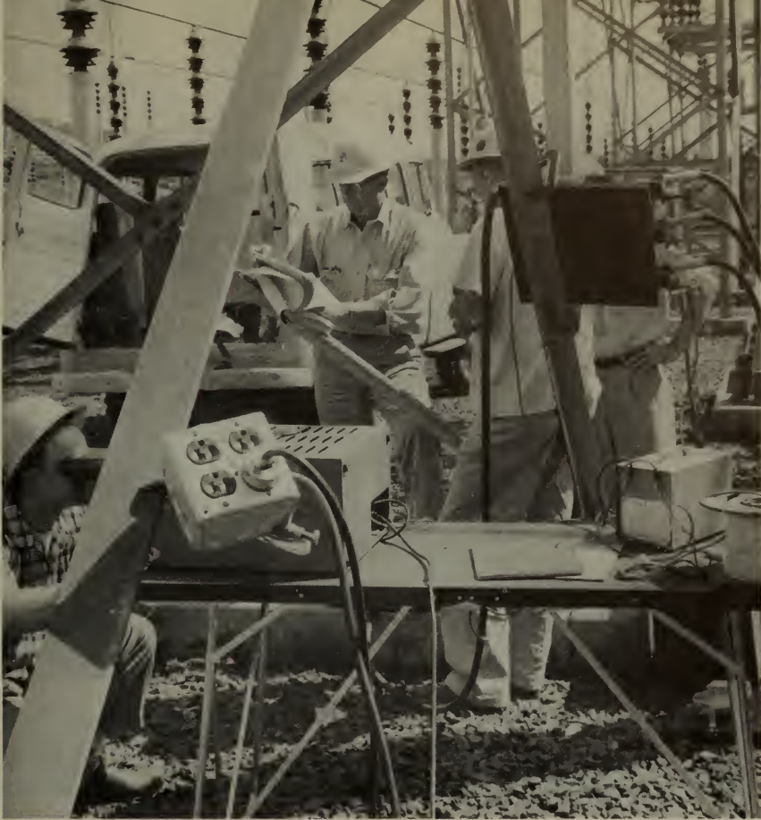
A Bonneville Power Administration testing crew checks out a fault locator and phase selector at one of BPA's large substations.
