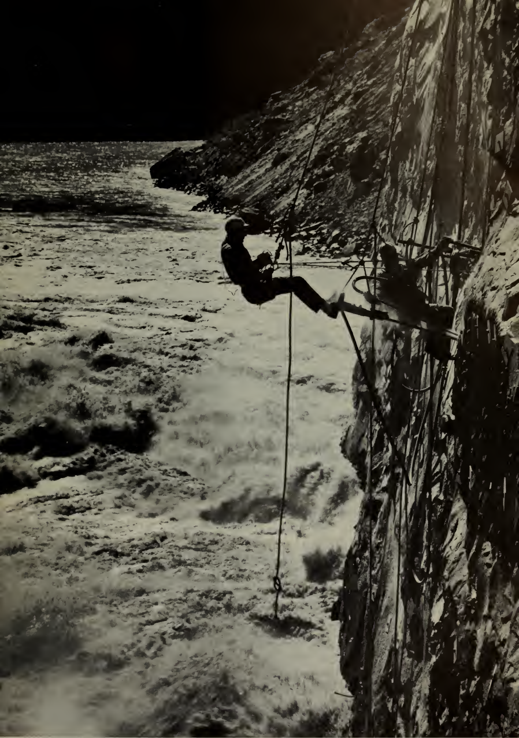
Highscalers drill on the canyon wall just above the rushing water as it pours from the right diversion tunnel.
