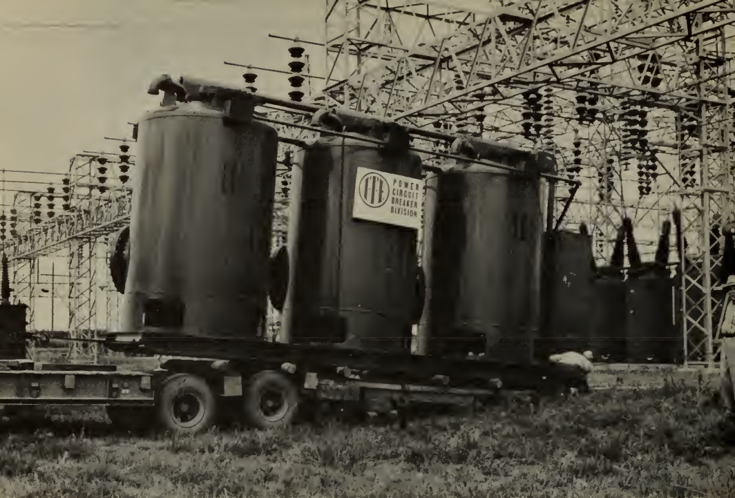
Breakers installed at Spa substation, Clinton, Mo. Extensive expansion of these installations was required to provide for interconnection of Kansas City Power and Light Co. and Missouri Public Service Co., Kansas City, Mo.
