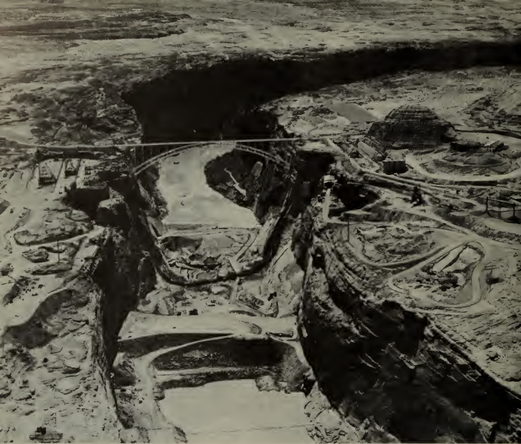
Aerial view looking downstream at Glen Canyon Dam site as excavation work has been almost completed. The upstream cofferdam is 160 feet high.
