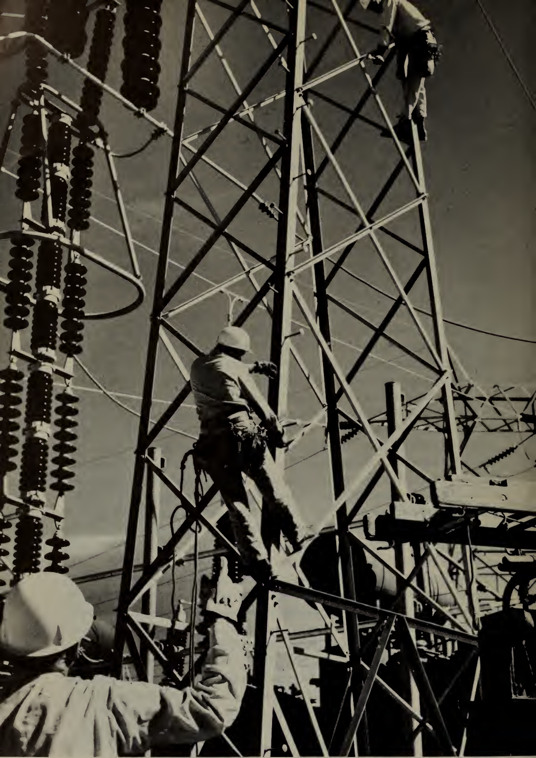
Workmen on the 230-kilovolt bus structure in the substation yard at the Watertown substation, South Dakota.
