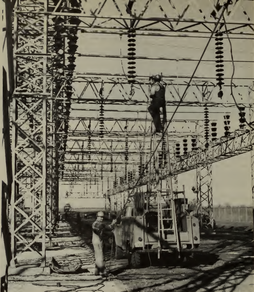
Southwestern Power Administration construction crew at work on new section constructed at SPA substation, Springfield, Mo., to provide for increased capacity resulting from the completion and interconnection of the department's Table Rock to Springfield 161-kilovolt transmission line placed in full commercial operation in fiscal year 1960.
