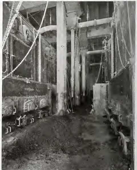
Boiler Room—The Wanamaker Power House, Philadelphia, Pa.
