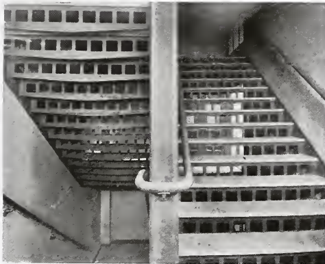
Double Fire Tower Stairs—The Wanamaker Building. D. H. Burnham & Co., Architects. Philadelphia, Pa.
