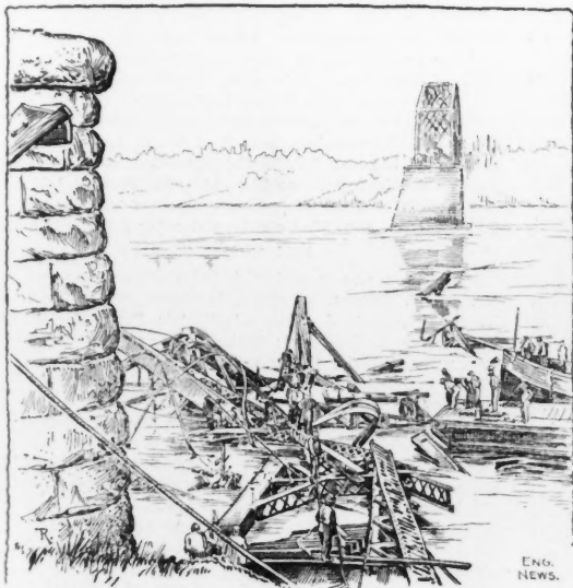
FIG. 3. VIEW OF WRECK OF THE NEW YORK & OTTAWA R. R. BRIDGE LOOKING NORTH FROM ABUTMENT ON AMERICAN SHORE.
