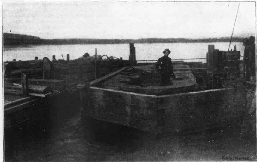
FIG. 4. VIEW OF PIER 2 FOR NEW YORK & OTTAWA R. R. BRIDGE UNDER CONSTRUCTION.
