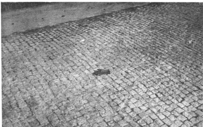
Half Regular Stone Block Pavement on the First Experimental Road at Nanking, China
