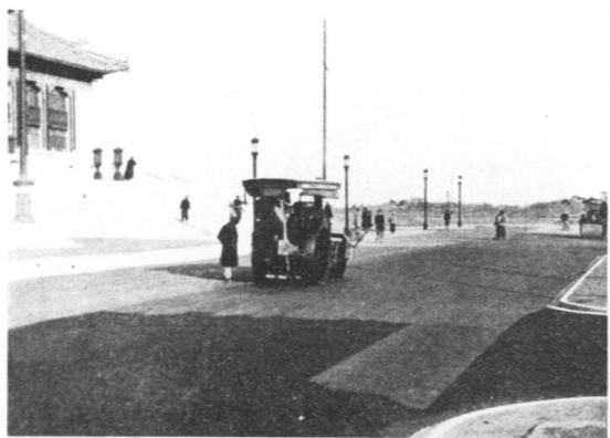
The cold laid bituminous pavement at Shanghai, by the Public Works Department of the Shanghai Municipality.
