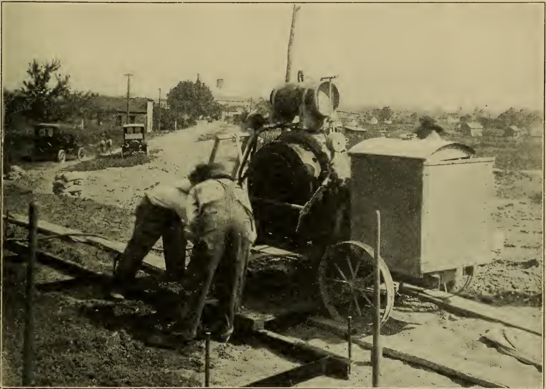
A small self-contained mixer-engine outfit at work on a job of mixing concrete for a concrete walk. Such an outfit is a profitable, labor-saving and efficient piece of equipment.
