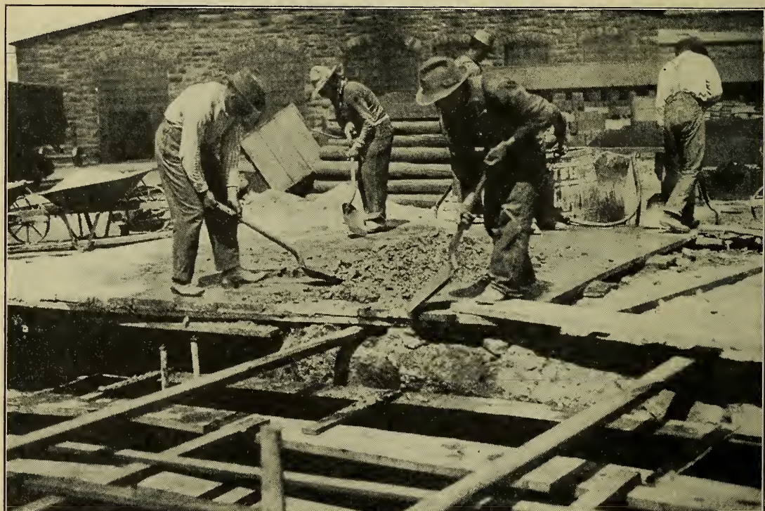
If the mixing platform can be placed near where concrete is to be deposited, the concrete may be shoveled directly from the platform into the forms.
