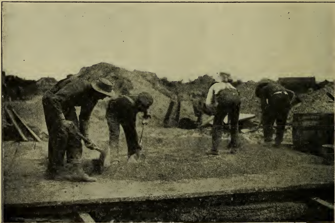
Men using square-pointed shovels turn the sand and cement thoroughly several times until the streaks of brown and gray have merged into a uniform color.
