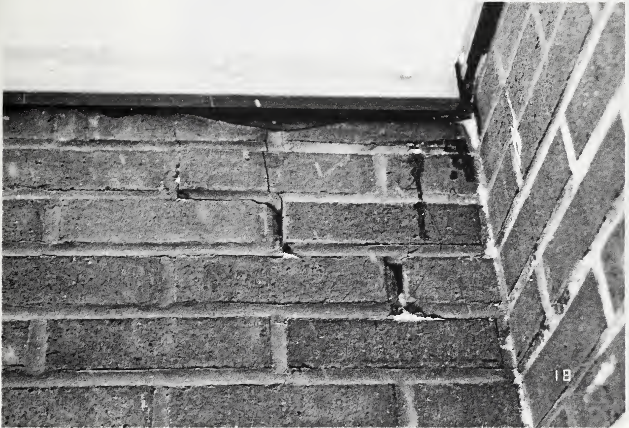
Figure 5.7.2. Cracks at intersection of parapet and penthouse walls
