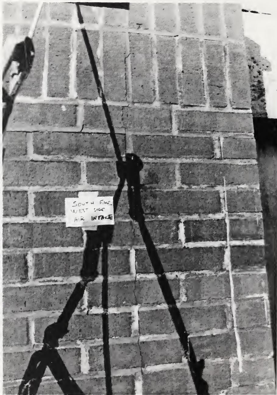
Figure 5.6.4. Vertical crack west of louver opening on south elevation
