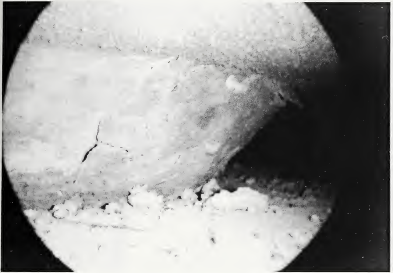
Figure 5.4.6. Borescope photograph inside joint of 6-G2/5 showing evidence of distress in the bearing button
