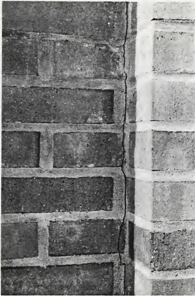
Figure 5.6.7. Crack in recess of north corner, east elevation
