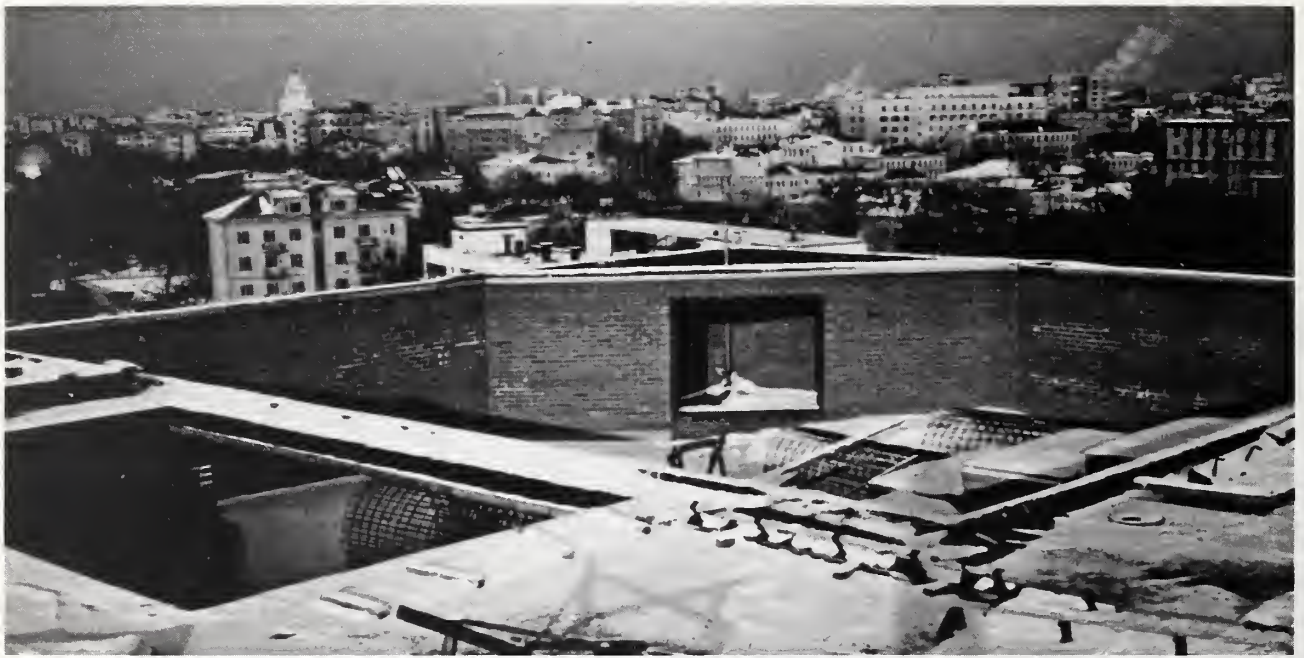
Figure 5.7.1. Northeast section of roof showing parapet walls, snow melting room and recess in penthouse wall
