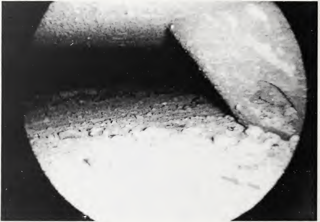
Figure 5.4.5. Borescope photograph inside joint of 6-G2/6 showing that no grout has been placed around the bearing button (at right)
