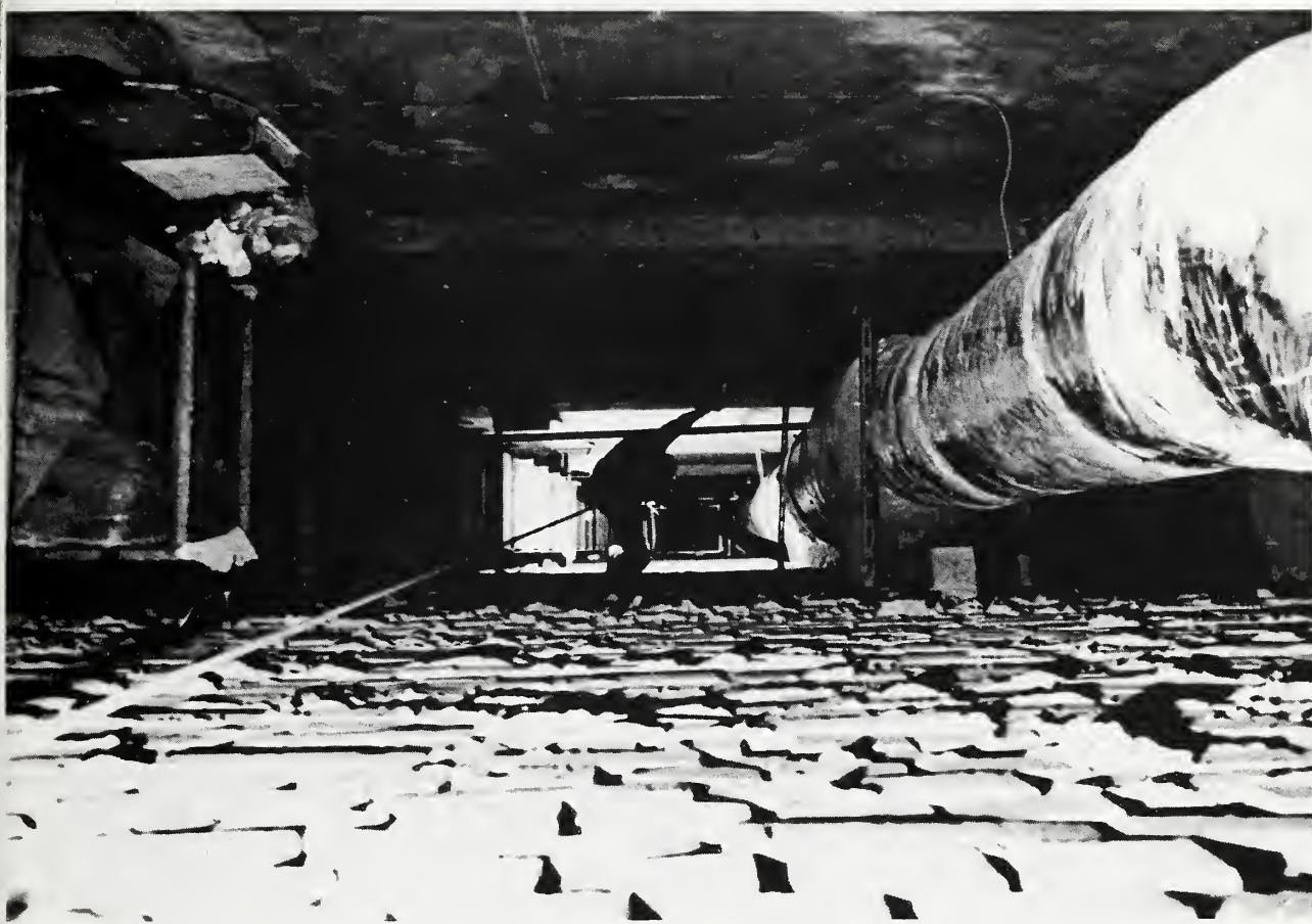
Figure 5.4.10. NBS investigator descends mechanical chase at northwest core for inspection of interior shear wall joints
