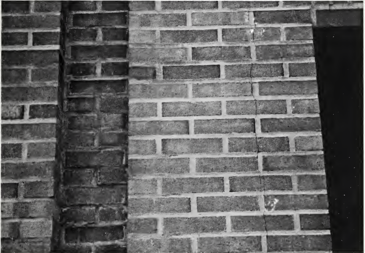
Figure 5.6.9. Crack near window at east corner of north elevation
