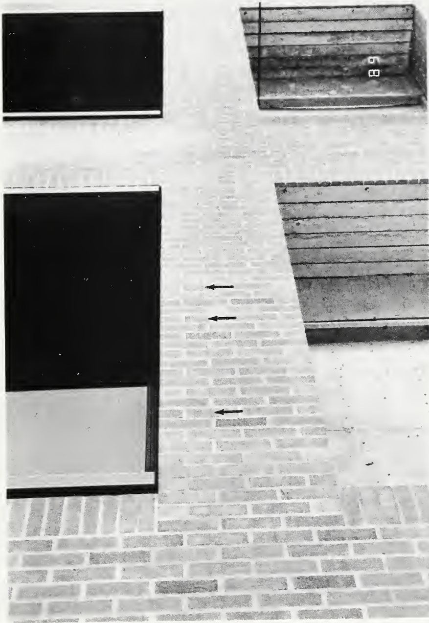
Figure 5.6.11. Crack in second story pier at column A1/5, west elevation
