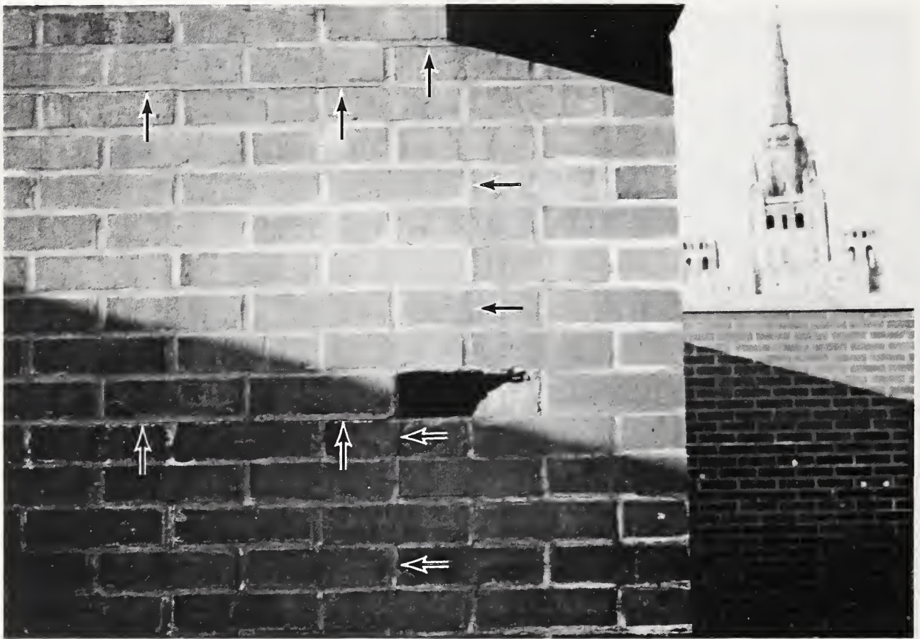
Figure 5.7.3. Brick removed at intersection of vertical and horizontal cracks in penthouse wall, northeast section
