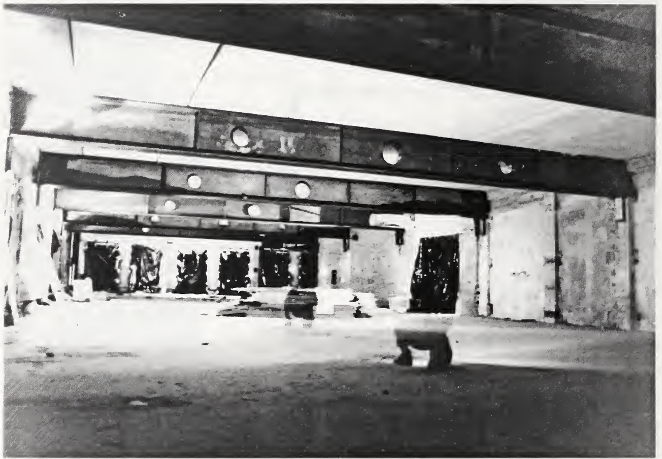
Figure 2.3.11. View along east-west direction showing 13.2 m long I-beams spanning between the exterior column line and interior core
