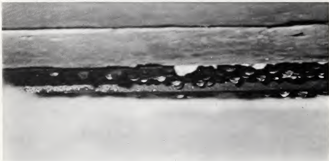
Figure 5.9.1. Water in soffit cavity above windows
