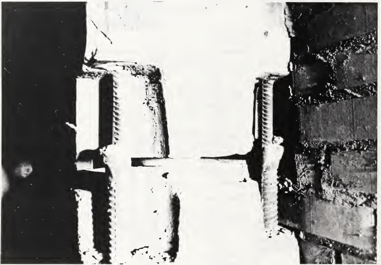
Figure 2.3.9. Typical reinforced concrete column connection prior to filling with grout and concrete (The joint tie is not present)
