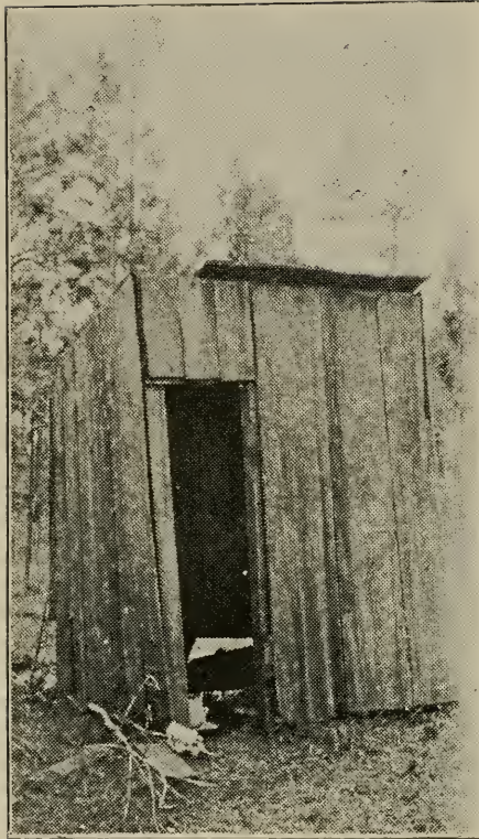
POOR SCHOOL CLOSET.
