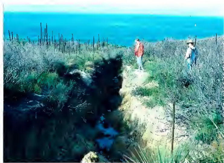
Figure 1: A previously in-filled and subsequently deeply gullied section of the Coast Walk, 1991.
