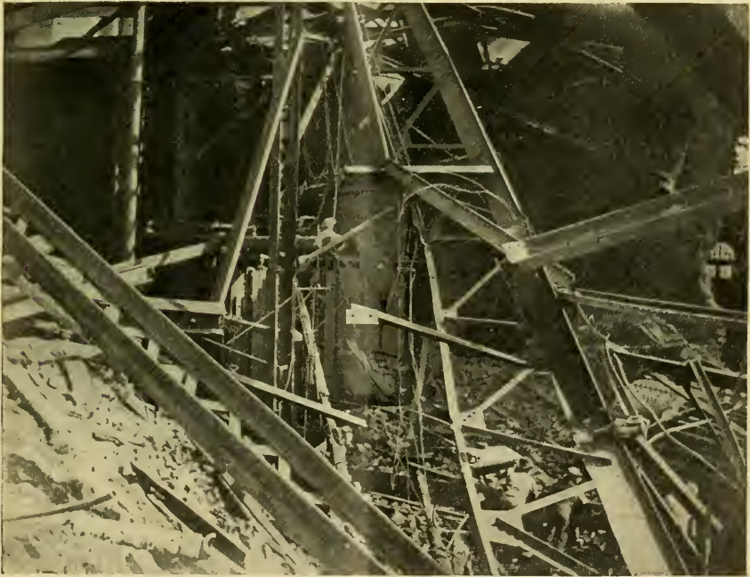
FIG. 3.— SHOWING SOME OF THE WRECKAGE IN DETAIL.
