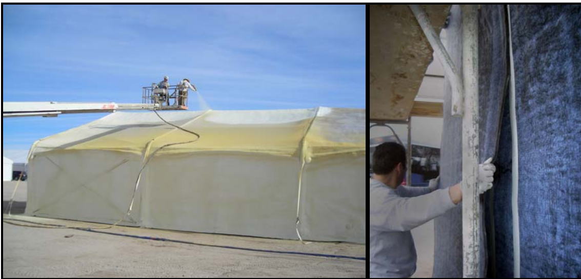
Figure 14. Gaco Western Polyfoam (left) sprayed application. FOB King at Fort Irwin. Aspen Aerogel (right) sheets applied to a building wall. (From Aspen Aerogels, 2006)
