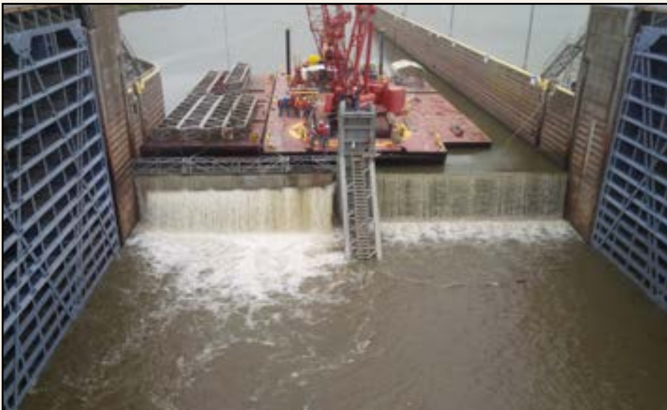
Lock dewatering 2016: Lock 16 MKARNS (McClellan- Kerr Arkansas River Navigation System) SWT District
