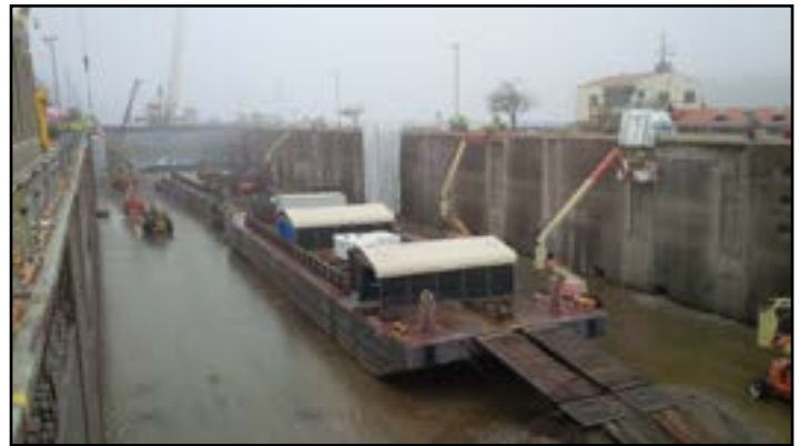
Lock Dewatering 2017: Figure 11 Lock 17 Upper Mississippi River equipment and fleet in use MVR District
