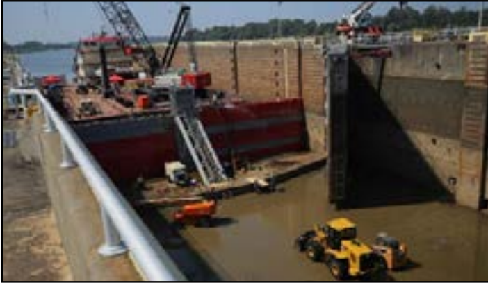
Lock Dewatering 2016: Figure 13 (see pg. 16) Lock 16 MKARNS Equipment and Fleet in use SWT District
