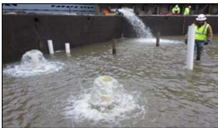
Lock dewatering 2016: Figure 10 Lock 13 Upper Mississippi River Weep holes stand pipes MVR District
