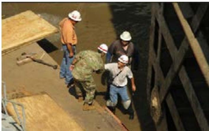
Lock Dewatering 2016: Figure 9 (see pg. 16) Lock 6 MKARNS command site visit. SWL District
