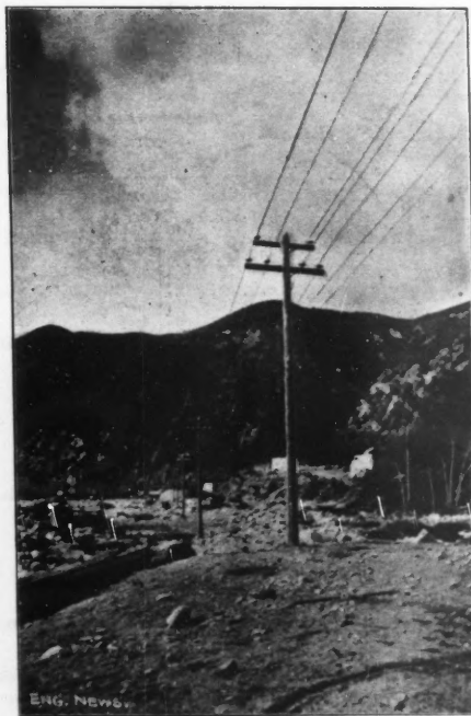
Fig. 16.—View of Pole Line for 80-Mile Transmission.
