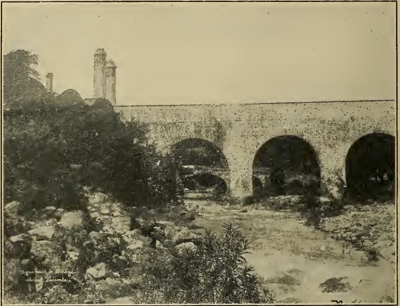
FIG. 1.—Masonry aqueduct and masonry bridge adjoining large hacienda in the State of Morelos, Mexico.
