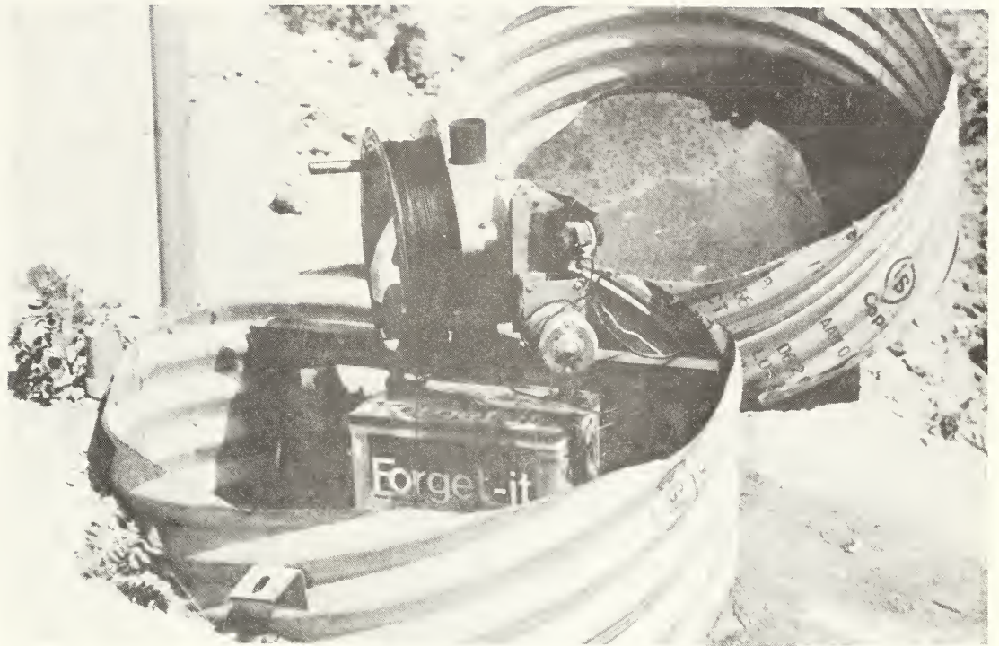
Figure 15.--Input structure which can be covered and locked.
