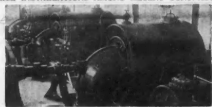
View of Generator Room.
