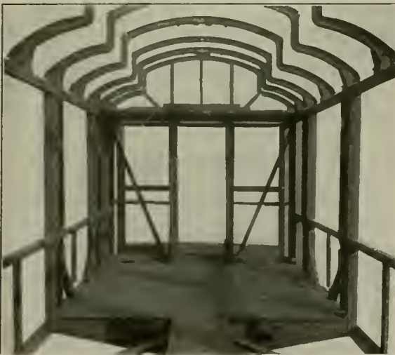
A View of the Framing at the End of the Car, Also Showing the Body Bolster and Underframe Stiffening Plate
