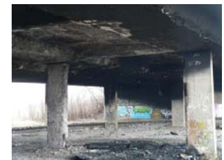
Fire incident on the highway bridge in Dormagen on 14 February 2012
