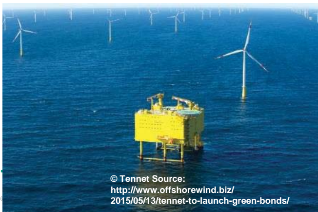
Example infrastructure node
