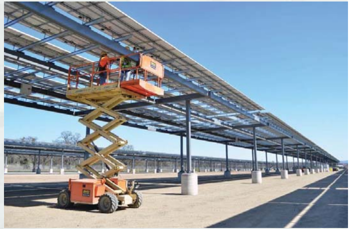
Workers complete electrical connections as part of a solar microgrid project at Fort Hunter Liggett, CA
