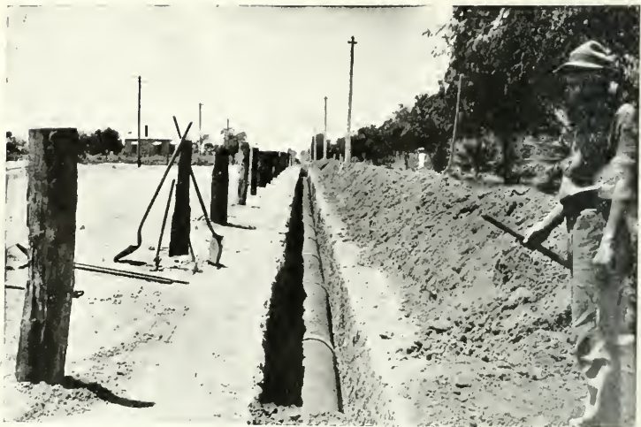
Section of 1\frac{1}{2} miles of 18 inch "Pioneer" Wood Pipe, installed for Mildura Irrigation Trust.
