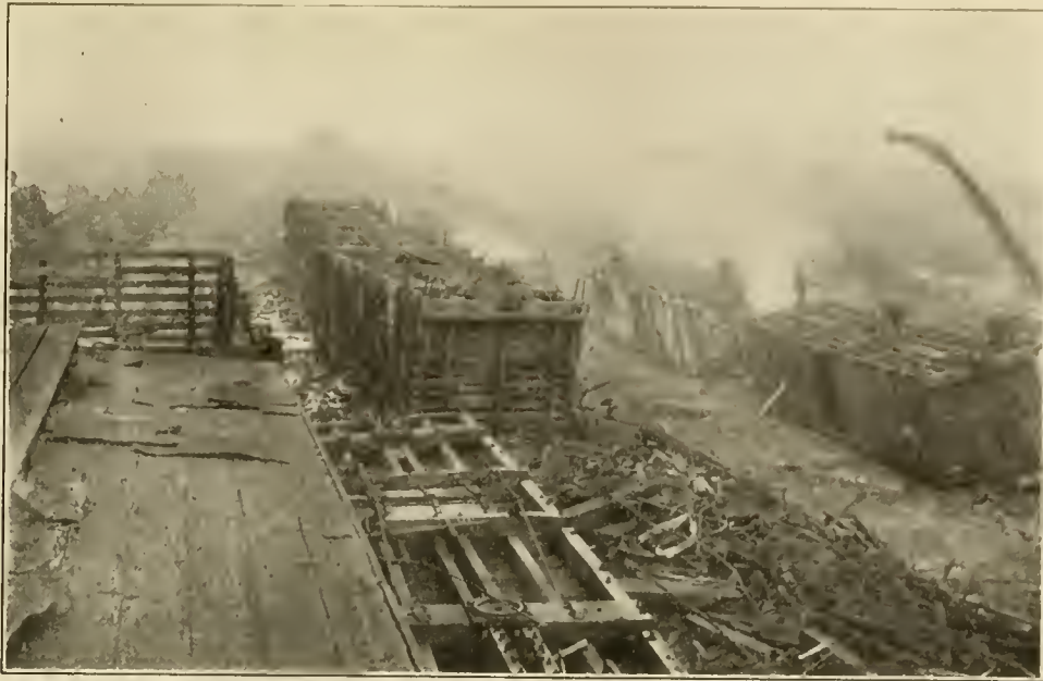
FIG. 3.—OLD WOODEN FREIGHT CARS BEING DISMANTLED AT THE METAL YARD PREPARATORY TO BEING BURNED.
