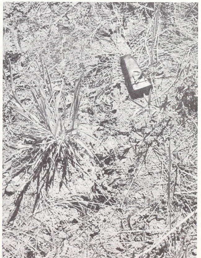
Figure 60. Tension cracks may be hard to find, but they indicate active soil movement
