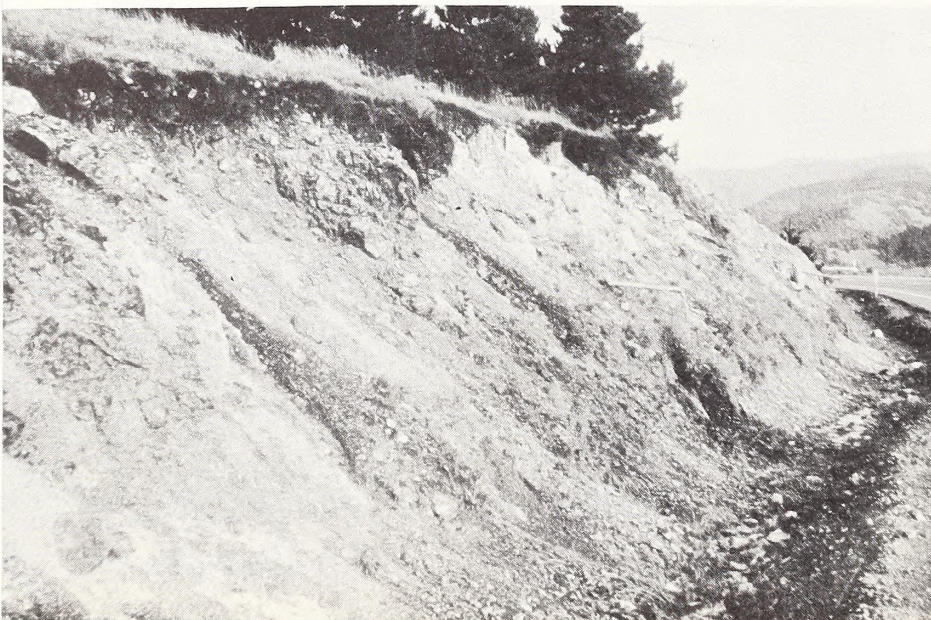
Figure 103. Perforated pipe may be needed to remove ground water from embankments in serpentine material. Note the volume of water issuing from the pipe at the right of center.
