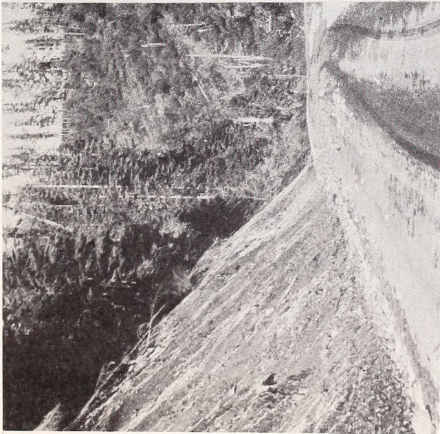
Figure 94. Rockfalls in deeply weathered schist. Note tipped tree.
