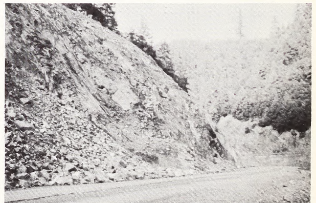
Figure 39. A photo of the rockslide illustrated at point B in Figure 23. Note how the shifting rock is lifting the road and moving it to the right towards Cow Creek
