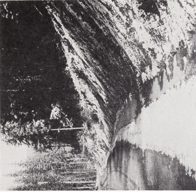
Figure 96. Small slumps cause impeded ditch drainage.
