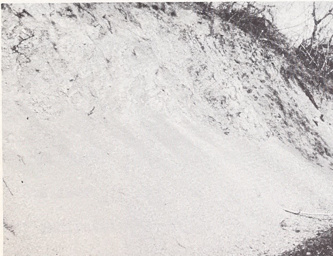
Figure 8. Nestucca formation showing weathered siltstone
