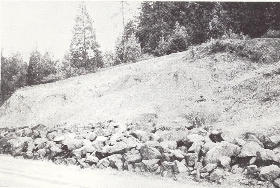
Figure 102. Heavy riprap may be used to support slumping embankments in serpentine material.
