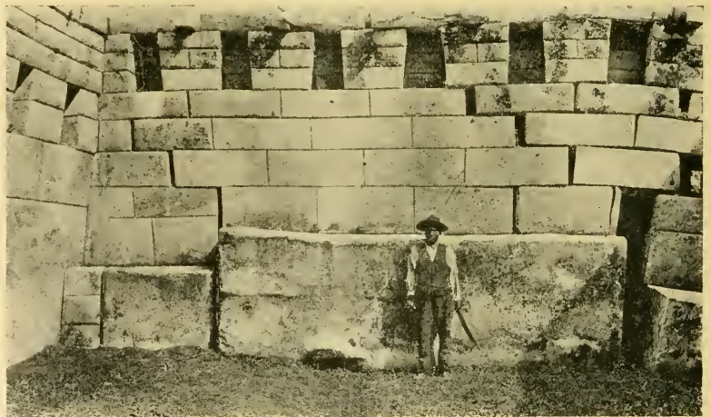
FIG. 4.—Machu Picchu. Sacred plaza. Chief temple, north wall, interior, showing the cracking caused by the settling of the east wall. Notice the care with which the size of the stones is made to decrease gradually in each ascending tier. The main altar stone is 14 ft. in length. Copyright by the National Geographic Society.
