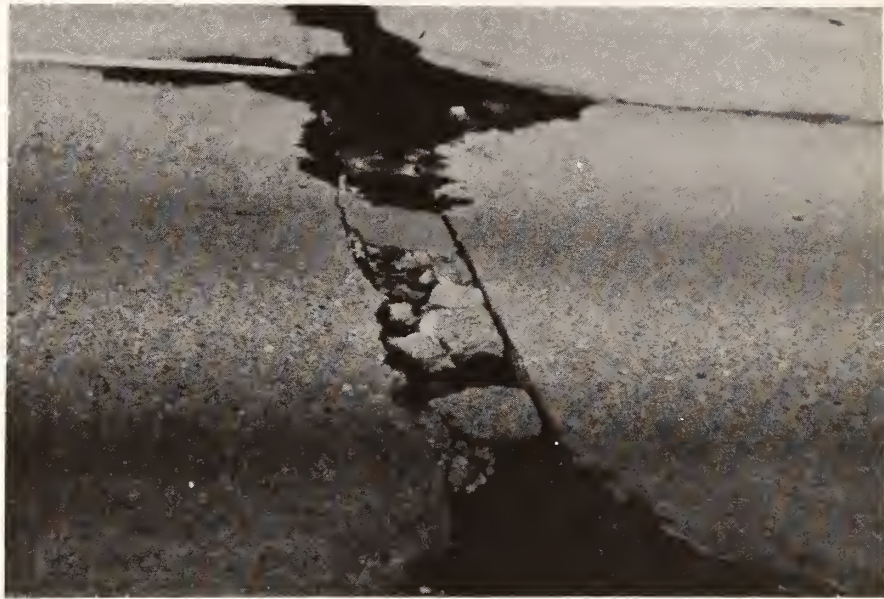
Figure C.15. High Severity Joint Load Transfer System Associated Deterioration.
