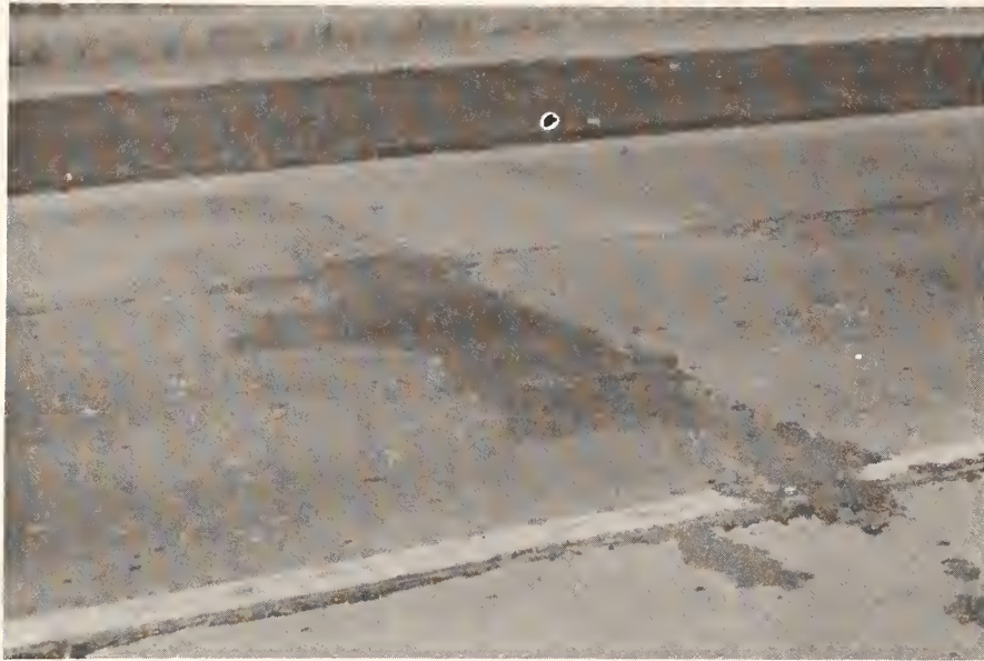
Figure C.33. Patch Adjacent Slab Deterioration ("D" cracking & temporary patching).
