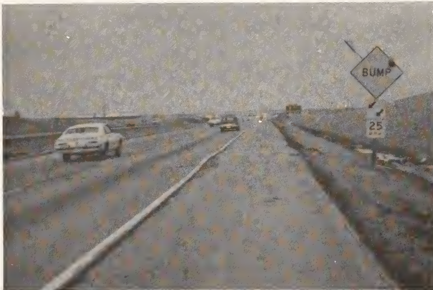
Figure C.51. Swell Due to Frost Heave.
