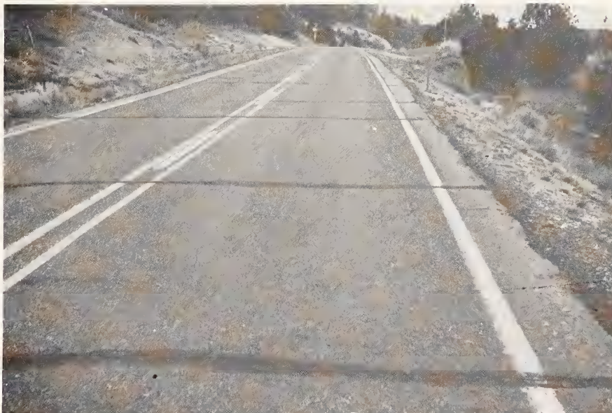
Figure B.36. Medium Severity Transverse Cracking.
