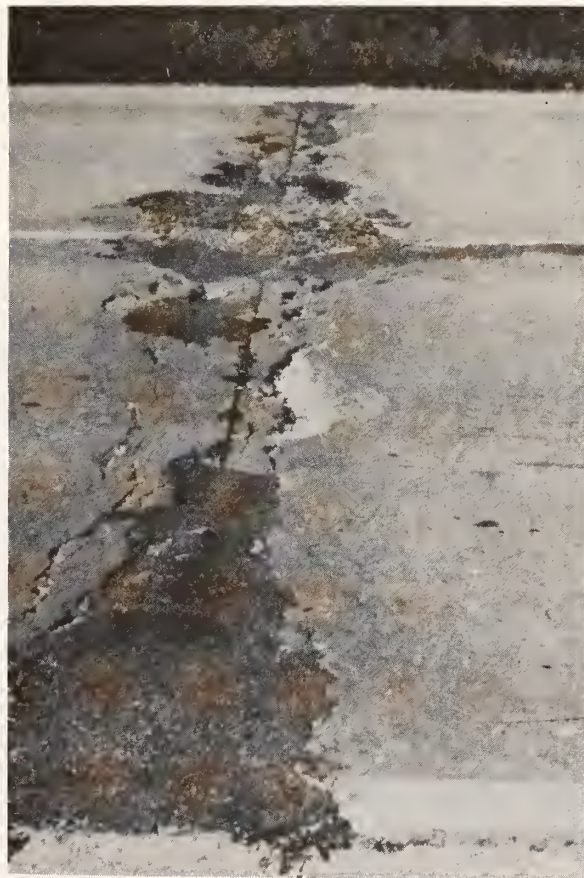
Figure C.47. High Severity Spalling.
