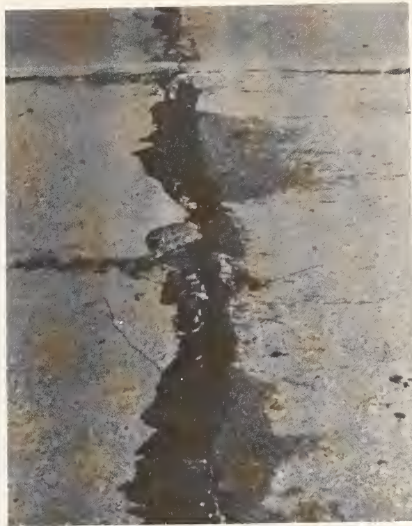
Figure C.36. Low Severity Pumping (Water Bleeding).
