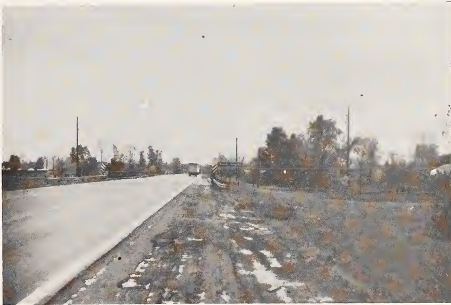
Figure B.67. High Severity Raveling and Weathering.
