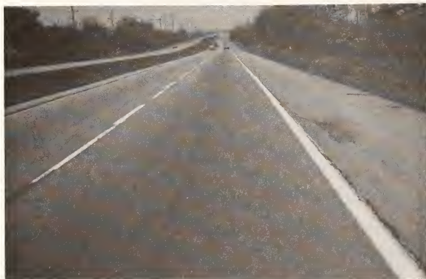
Figure B.32. Medium Severity Lane/Shoulder Joint Separation (note separation near outside of edge paint strip). (See Figure 2.31 for photo of high severity lane/shoulder joint separation.)
