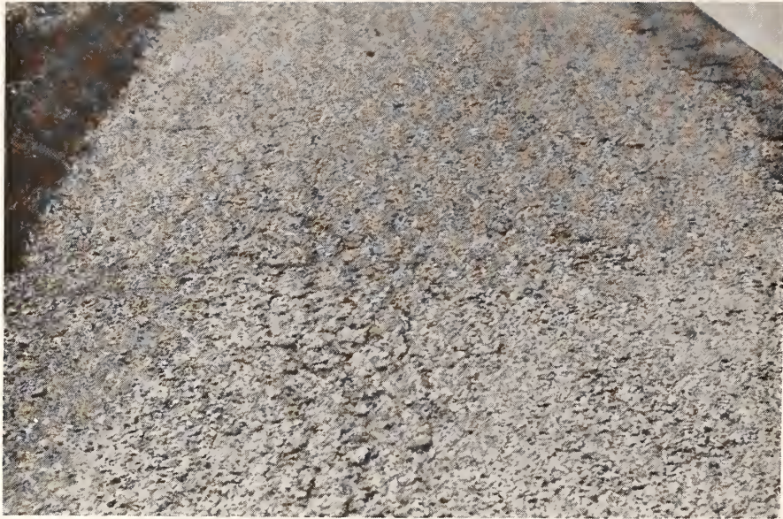
Figure B.64. Medium Severity Raveling and Weathering.
