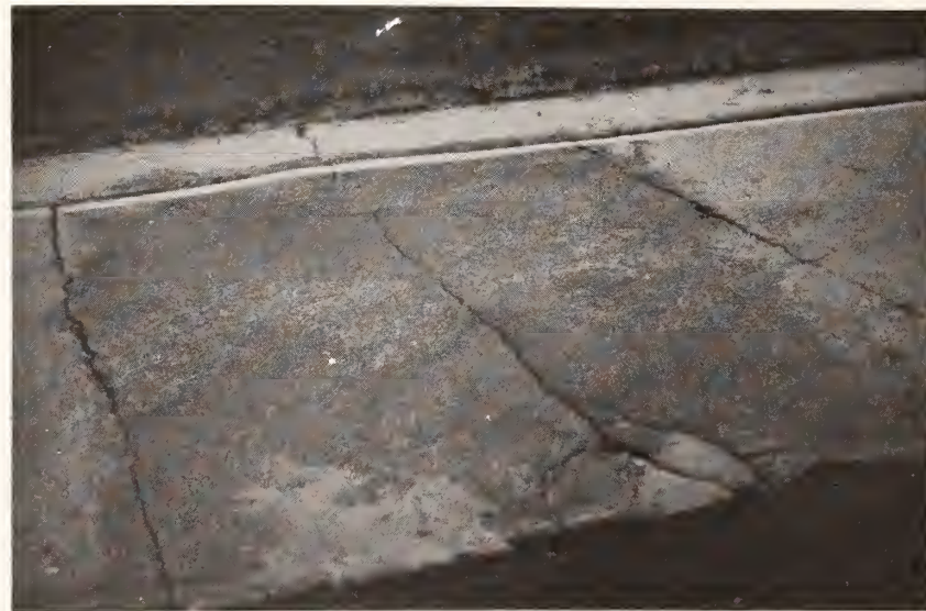
Figure B.74. Medium Severity Swell Occurring at a Patch Due to Buckling of Concrete Slab Beneath Asphalt Surface.
