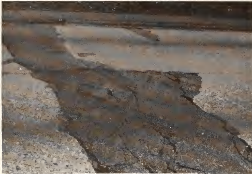
Figure C.28. High Severity Asphalt Patch Deterioration.
