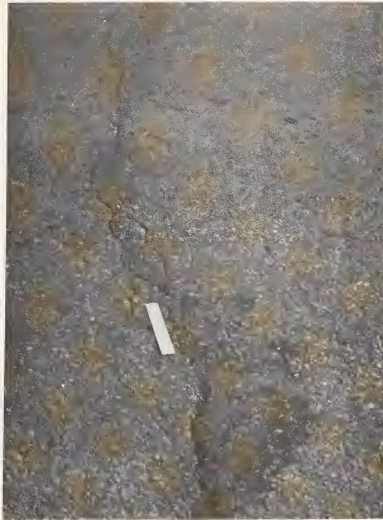
Figure B.39. Medium Severity Transverse Cracking.
