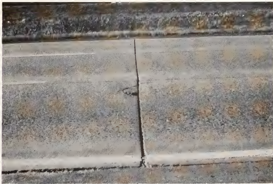
Figure C.43. Low Severity Spalling.
