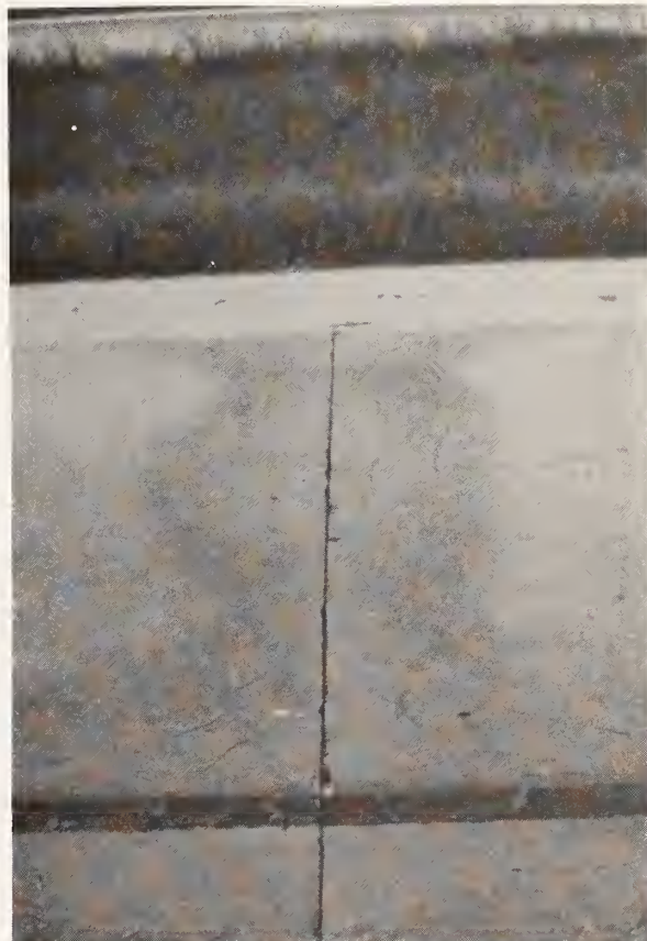
Figure C.6. Medium Severity "D" Cracking.
