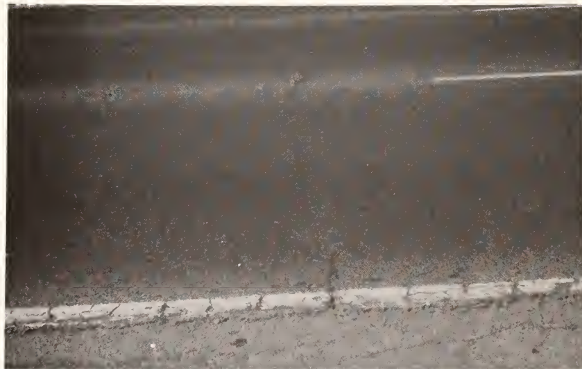
Figure B.25. Low Severity Joint Reflection Cracking from Transverse Joint in PCC Slab.
