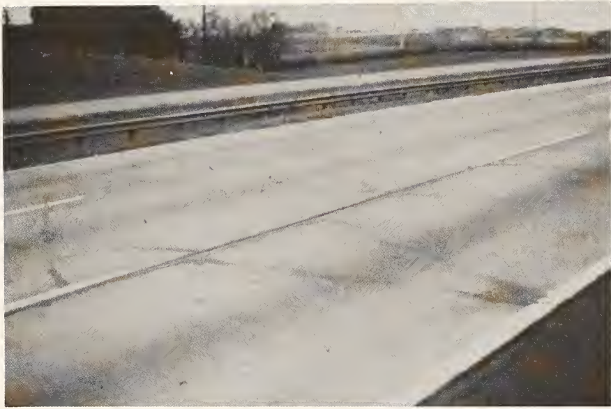
Figure C.52. Swell Due to Expansive Soil.
