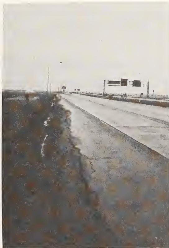
Figure B.23. High Severity Depression in Shoulder (high severity alligator cracking also exists and would be recorded in addition to the depression).
