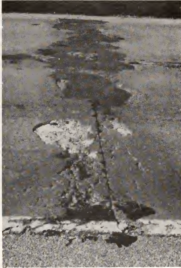
Figure C.9. High Severity "D" Cracking.
