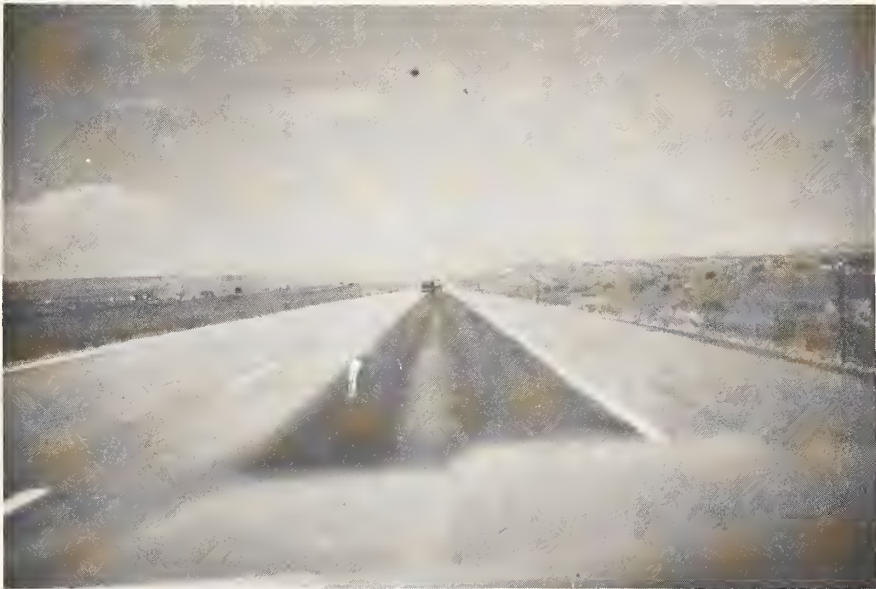
Figure B.14. Bleeding in Wheel Paths.
