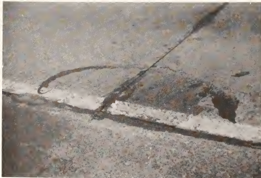
Figure C.3. Low Severity Corner Break.
