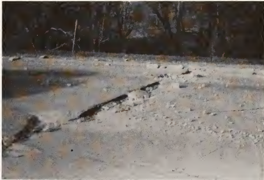
Figure C.2. High Severity Shattering Type Blow-up.
