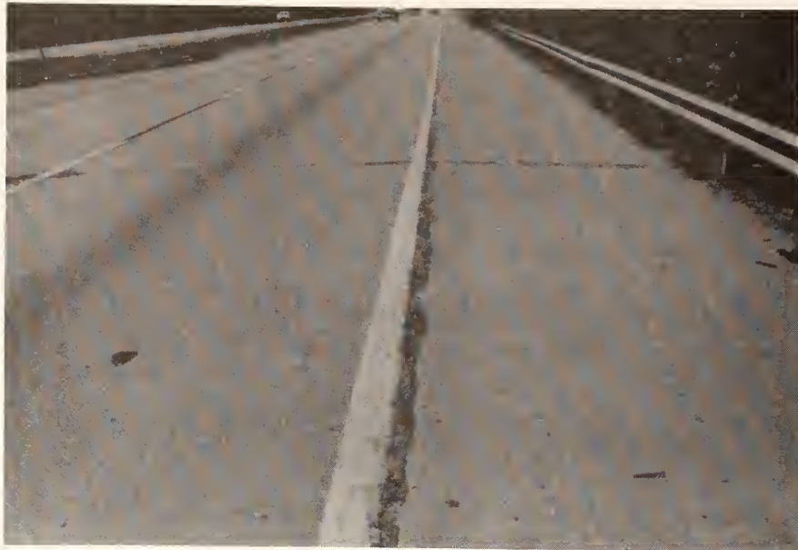
Figure C.22. Lane/Shoulder Separation (PCC Shoulder).
