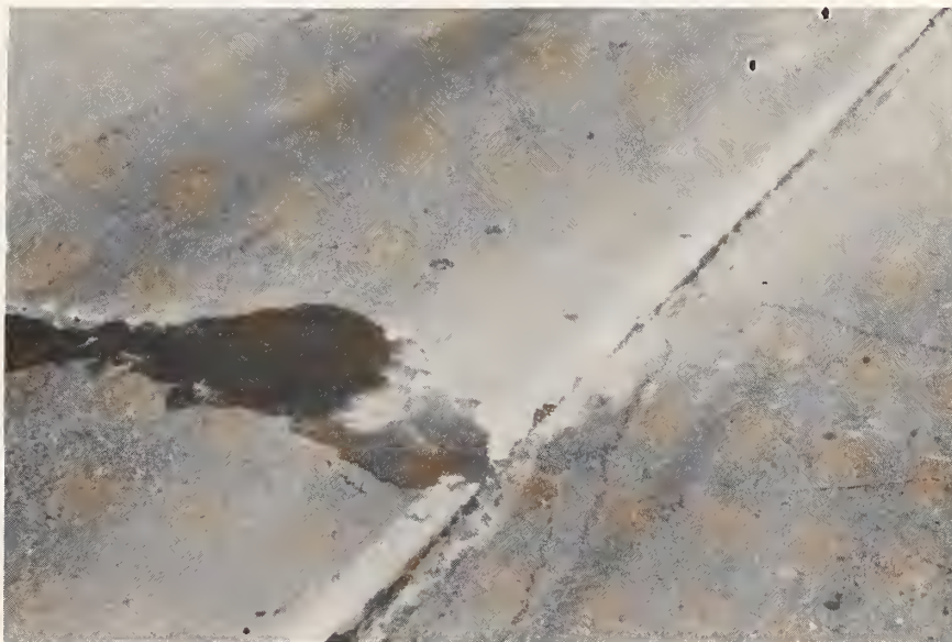
Figure C.37. Medium Severity Pumping (pumped material like this occurs only at a few of the joints and cracks).
