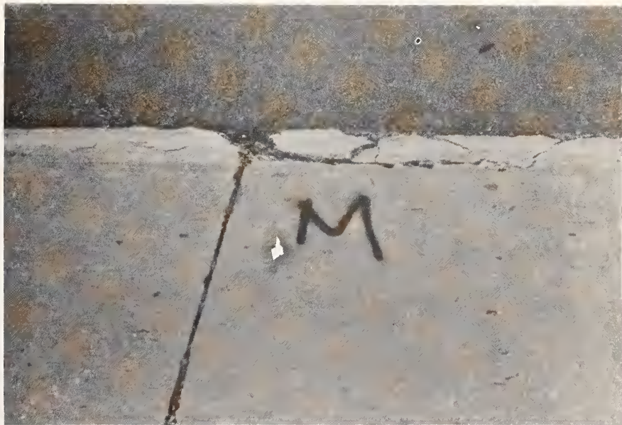
Figure C.17. Medium Severity Joint Seal Damage.
