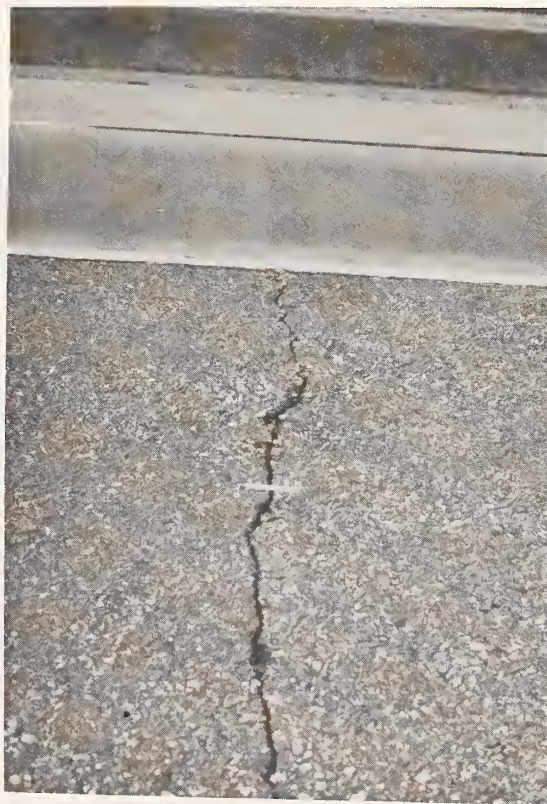
Figure B.40. Medium Severity Transverse Cracking Across Shoulder.
