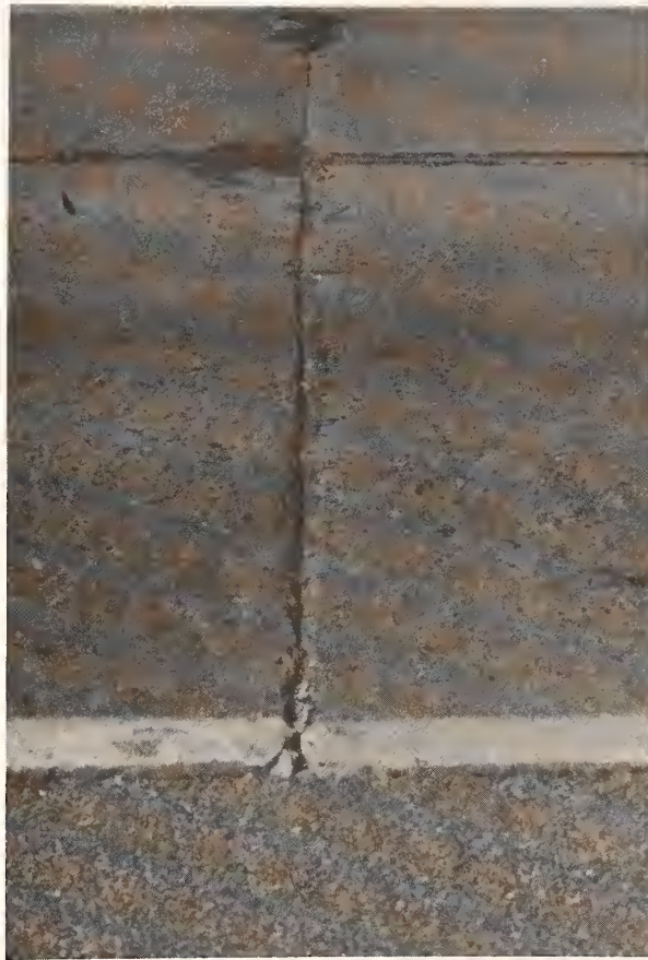
Figure C.18. High Severity Joint Seal Damage.
