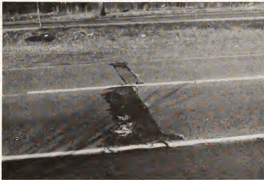
Figure C.14. High Severity Joint Load Transfer System Associated Deterioration.
