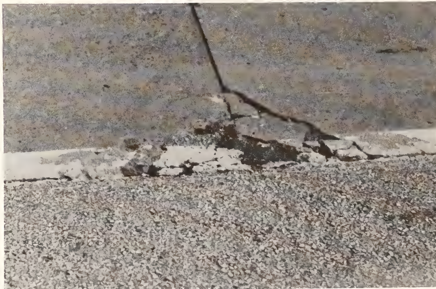
Figure C.48. Medium Severity Corner Spall.
