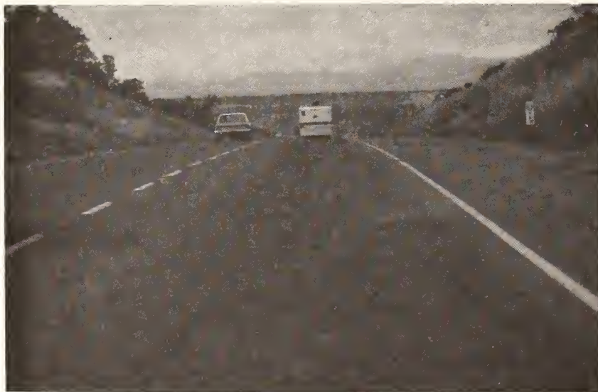
Figure B.58. Medium Severity Pumping (stabilized base is pumping)(Note: see also Figure 2.9 for medium severity pumping photo).
