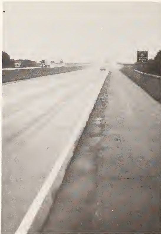
Figure B.47. Low Severity Patch Along Shoulder Joint.
