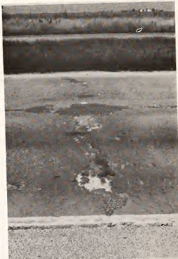
Figure C.8. High Severity "D" Cracking.
