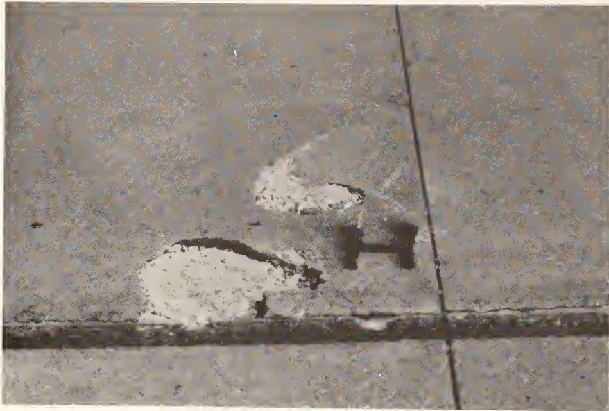
Figure C.49. High Severity Corner Spall.
