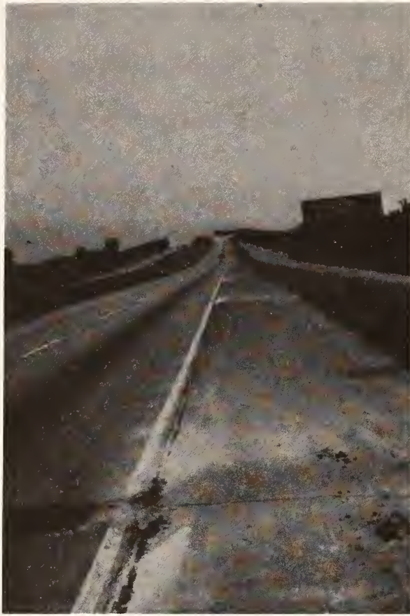
Figure C.38. High Severity Pumping.
