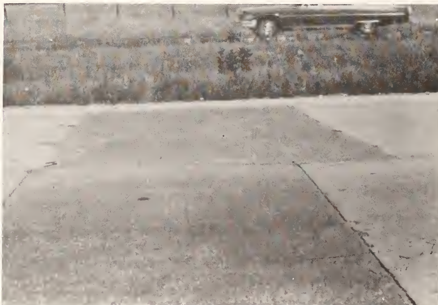
Figure C.27. Low Severity Asphalt Patch Deterioration.
