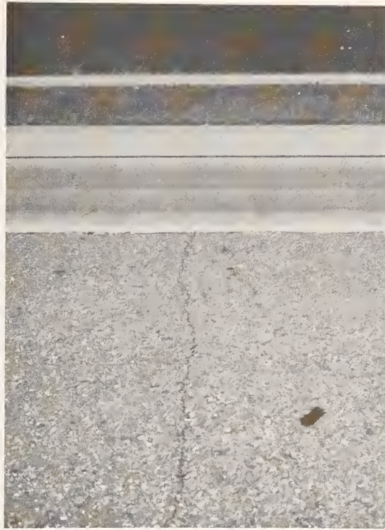
Figure B.35. Low Severity Transverse Cracking Across Shoulder.
