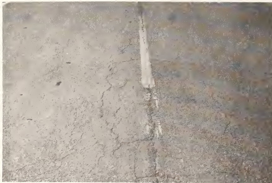
Figure B.16. Low Severity Block Cracking Near Centerline.
