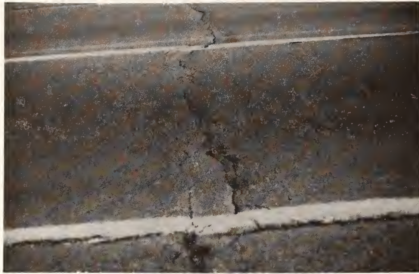
Figure B.41. High Severity Transverse Cracking.
