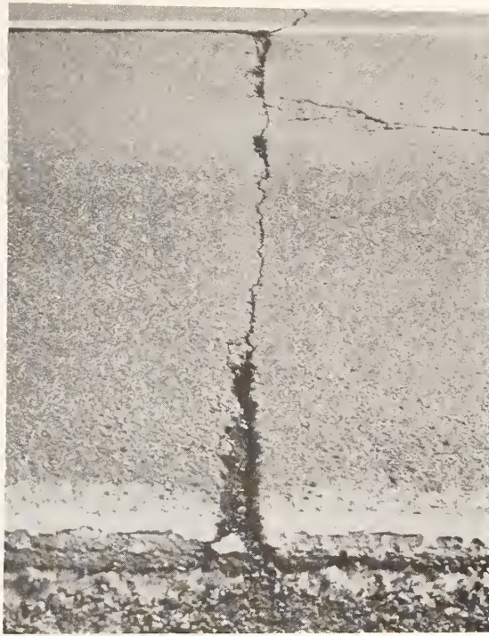
Figure B.43. High Severity Transverse Cracking.
