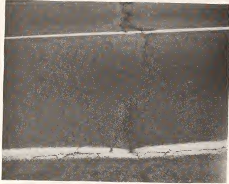
Figure B.37. Medium Severity Transverse Cracking.
