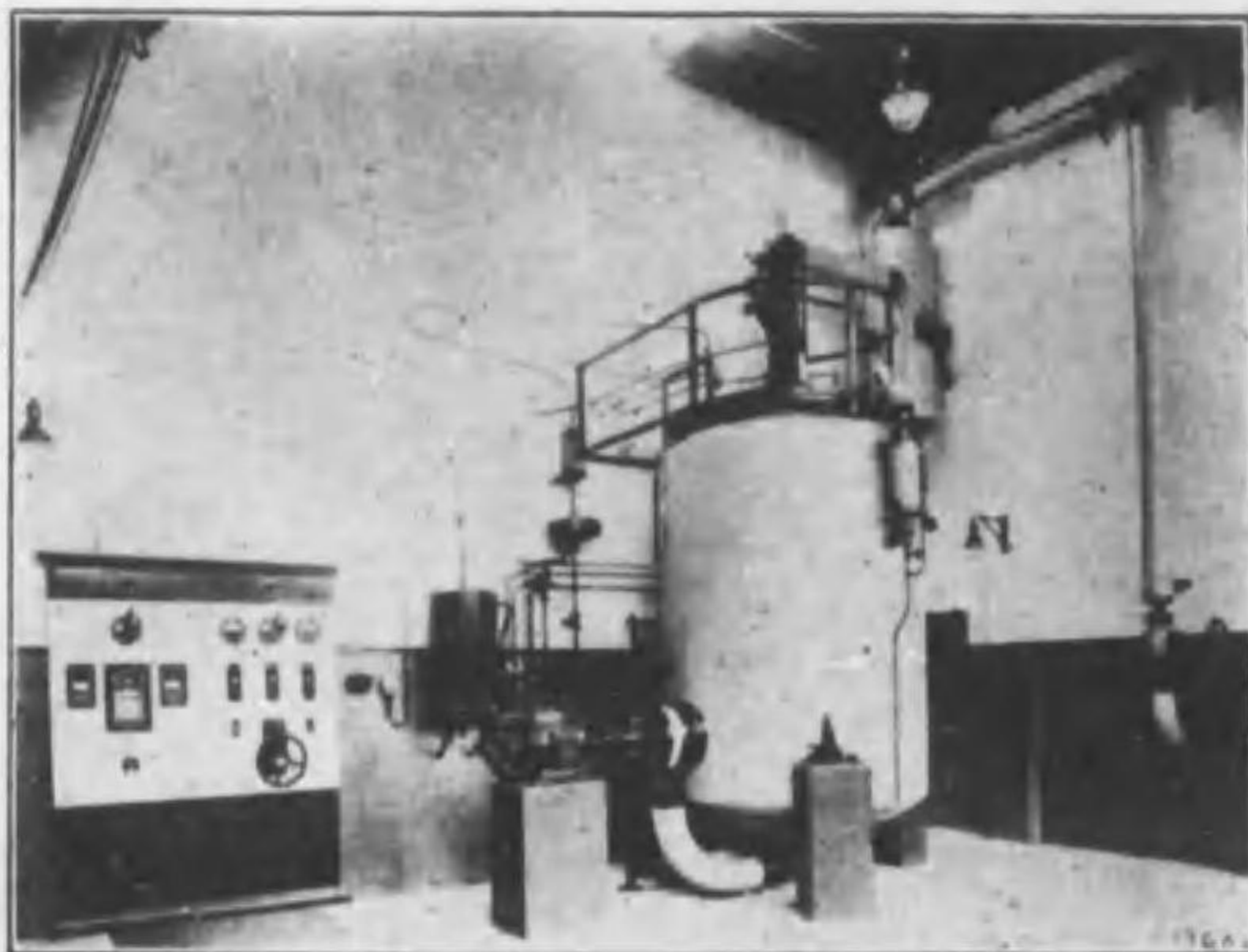
Sulzer Electric Steam Boiler in a Paper Mill in Bern. Working Pressure 150 lbs./sq.in., 3,500 Kw., 3 Phase, 10,000 Volts, with automatic regulation of water level.
