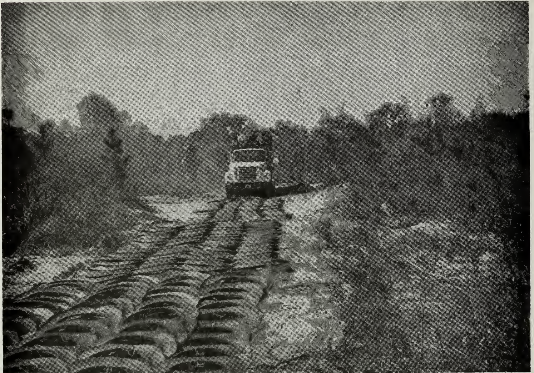
Figure 29. Narrow width of mats could create maneuvering and load distribution problems.
