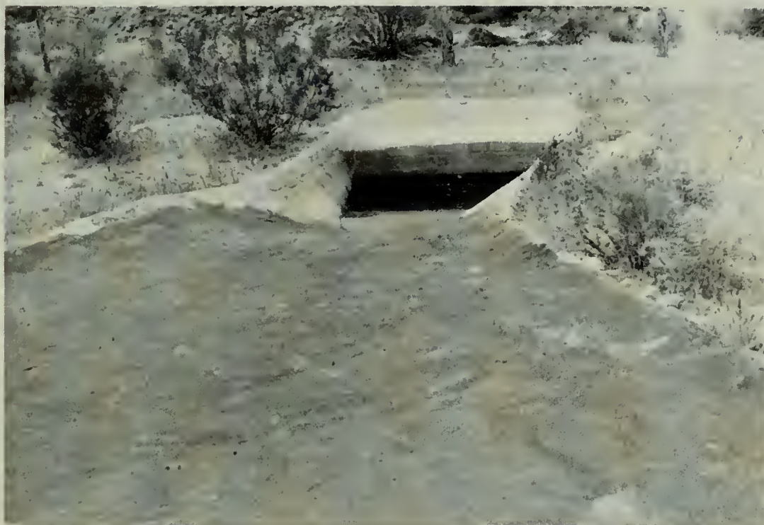
Figure 12. Concrete open-basin type water catchment.
