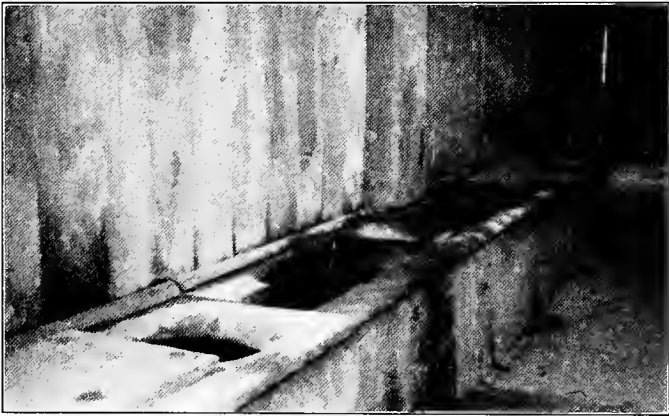
THE PRIVIES OF THE RIDGELY SCHOOL ARE IN SERIOUSLY BAD CONDITION
