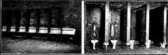
THE URINALS ARE OF POOR DESIGN AND THE TOILET STALLS SHOULD HAVE DOORS
