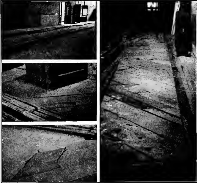
PATCHED, CRACKED, AND DEFECTIVE SECOND-HAND LUMBER USED AS SHEATHING IN THE NEW LINCOLN SCHOOL
