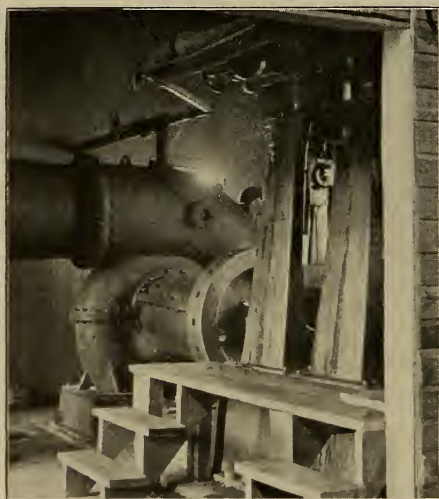
ENGINES AND PUMP.
