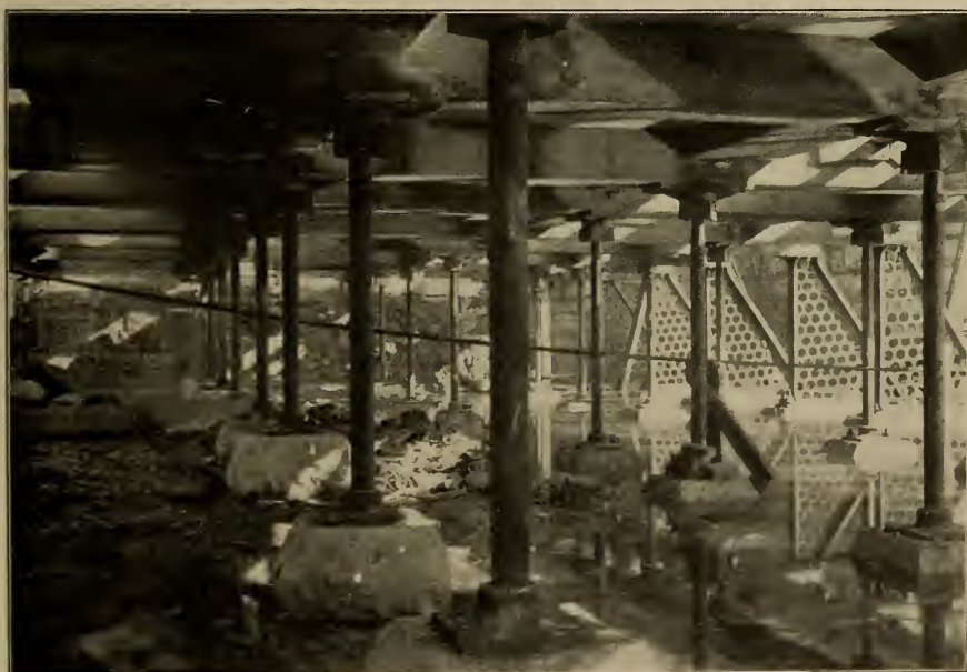
UNDER THE WHEEL PIT—ROCKFORD GENERAL ELECTRIC CO.
