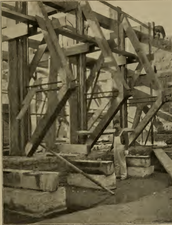
GATE POST BRACING—ROCKFORD GENERAL ELECTRIC CO.
