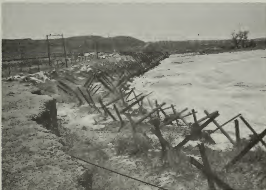
Many miles of steel jetties, riprap, and other similar protective measures have been installed by the Santa Fe Railway Co. in an attempt to protect its roadbed and track from erosion damage.
