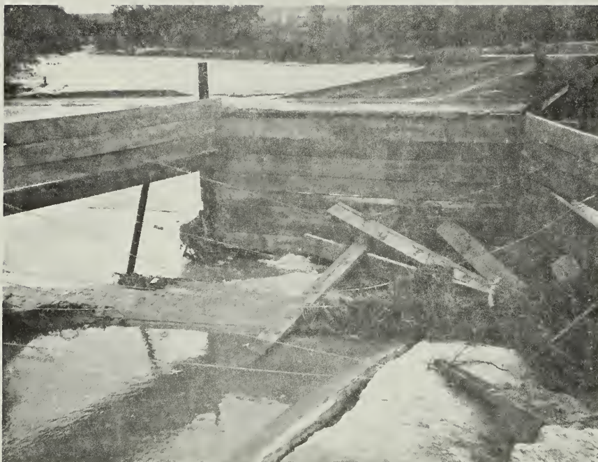
County Road and Bridge Damage at Mendota from May 1969 Flood
