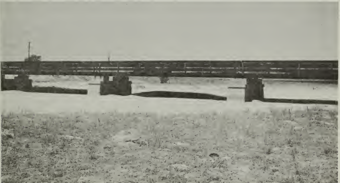
Sand accumulations in channels and deposition on the flood plain is encroaching on the effective capacity of this railroad bridge crossing Red Deer Creek. Other bridges, culverts, and the roadbed of the railroad, and the highways and county roads in the Red Deer Creek valley are similarly affected.
