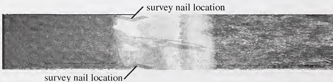
Figure 14. A single frame recorded by BMS showing two survey nails highlighted using black and white paint.
