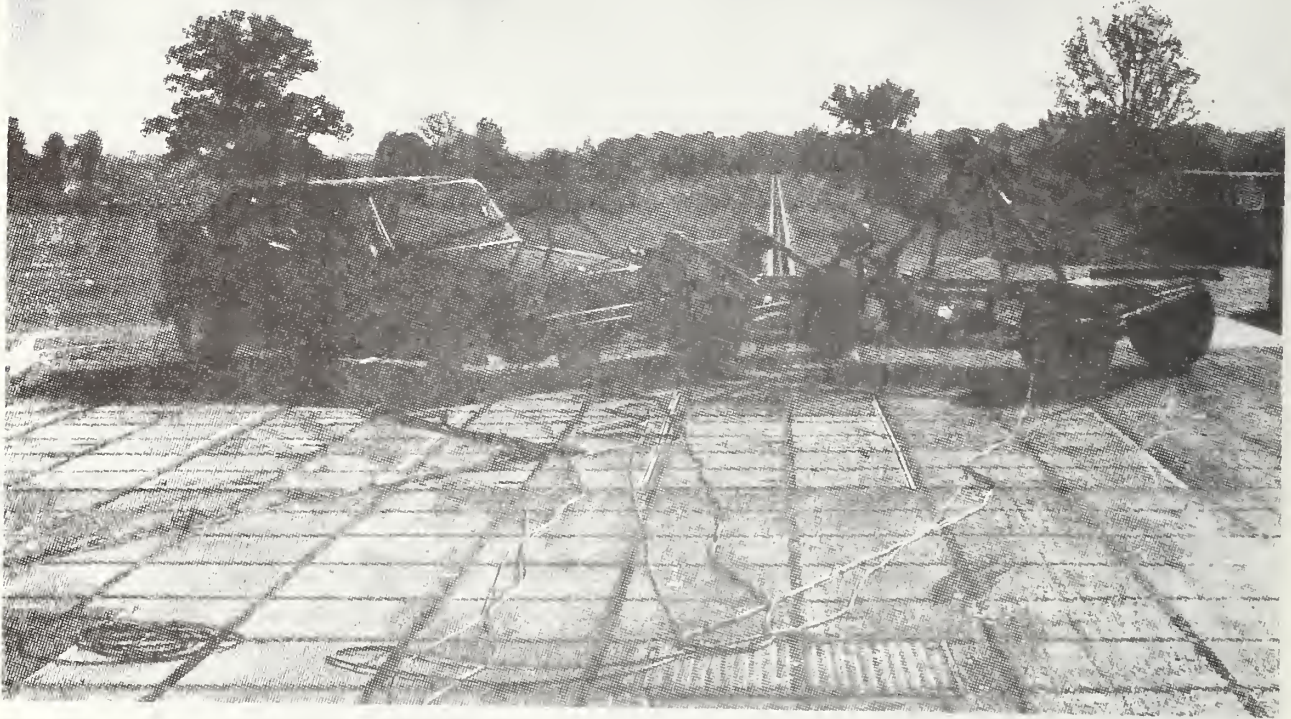
Figure A-17. POST-TEST OVERALL - VIEW 3
