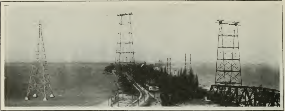
TRANSMISSION LINES, NIAGARA SYSTEM—BURLINGTON BEACH Hydro, Dominion Power and Toronto Power transmission lines looking north from bridge
