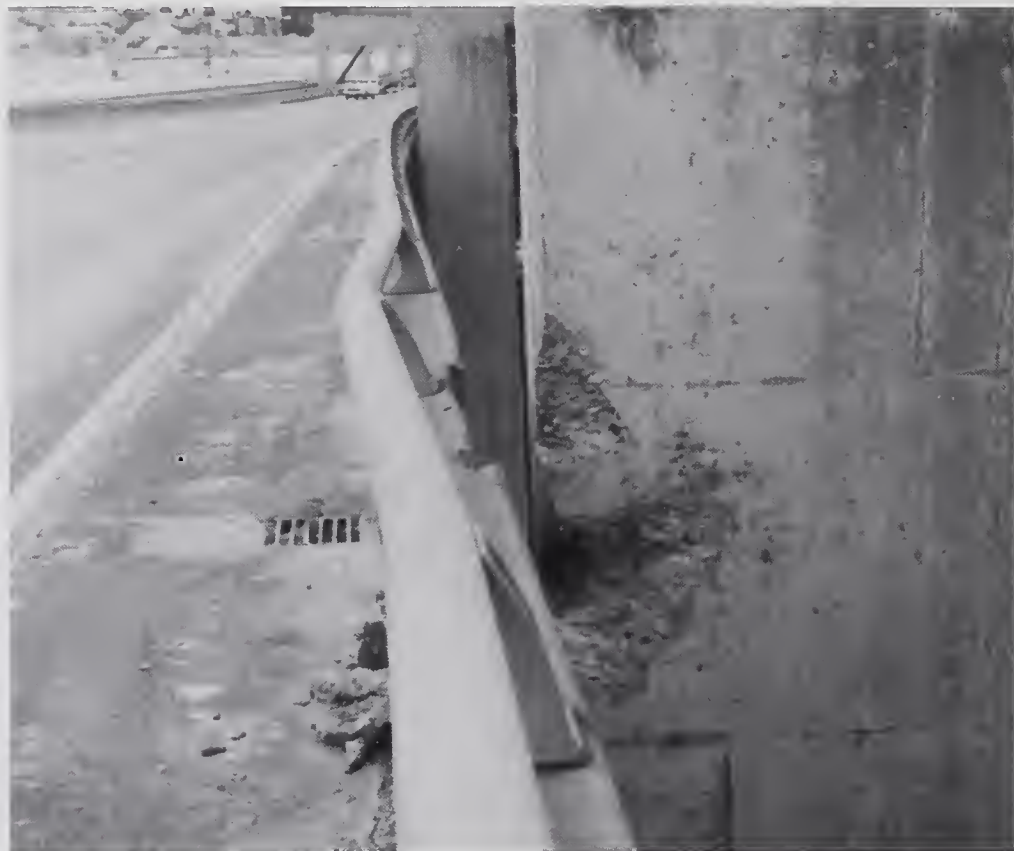
Figure 5.9.10 Pounding damage at I-280 south of Army Street.
