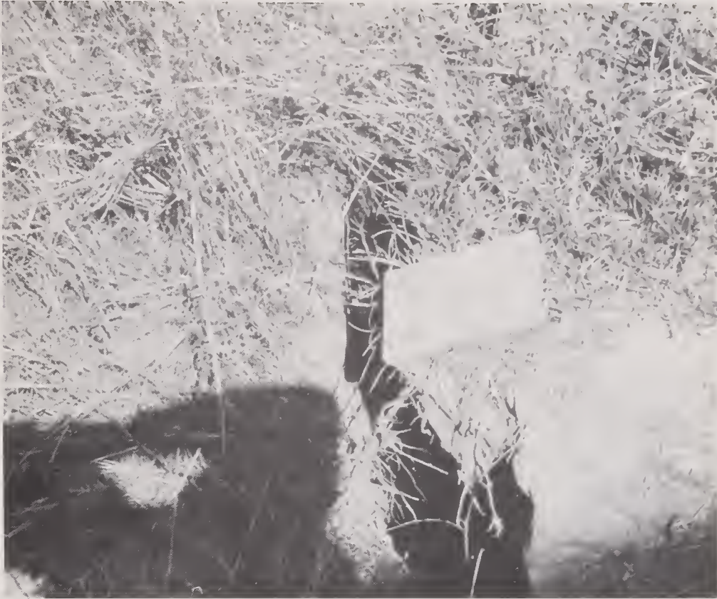
Figure 3.3.8 Tension cracks on Pajaro River bank in Watsonville.
