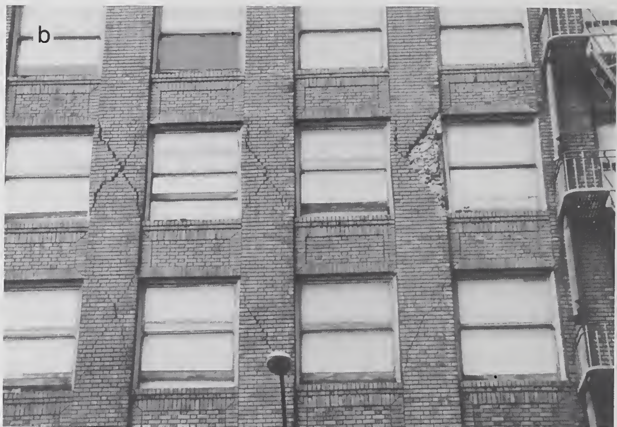
Figure 4.3.2 Dalziel apartment building: (a) overall appearance and (b) close-up view of cracking in masonry piers (location #1).
