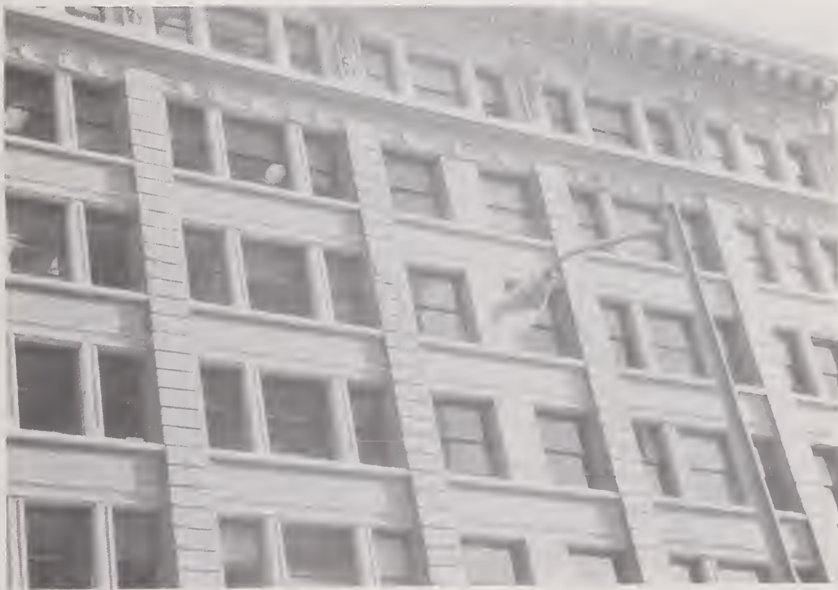
Figure 4.2.32 Example of damage to masonry cladding of Wells Fargo Bank building (location #7).
