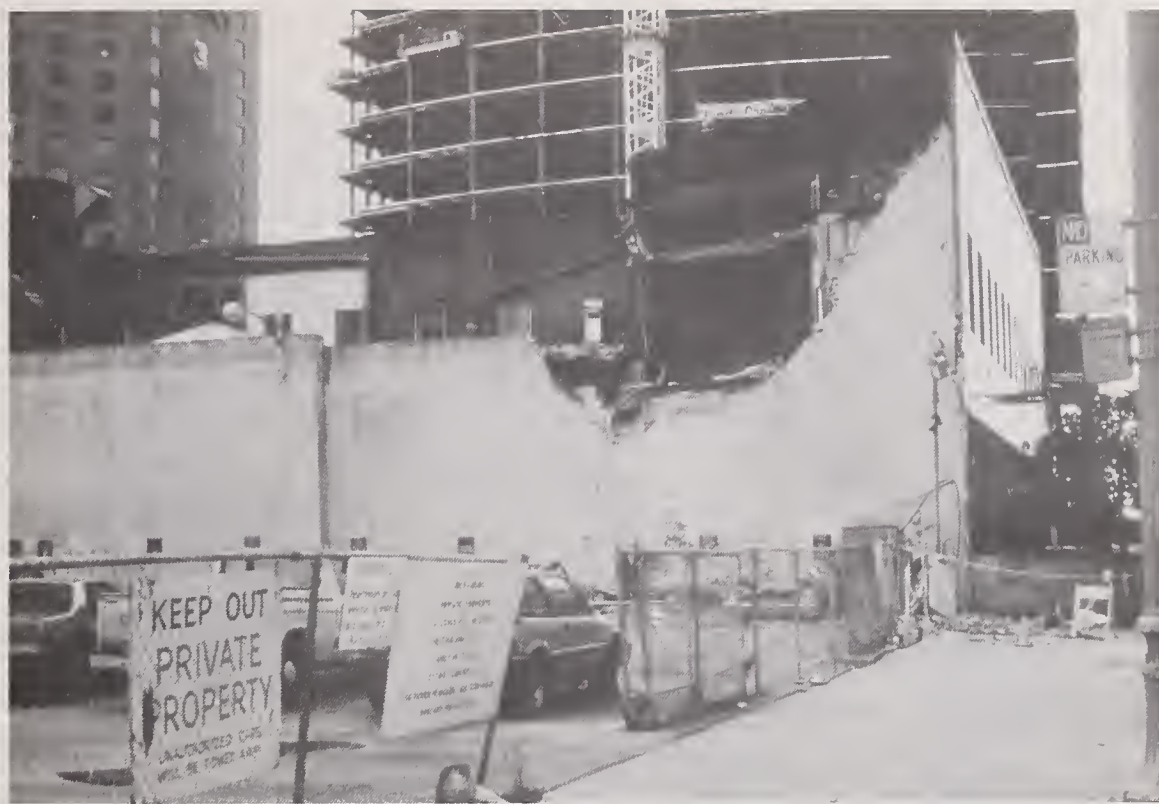
Figure 4.3.6 Collapse of unreinforced masonry wall crushed vehicles in adjacent parking lot (location #5). In background is a steel-framed building under construction which sustained damage.
