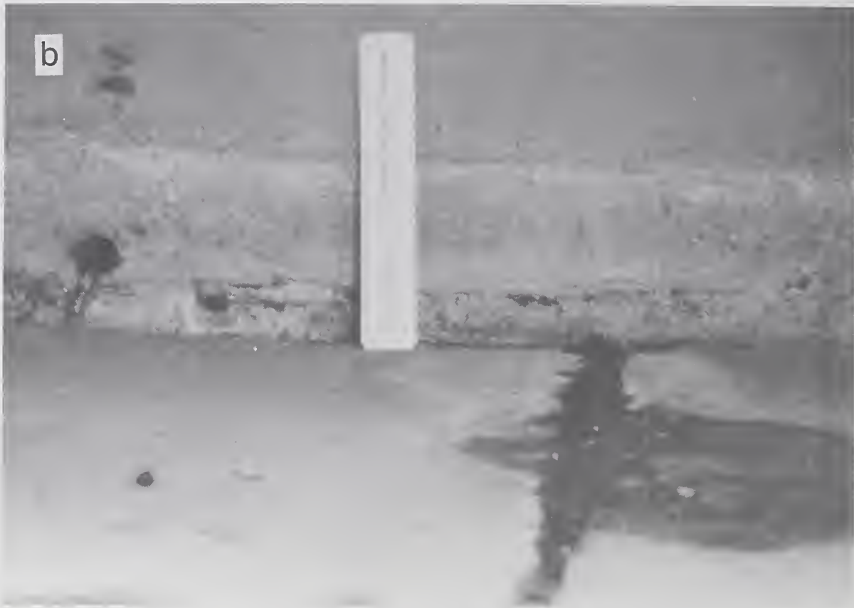
Figure 4.2.26 (a) Sidewalk showing distortions due to differential settlements, and (b) close-up view of intersection of sidewalk with retaining wall showing magnitude of differential movement.
