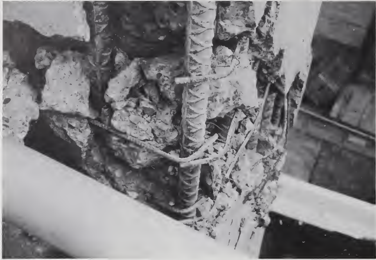
Figure 5.9.9 Close-up view of the failure zone of Bent 51, showing anchorage failure of ties.
