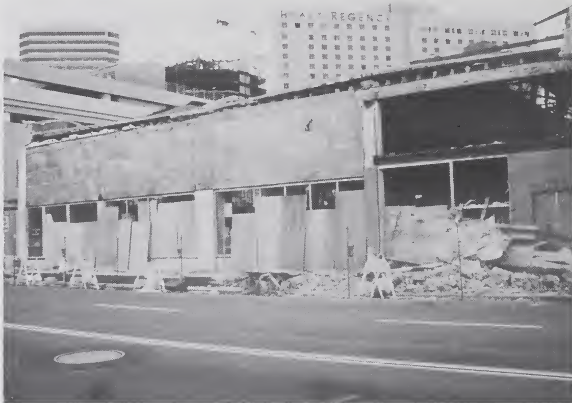
Figure 4.3.5 Extensive damage occurred to a two-story unreinforced masonry building built in 1917 (location #3).
