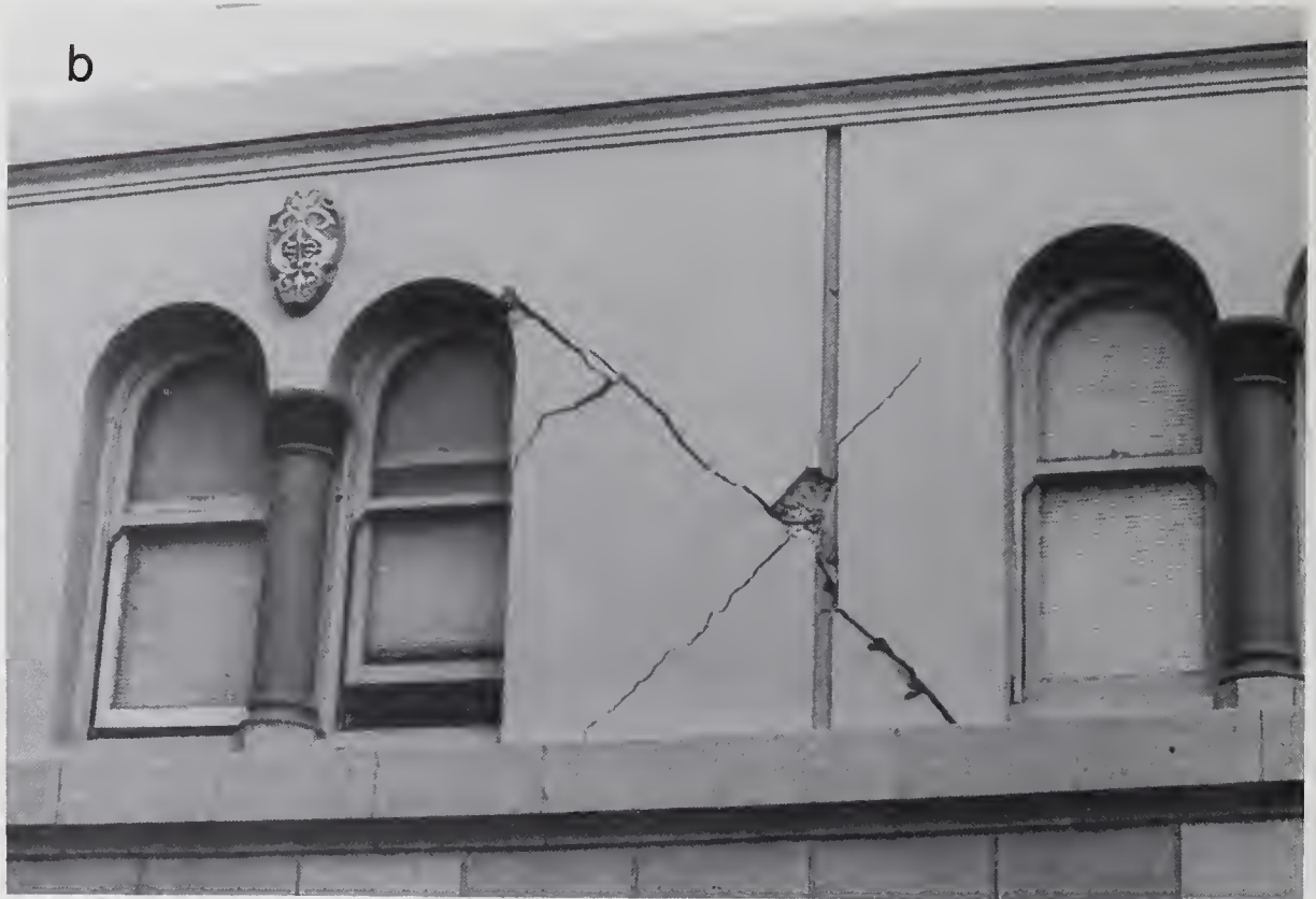
Figure 4.4.11 (a) Seven-story, reinforced concrete building suffered severe cracking; (b) Close-up view of damage to second-story walls.
