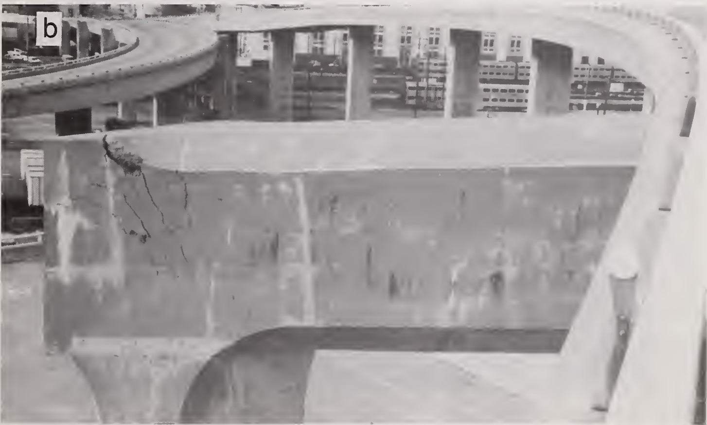
Figure 5.9.14 Damage to girder supporting exit ramp: (a) eastern portion and (b) western portion.
