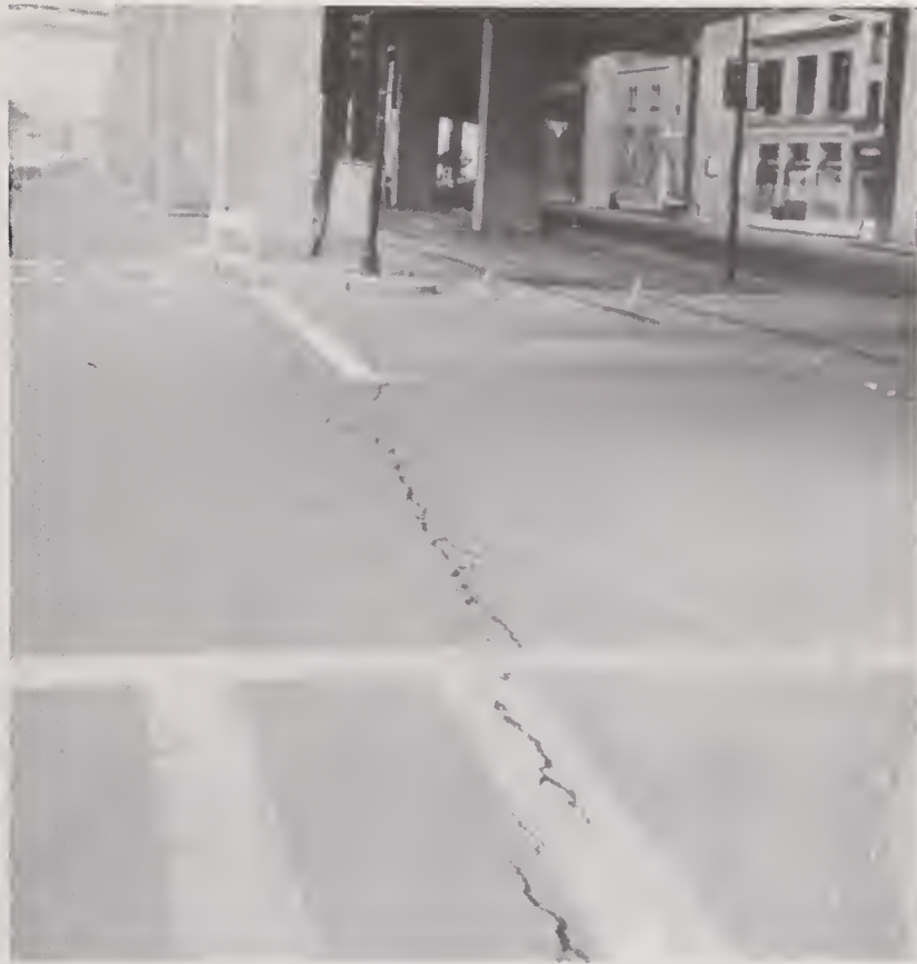
Figure 3.3.5 Tension crack at Mission Street and Embarcadero Freeway.
