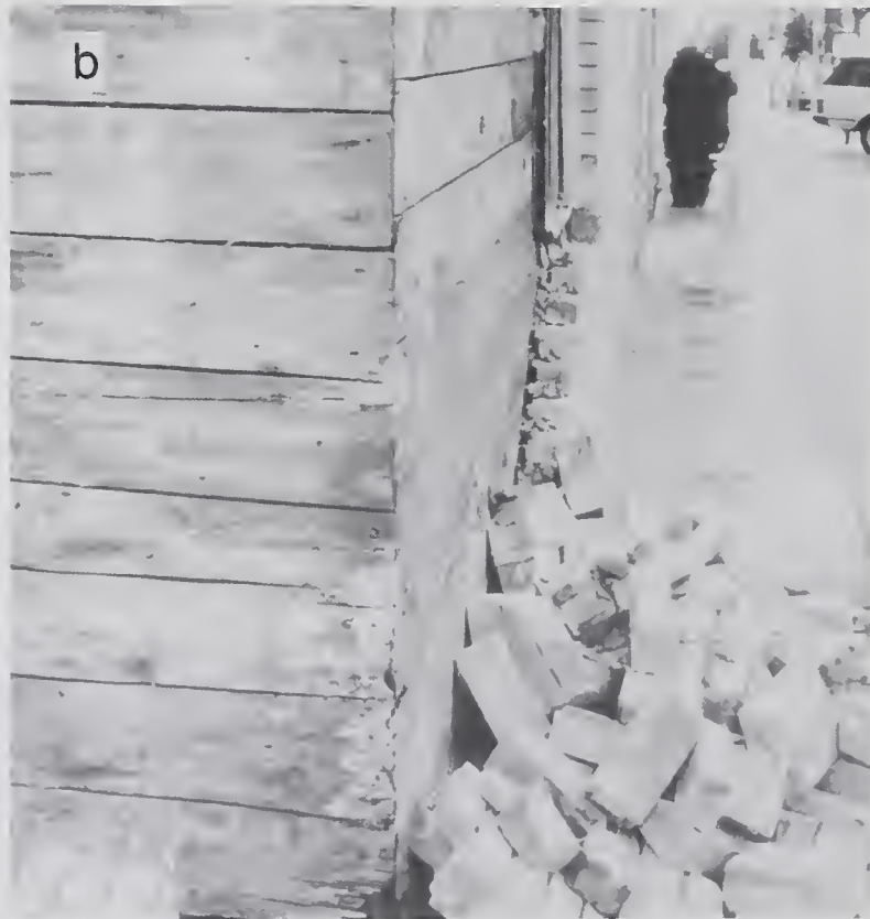
Figure 4.2.19 (a) Example of building with failure of brick masonry facade (location #12) and (b) close-up view of corner showing damaged wood and lack of anchorage to the masonry.
