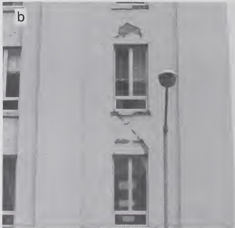
Figure 4.2.33 (a) Reinforced concrete, flat-slab building which sustained severe damage to the exterior walls (location #6); (b) close-up view of damage to spandrels.
