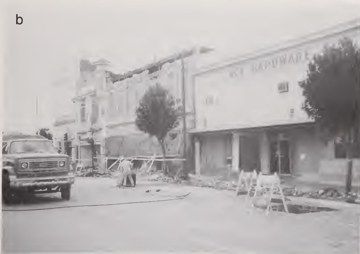
Figure 4.4.4 (a) Failure of wood-framed building with masonry walls and multiple opening in first story (Los Gatos); (b) typical damage to parapets and storefront windows (Watsonville).
