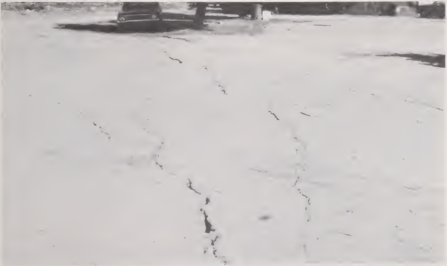
Figure 3.3.9 Tension cracks behind Pajaro River levee.
