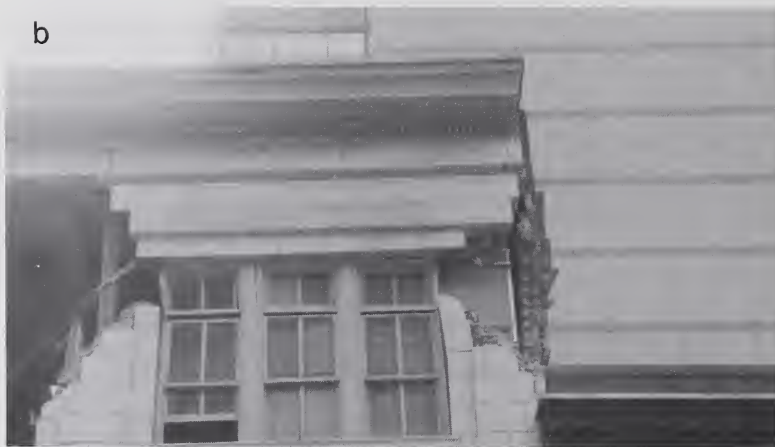
Figure 4.2.28 (a) Damage to the southeastern corner of the Golden State Bank Building; (b) Close-up view of the northeastern corner; damage was likely caused by pounding against the adjacent building.
