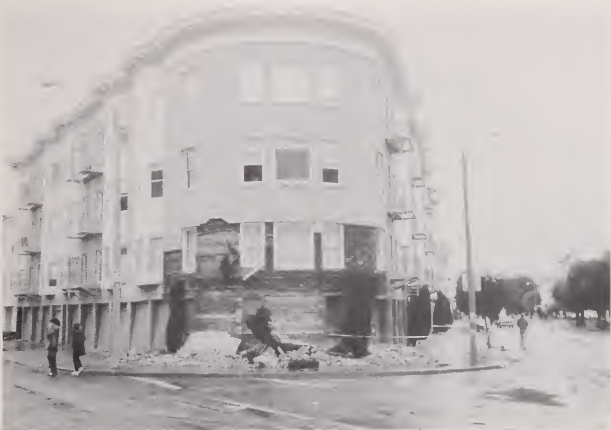
Figure 4.2.17 Example of building with failure of brick masonry facade (location #2).
