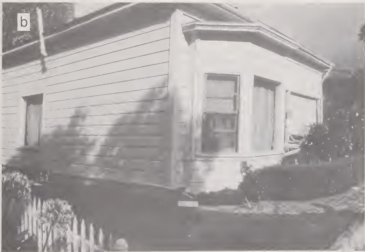
Figure 4.4.2 Examples of failures of houses in Los Gatos: (a) large house suffered large distortion and (b) a small house was rocked off of its foundation.
