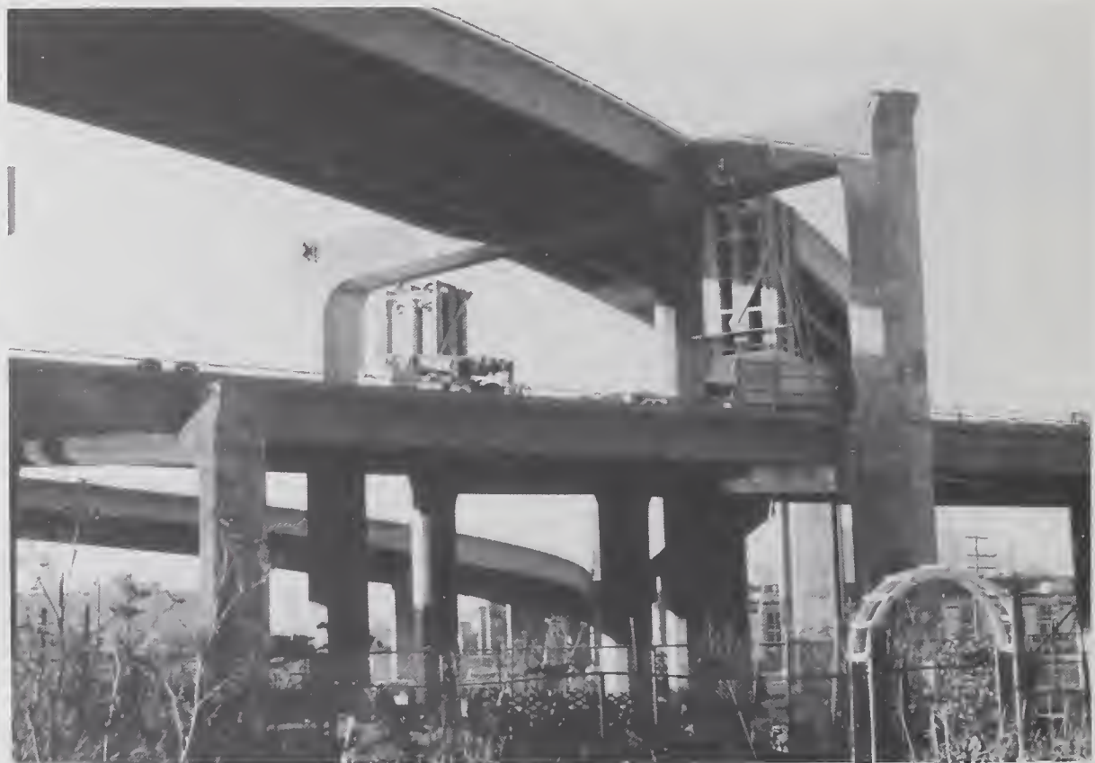
Figure 5.9.13 The Sixth St. exit ramp where it passes over the northbound lanes of I-280. (View is toward west; cribbing was added to provide temporary support.)
