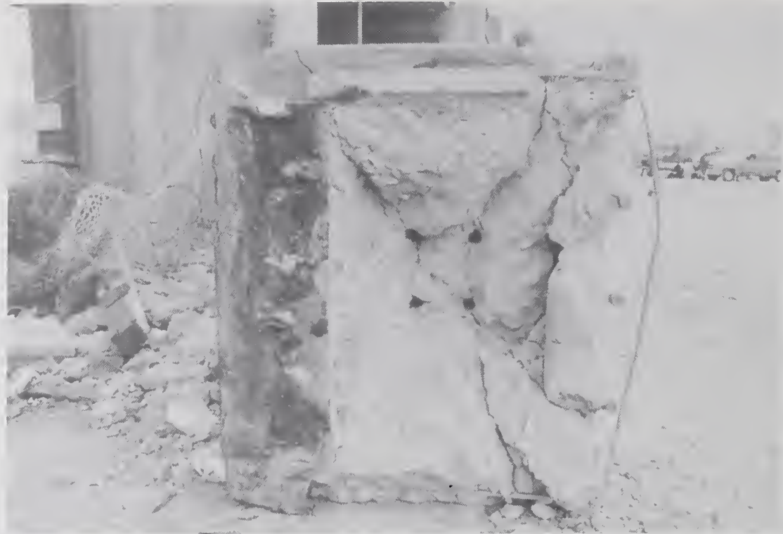
Figure 5.6.34 Detail of the base of the two-hinged column that was ejected from the west side of Bent 72. The 4-#10 dowel bars which passed through the center of the shear key have been pulled free.
