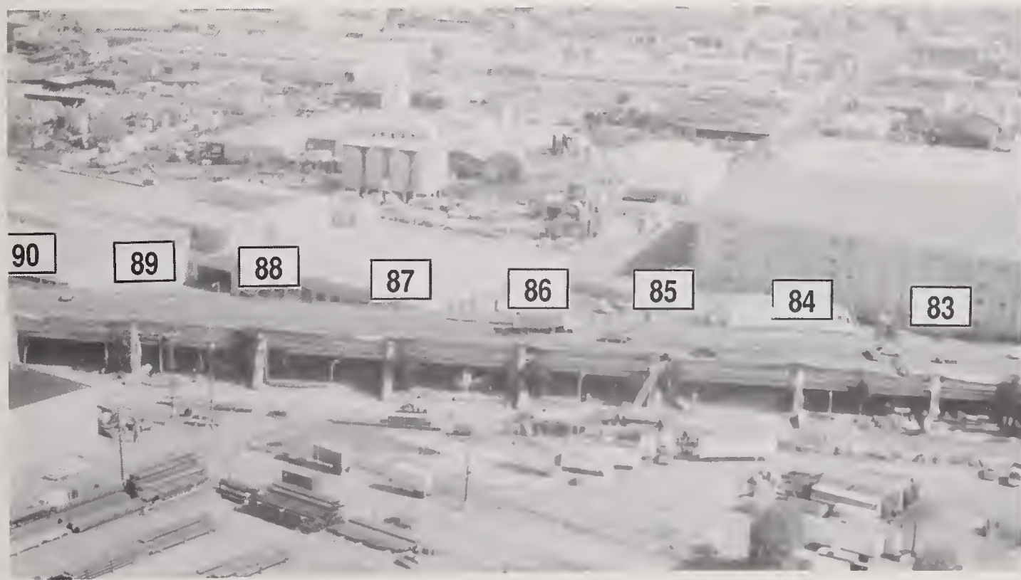
Figure 5.6.17 Aerial photo looking east to the collapsed portion of Cypress Structure between Bents 83-90.
