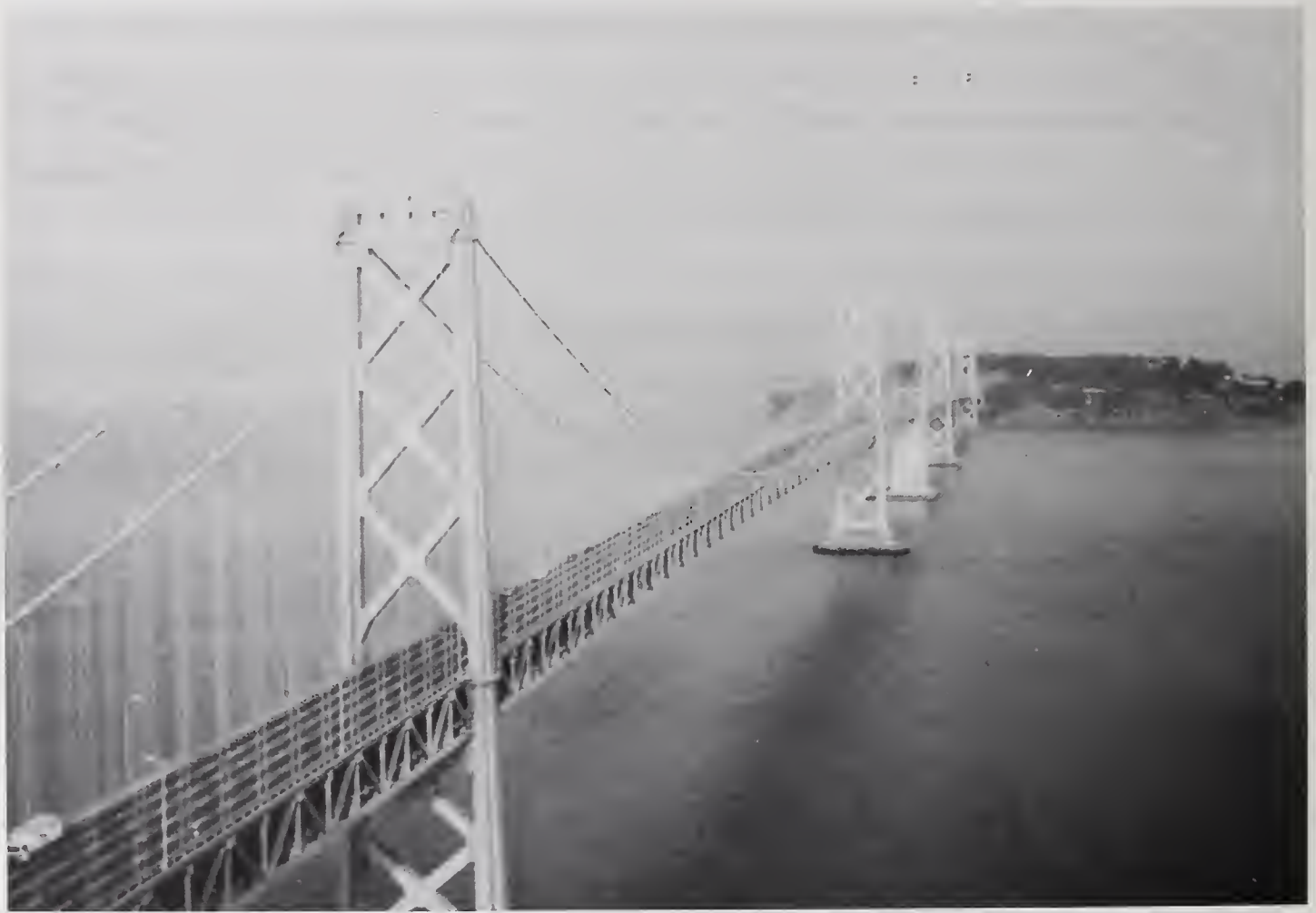
Figure 5.7.1 View looking east from San Francisco to Yerba Buena Island showing the two main suspension spans for the Bay Bridge. No damage was detected in this section.
