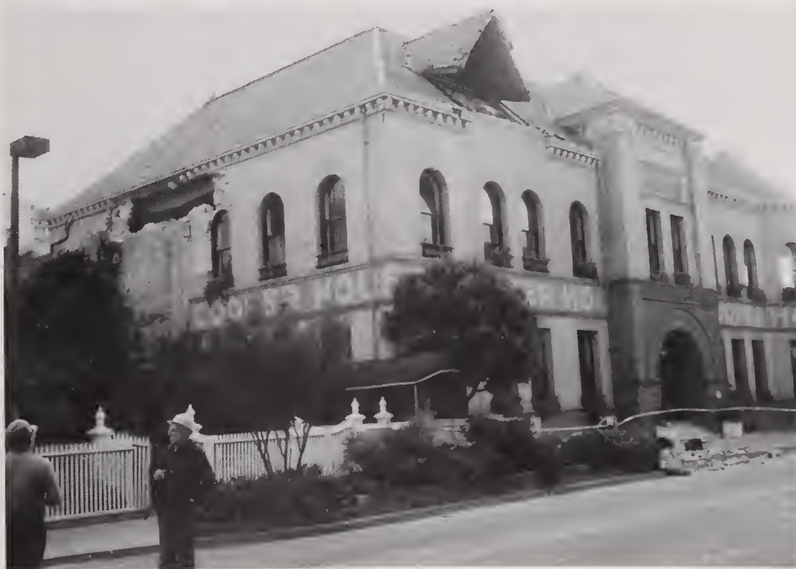
Figure 4.4.10 Historic Cooper House in Santa Cruz was severely damaged and had to be demolished (location #2).
