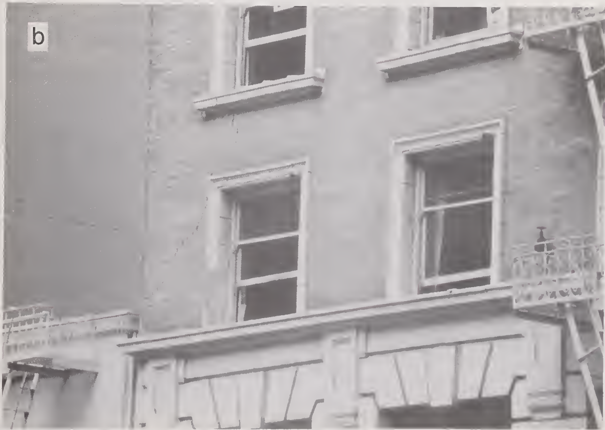
Figure 4.2.27 (a) Severely damaged Marine Building at corner of Front St. and California St.; (b) Close-up view of the northwest corner showing severity of cracking.
