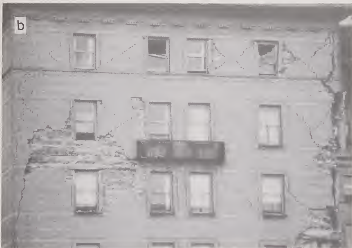
Figure 4.3.3 Oakland Hotel: (a) View of west wing and (b) close-up view of damaged masonry infill (location #6).
