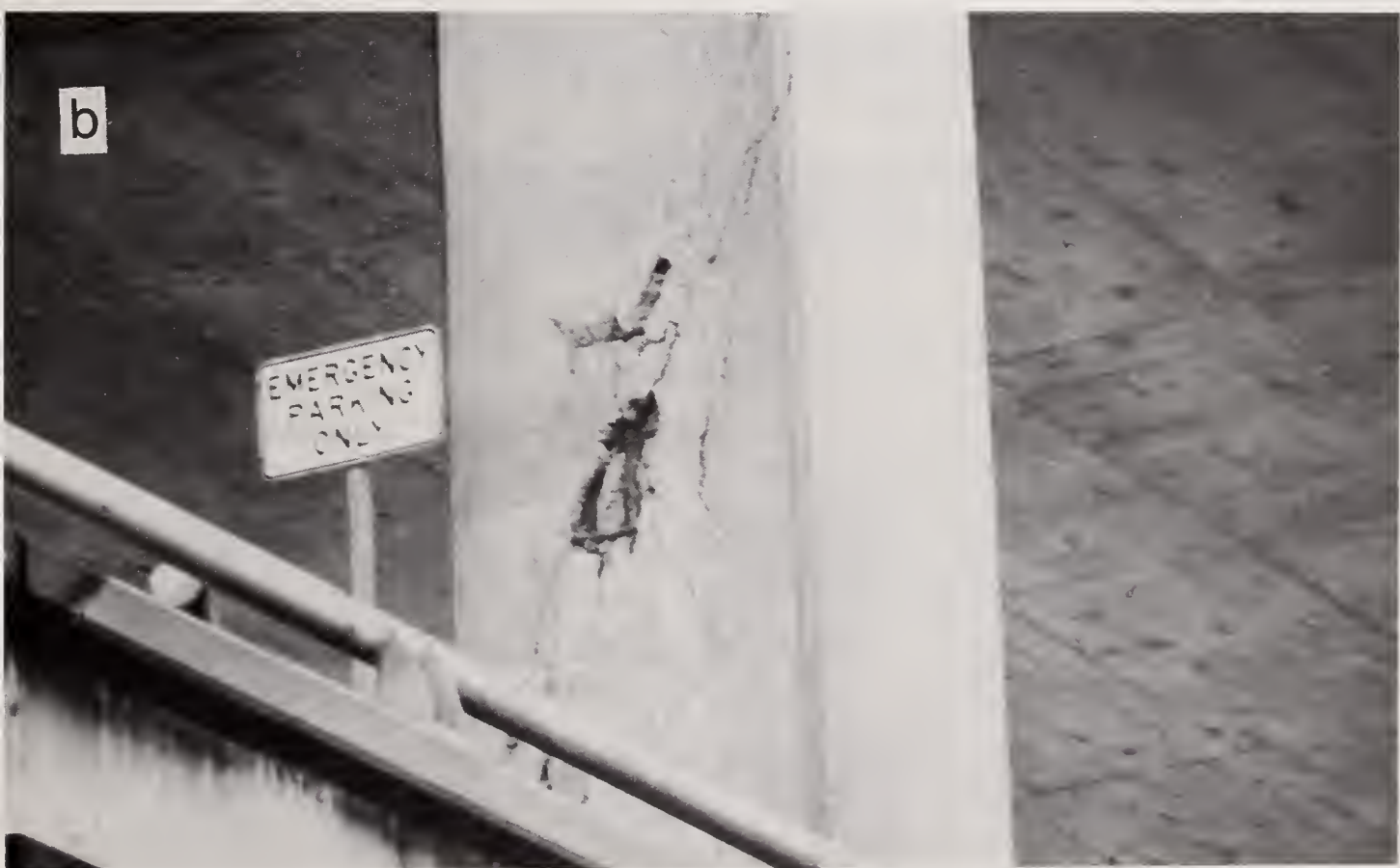
Figure 5.11.3 Close-up views of east side columns of (a) Bent 42 and (b) Bent 43.
