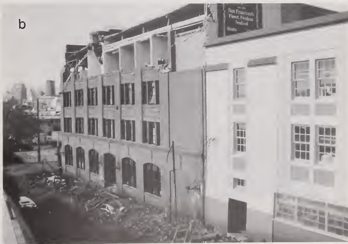
Figure 4.2.34 (a) Damage to upper story of unreinforced masonry building on Bluxome St. (location #8); (b) damage to the southwestern wall which resulted in the death of six persons.
