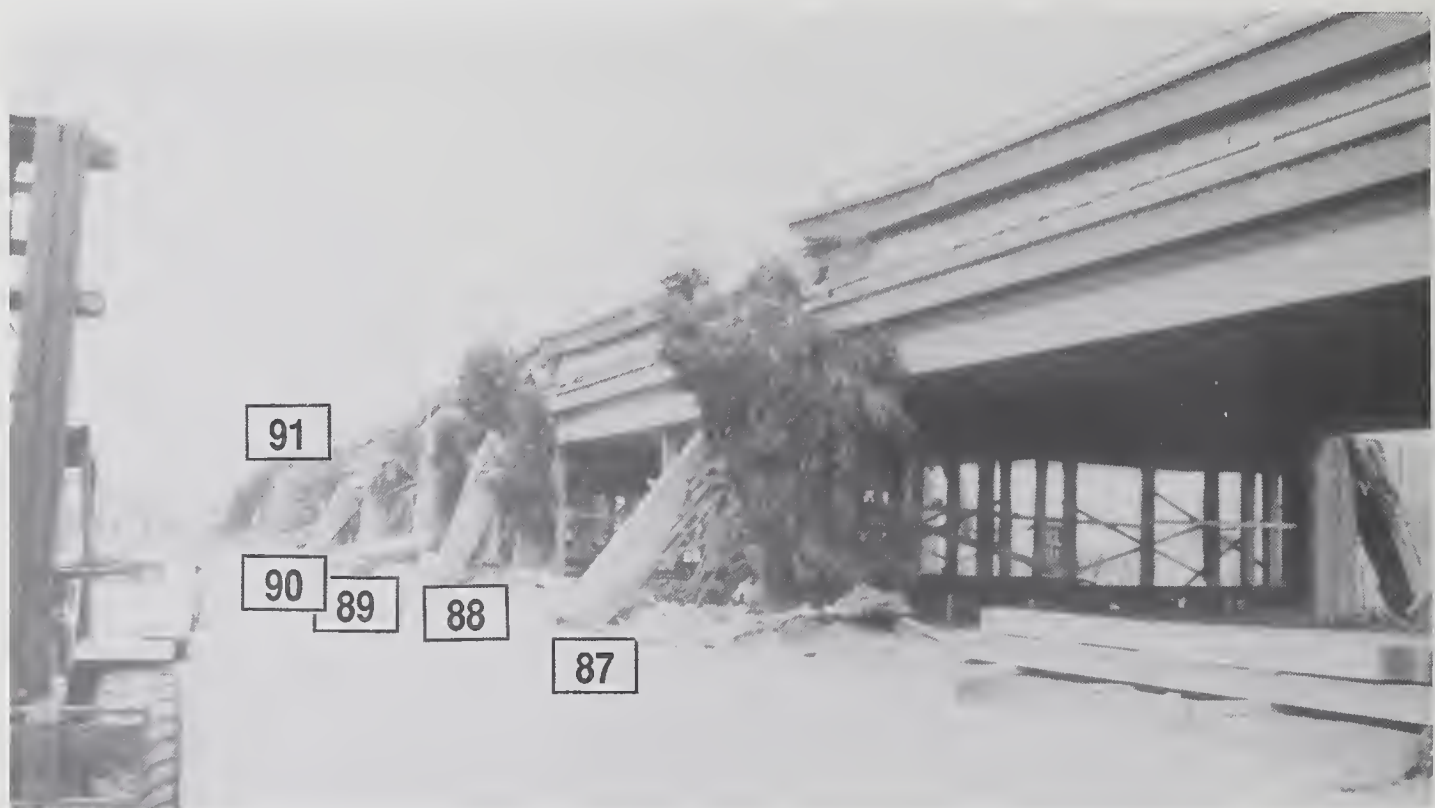
Figure 5.6.23 View of the west side of Cypress Structure looking north between Bents 86-92. These were all Type 1 bents which demonstrate the uniformity of the collapse mechanism.
