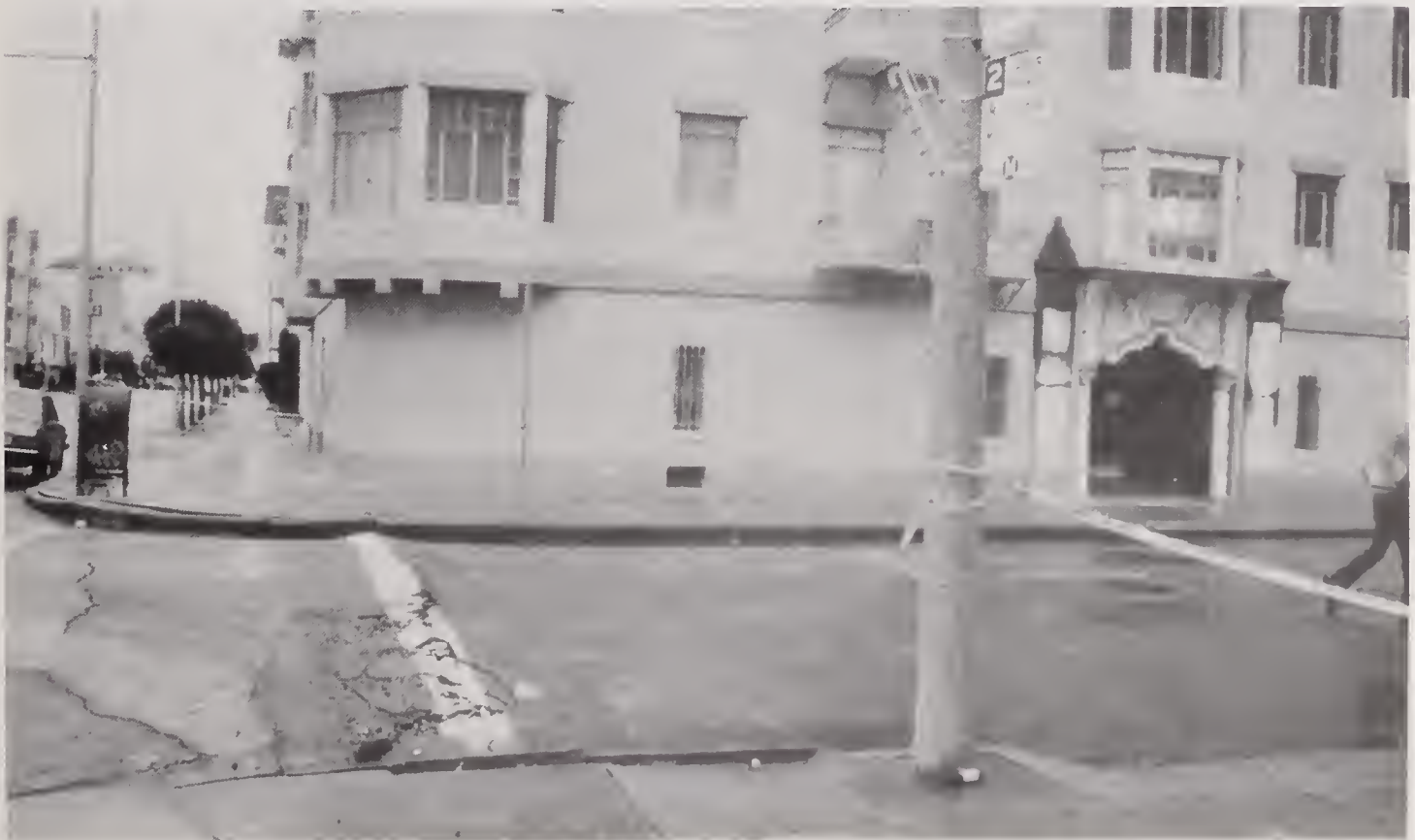
Figure 3.3.6 Pavement heave over utility pipe.
