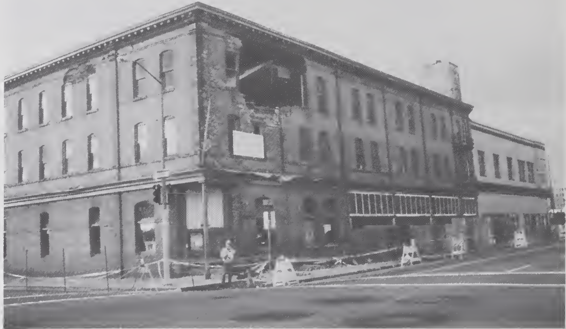
Figure 4.3.4 Damage to the Clay Building, an unreinforced masonry structure (location #2).
