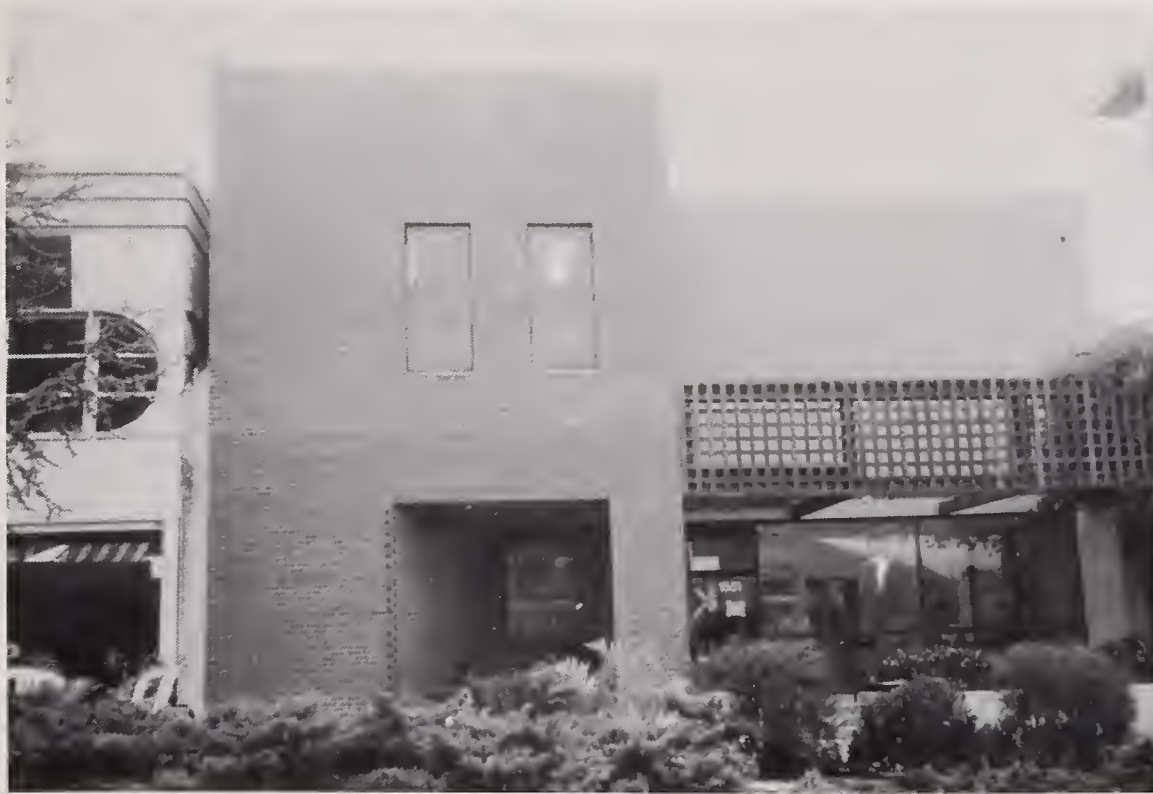
Figure 4.4.9 Modern reinforced masonry structure which was undamaged; building on the left suffered roof failure causing two deaths (location #1).
