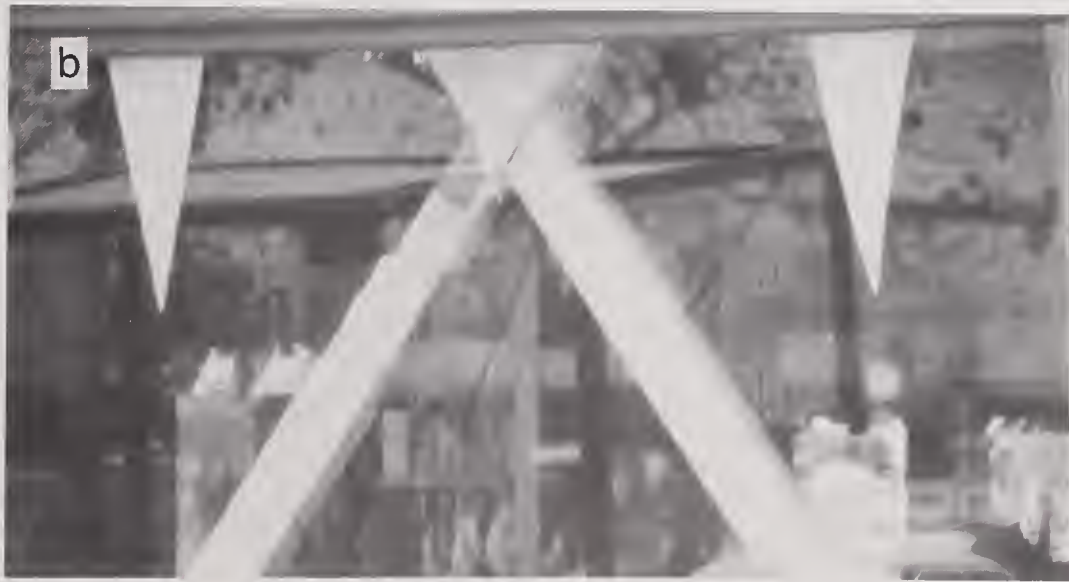
Figure 4.2.29 (a) The historic DeBernardi warehouse building showing the bracing added during seismic retrofitting; (b) close-up view of the bracing showing damage caused by earthquake.
