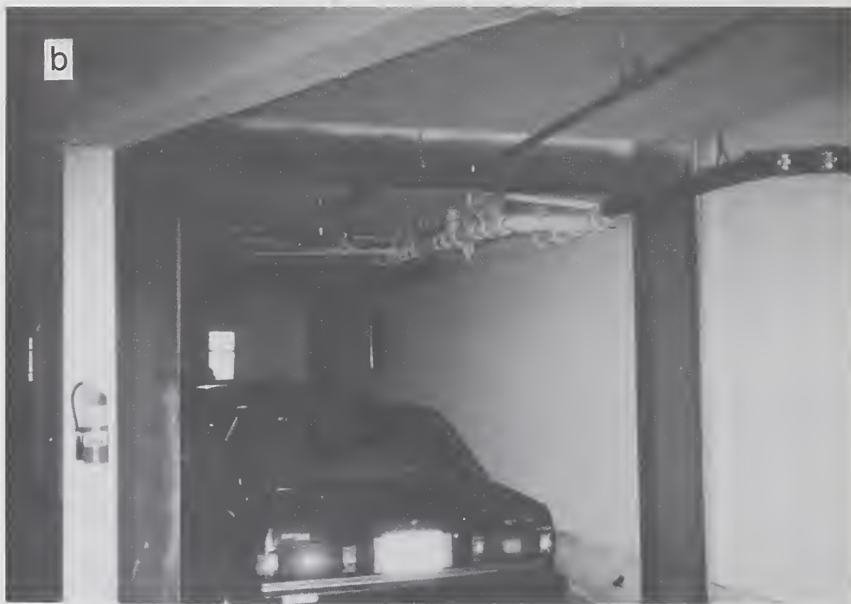
Figure 4.2.22 (a) An undamaged, three-story building (location #8) and (b) view of the moment-resting frame used for retrofitting.
