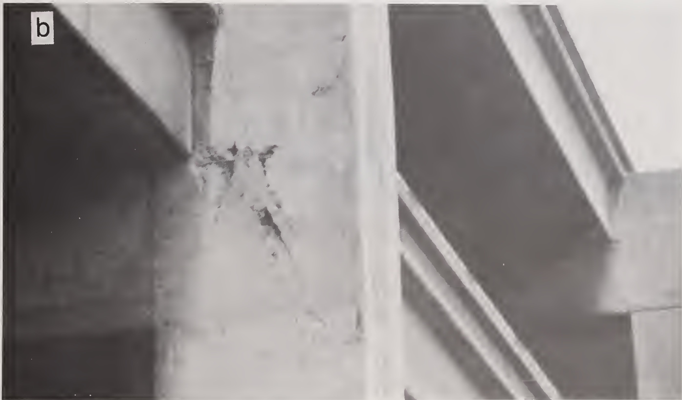
Figure 5.10.5 (a) Close-up view of west side of Bent 78 showing diagonal cracking in joint and vertical cracking at girder-column boundary; (b) close-up view of east side of Bent 79 showing diagonal cracking in joint.
