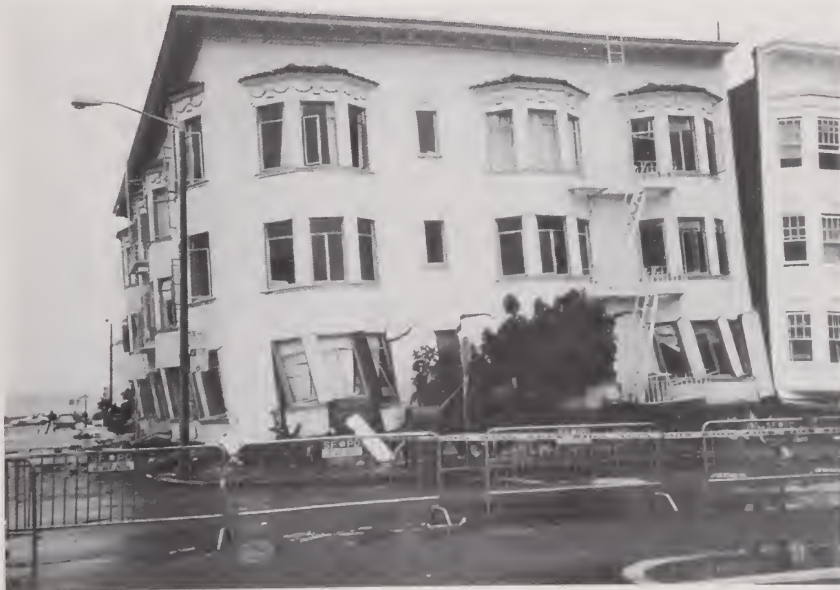
Figure 4.2.7 Two four-story buildings which suffered total collapse of their first stories (location #14).
