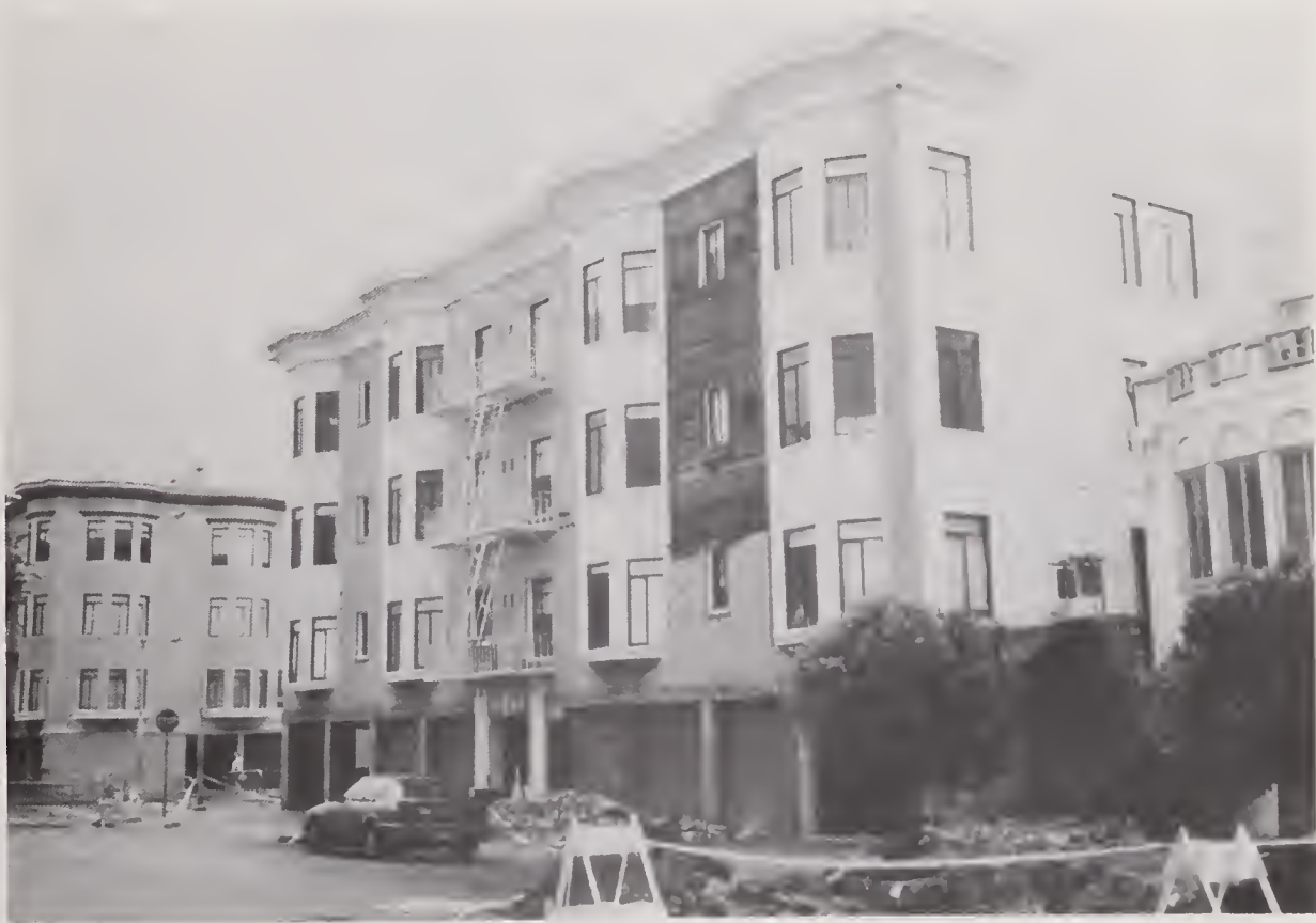
Figure 4.2.18 Example of building with failure of brick masonry facade (location #10).
