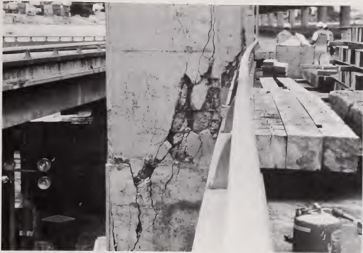
Figure 5.9.7 Diagonal cracking of the east-side column of Bent 52 (north face).
