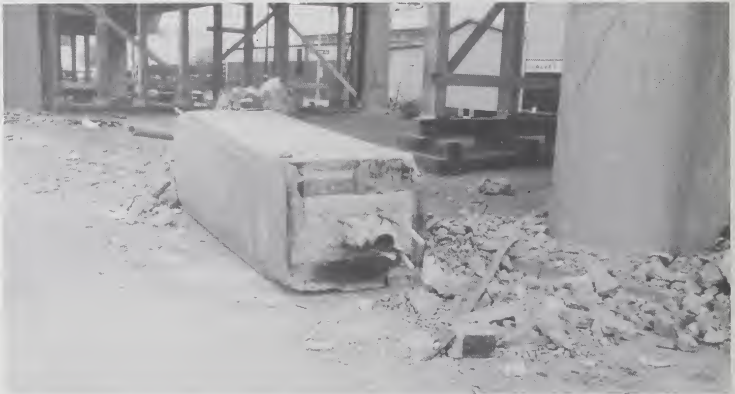
Figure 5.6.35 Detail of the bottom of the two-hinged column that was ejected from the west side of Bent 71 showing central pipe used to drain the upper road deck and the 4-#10 dowel bars used to transfer shear across the hinge.
