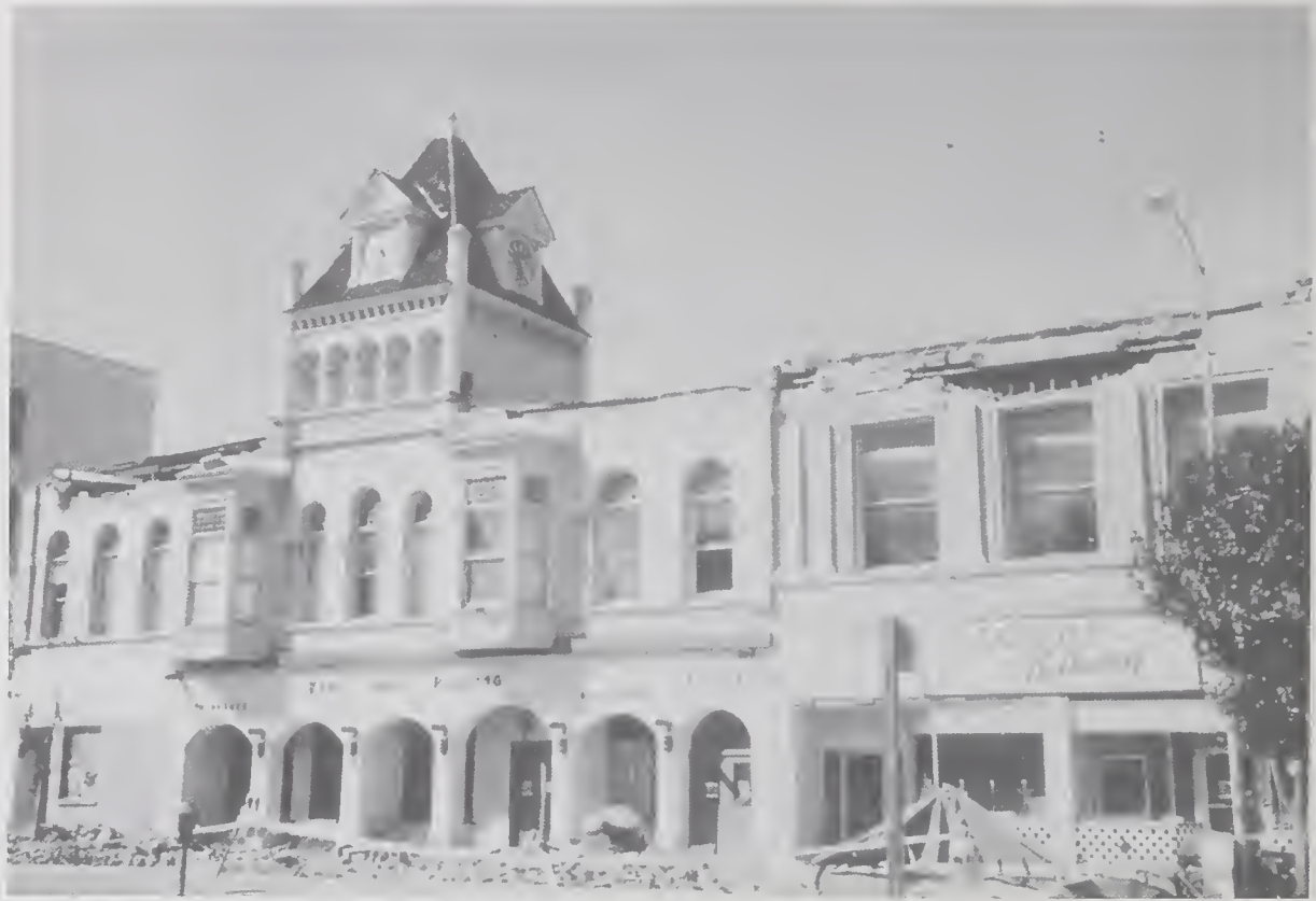
Figure 4.4.5 Falling brick from this old masonry building in Watsonville caused one death.
