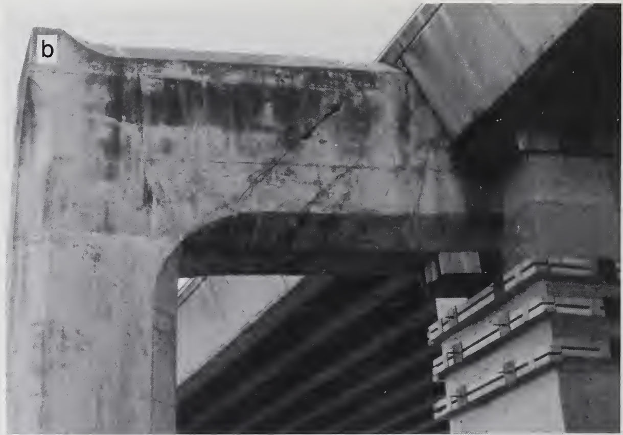
Figure 5.9.15 (a) Bent 32 supporting I-280 at Sixth St. exit ramp and (b) close-up of girder showing diagonal cracking.
