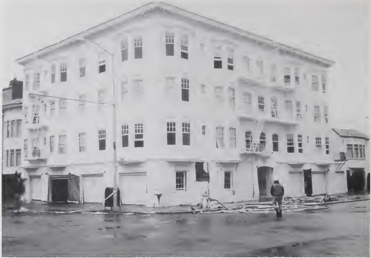
Figure 4.2.12 Example of four-story building with multiple garages in the first story (location #6).
