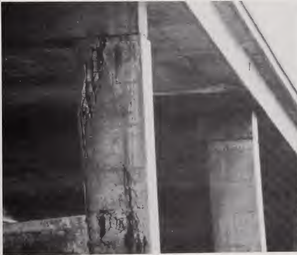
Figure 5.9.4 Damage to west-side column of Bent 48 (looking toward south).
