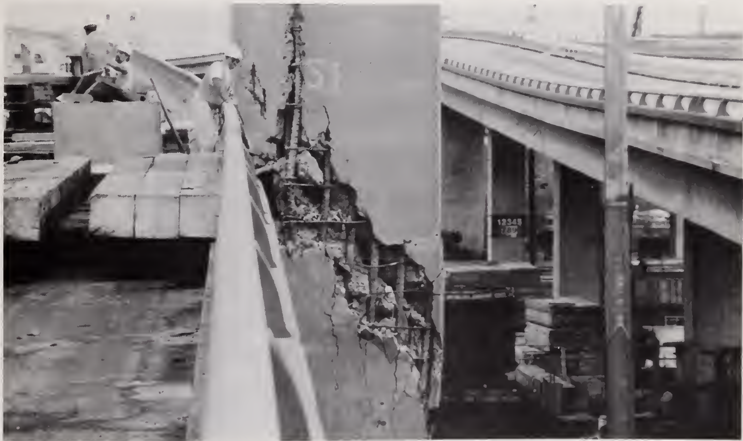
Figure 5.9.8 Diagonal cracking of the east-side column of Bent 51 (south face).
