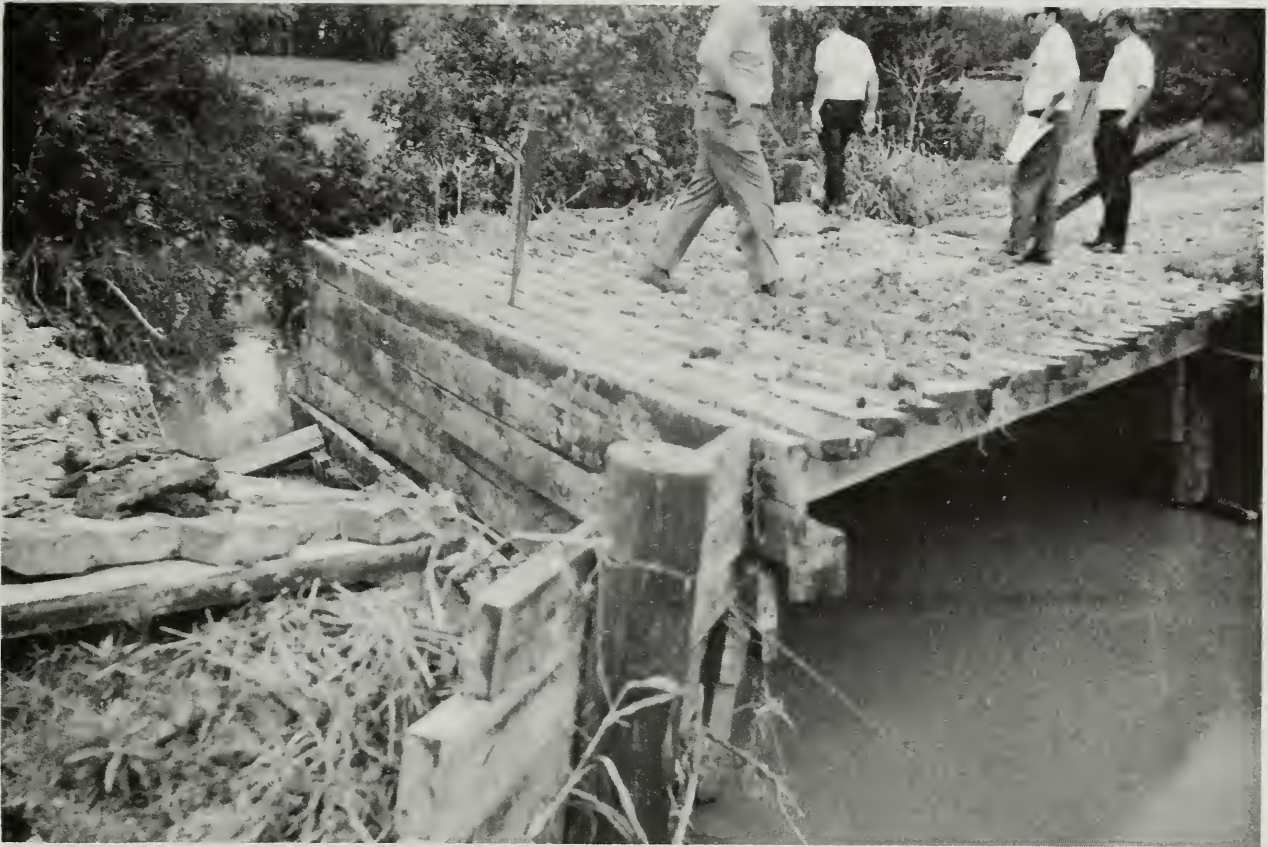
Floodwater damage to county road bridge on Pecan Creek tributary following heavy spring rain of May 9, 1971.
