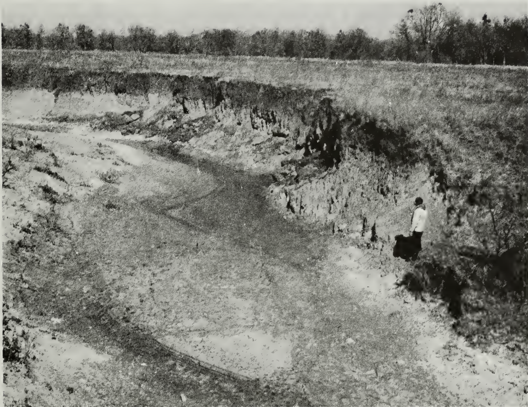
New channel formed by nature in the flood plain of North Elm Creek. The abandoned tree-lined and sediment filled original channel is located in the background. Notice nature does not use spoil banks. The material moved from this section was transported downstream as sediment.
