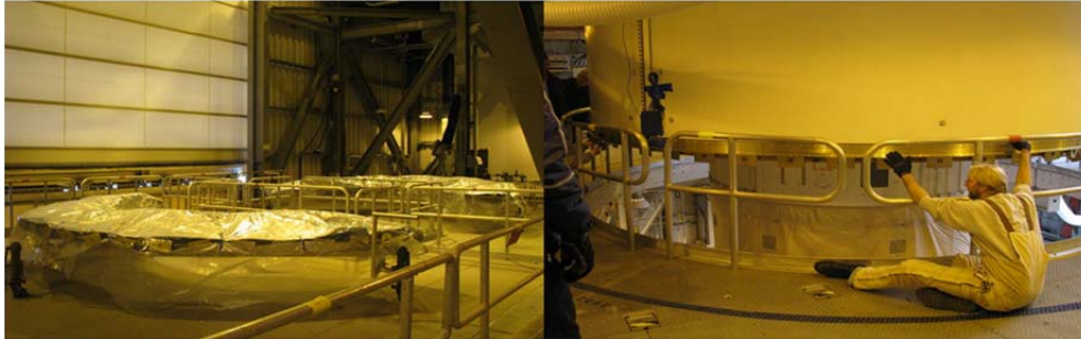
Figure 29. Centaur Forward Load Reactor and Base Module
