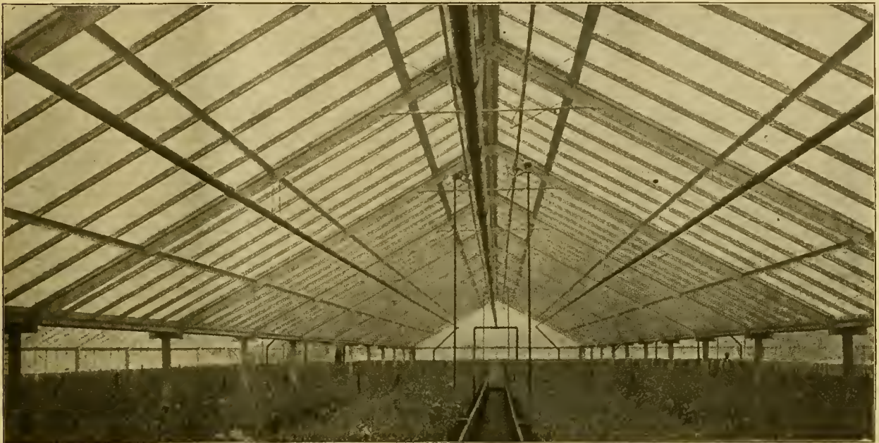
THE ABOVE ILLUSTRATES OUR IRON CONSTRUCTION WITH IRON GUTTER, MADE IN LENGTHS UP TO 25 FEET. FROM A PHOTOGRAPH OF THE CRESSBROOK GREENHOUSES, FALL RIVER, MASS.
