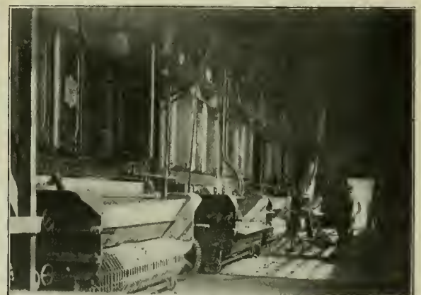
View in Boiler Room, Showing Boiler Fronts, Chain-Grate Stokers, and Coal Chute to Stoker Hopper from Pockets Above.
