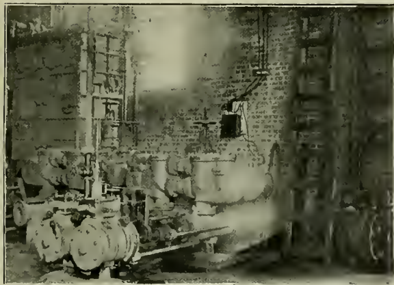
Feed-Water Heater and Purifier, and Boiler Feed Pumps, Bucket Coal and Ashes Conveyor to the Right.
