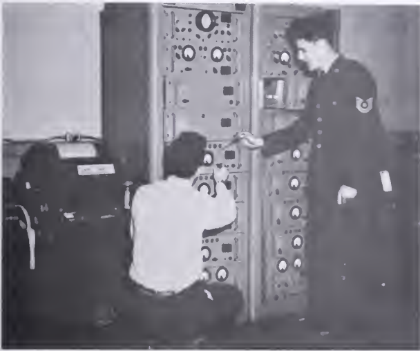
Instructor Ray Angerer and Technical Sergeant Henry W. Case discuss the AN/FGC-5 multiplex terminal equipment.
