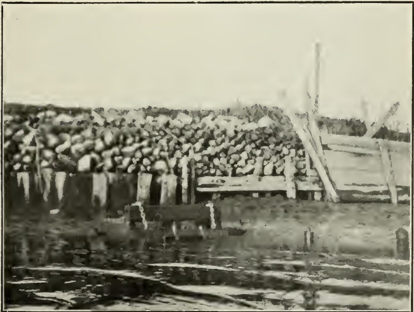
FIG. 2.—METHODS OF LEVEE PROTECTION AND SLUICE 4 AT LOW TIDE IN MAURICE RIVER, DORCHESTER, N. J., NOVEMBER 12, 1909.
