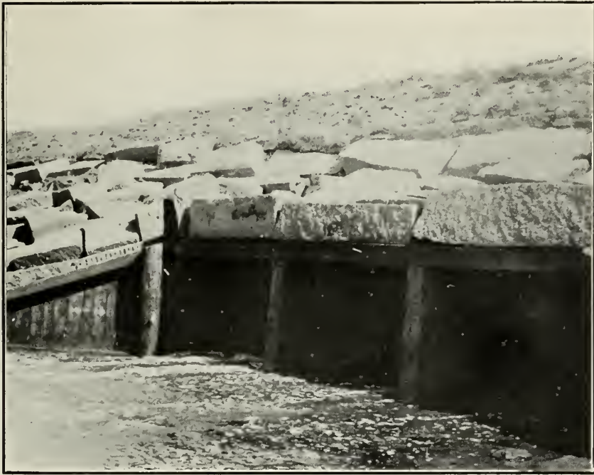
FIG. 1.—OUTER END OF SLUICE AT LOW TIDE, SHOWING GRANITE QUARRY GROUT FACING.
