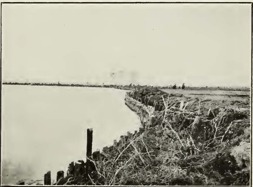
FIG. 2.—LEVEE AND PILE AND BRUSH PROTECTION, MAURICE RIVER, NOVEMBER 2, 1909. MARSH LANDS OF HOWARD COMPTON, DORCHESTER, N. J.
