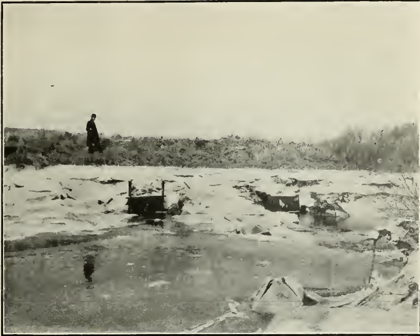
FIG. 1.—SLUICES 8 AND 9, SHOWING FORMATION OF ICE BELOW ORDINARY HIGH WATER MARK.
