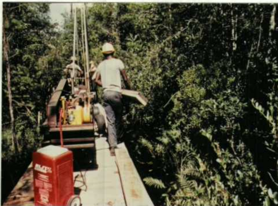
YCC enrollees played a major role in the construction of the Ridley's Little Island Trail boardwalk. 83-1-DLF (08/83)
