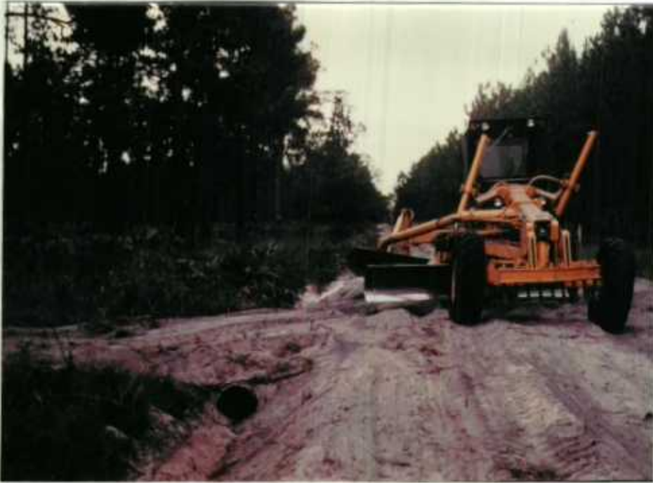
Maintenance of forest compartment roads was necessary for access for wildlife and fire management activities. 83-14-UNK (12/78)
