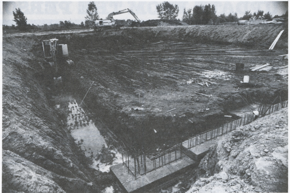
Near the Ross Memorial Building, excavation for NTID's new academic building proceeds.
