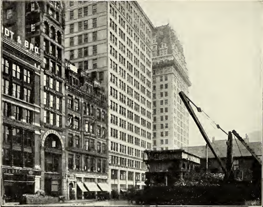
The old home. In the foreground are evidences of the Broadway subway excavation.
