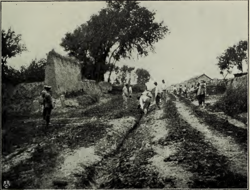
Troops making surface drain in village street, Tang-hsiang-kung-tai. The unit medical officer and a company officer are superintending the work.
