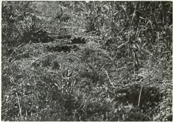
Fig. 62. Perforations due to muskrat burrows in dike about spring used for irrigation; Fall River Valley, Shasta County, California.
