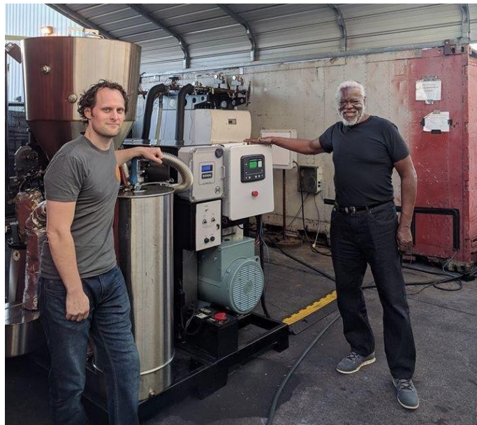
Figure 31: Combined Cooling, Heating, and Power Power Pallet Open House June 2018
