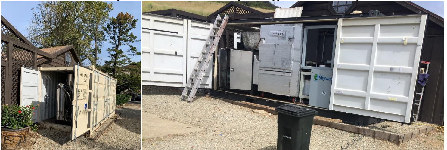
Figure 22: Containerized Combined Cooling, Heating, and Power Power-Pallet at the Skysource Ranch in Malibu (Prototype PP30 in-Field)
