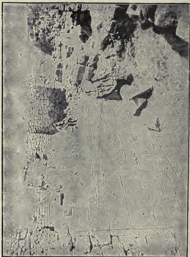
FIG. 29. WALLS OF VI E The retaining wall of the building VI E is seen at a and b , the rear wall at d .
