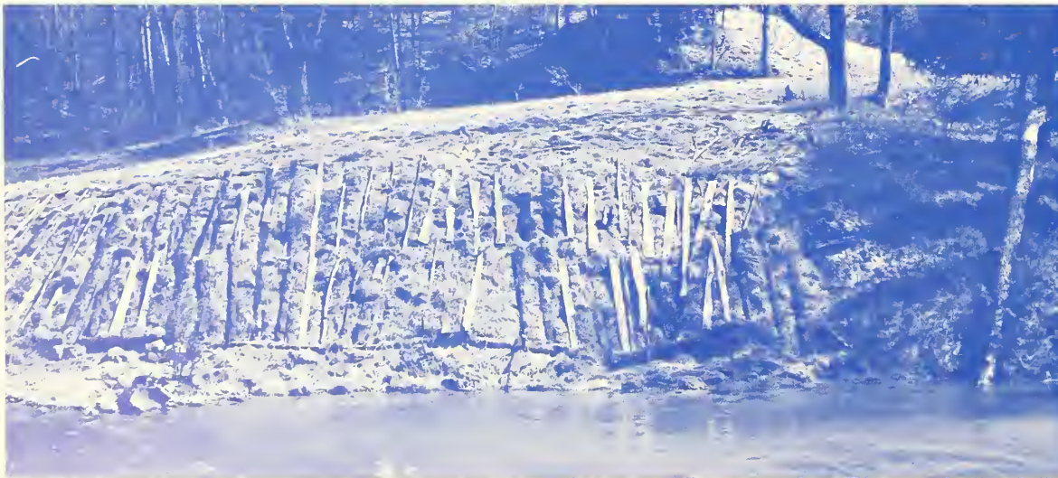
Completion of a streambank stabilization job with mulch and poles in place to stabilize the bank until vegetation covers the site.
