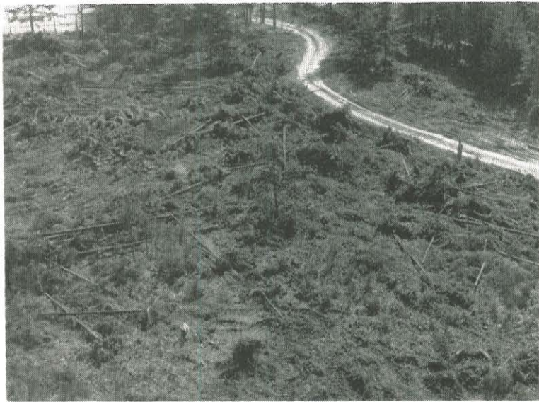
Trees fell to the ground to clear the path for the new Dependent Hospital Unit which is arising at the north of the hospital compound. Shown above is the clearing from which will arise the new unit which will benefit Navy personnel's dependents in this area.
