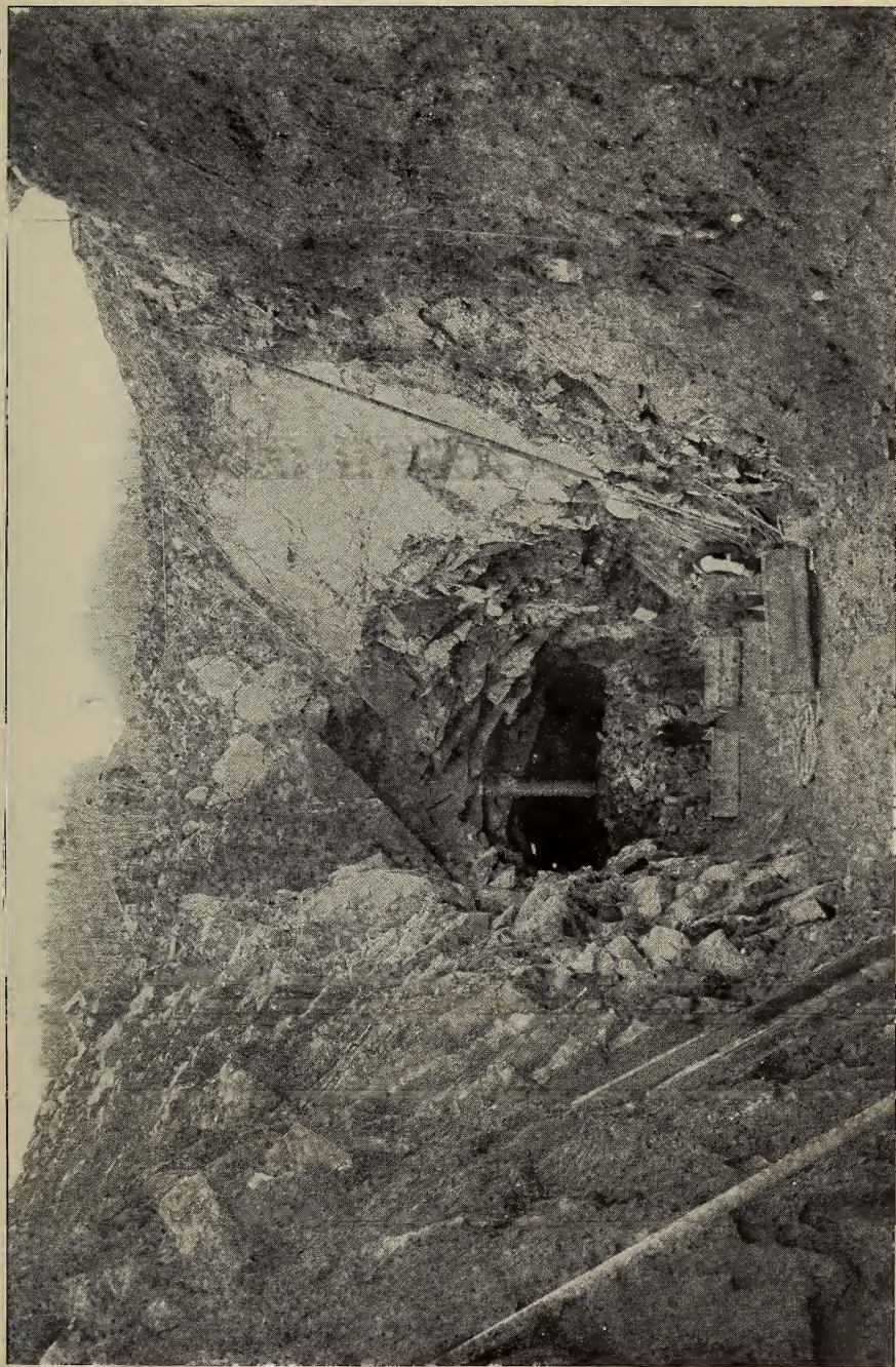
South portal to Garrison tunnel on the Peekskill division. The rock is a badly jointed granite belonging to one of the intrusives of the older gneisses. (Photograph by Board of Water Supply)
