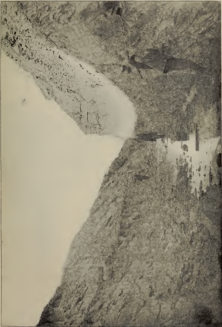
A trench through Hudson River slates and sandstones for cut-and-cover aqueduct construction on the Newburgh division. (Photograph by Board of Water Supply)
